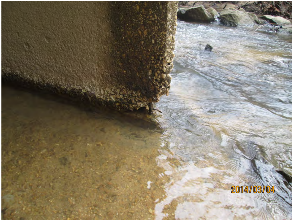
Damage on Downstream Center Barrel
