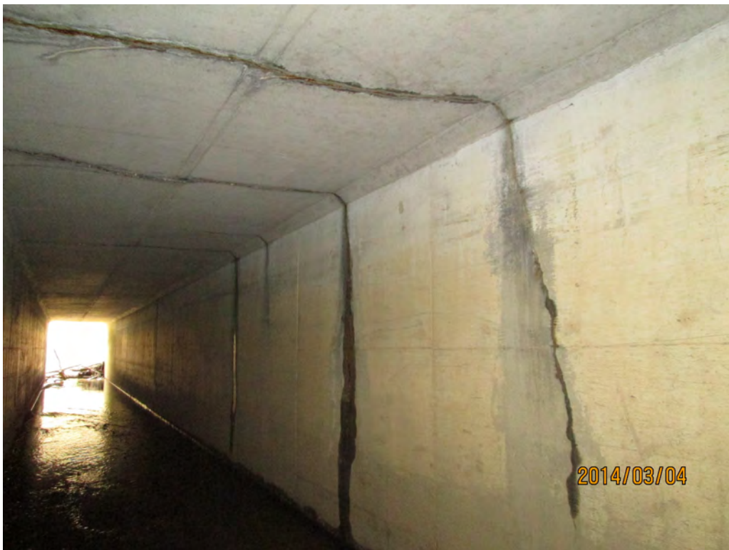
Cracks in Left Barrel
