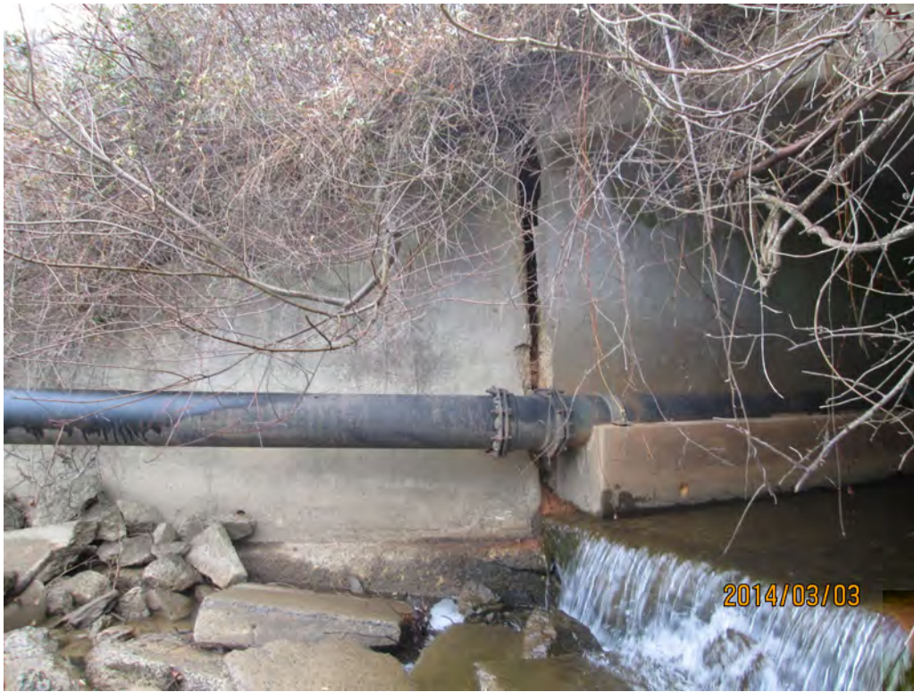
Right Headwall Separation on the Downstream Side
