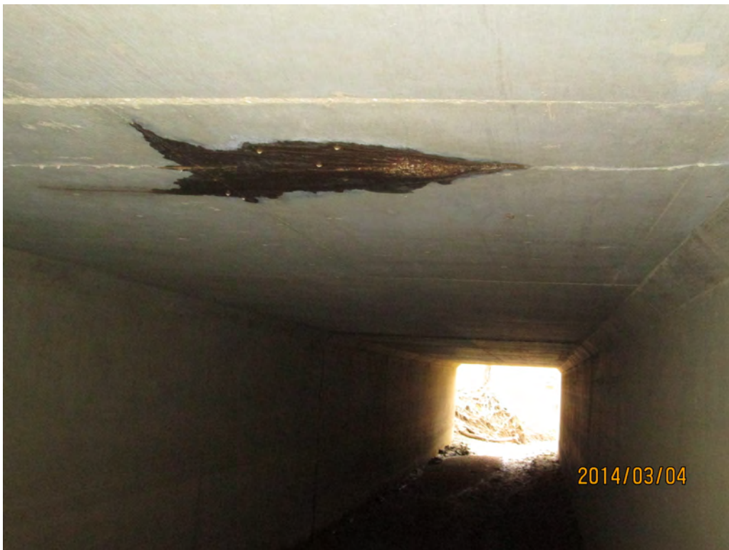
Crack in the Top Slab of Left Barrel
