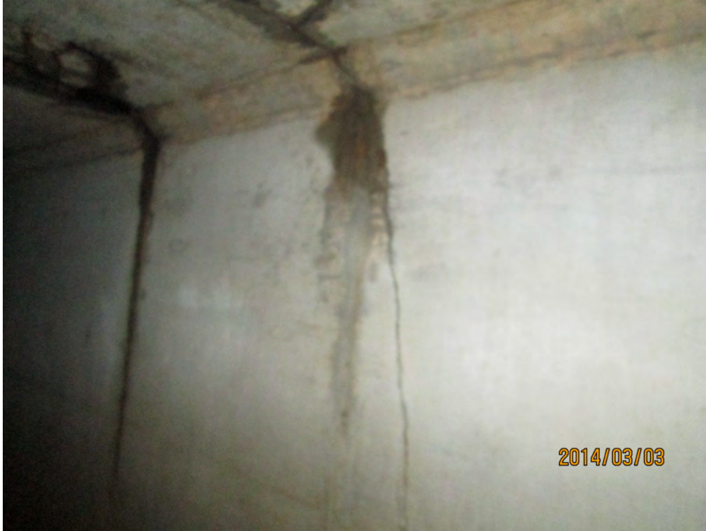
Cracks in the Box
