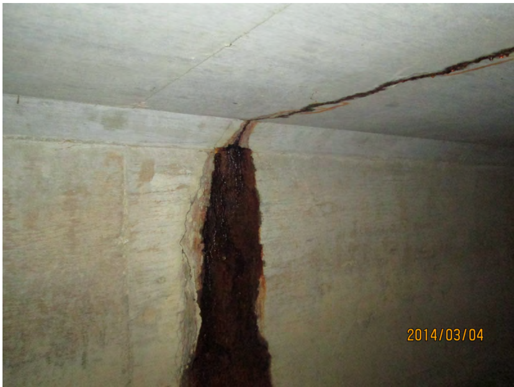
Crack in Right Barrel
