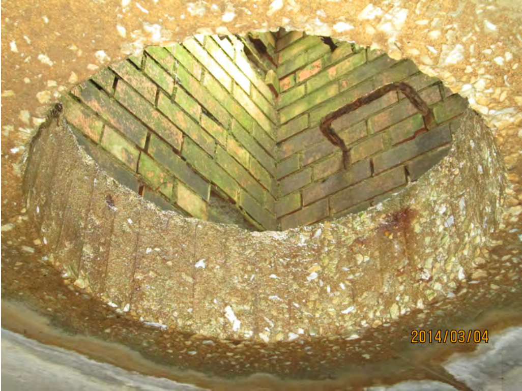
Drop Inlet in Center Barrel
