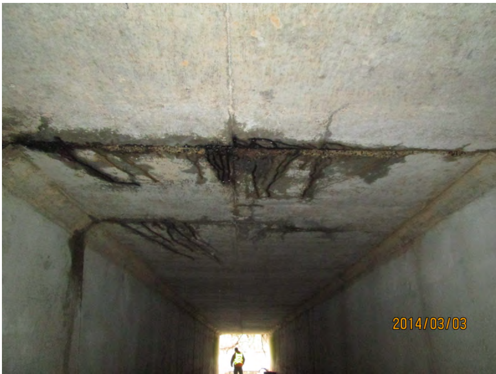
Crack in the Top Slab
