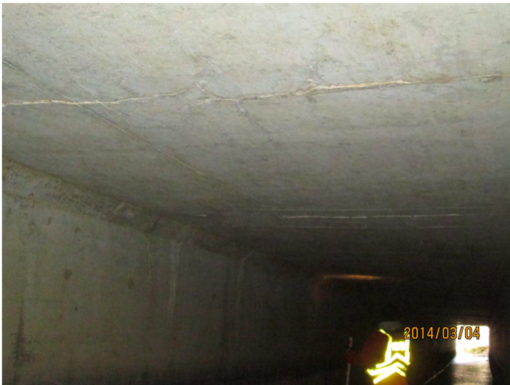
Cracks on the Top Slab Inside of the Barrel
