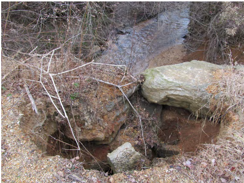
Erosion on top of 78" CMP
