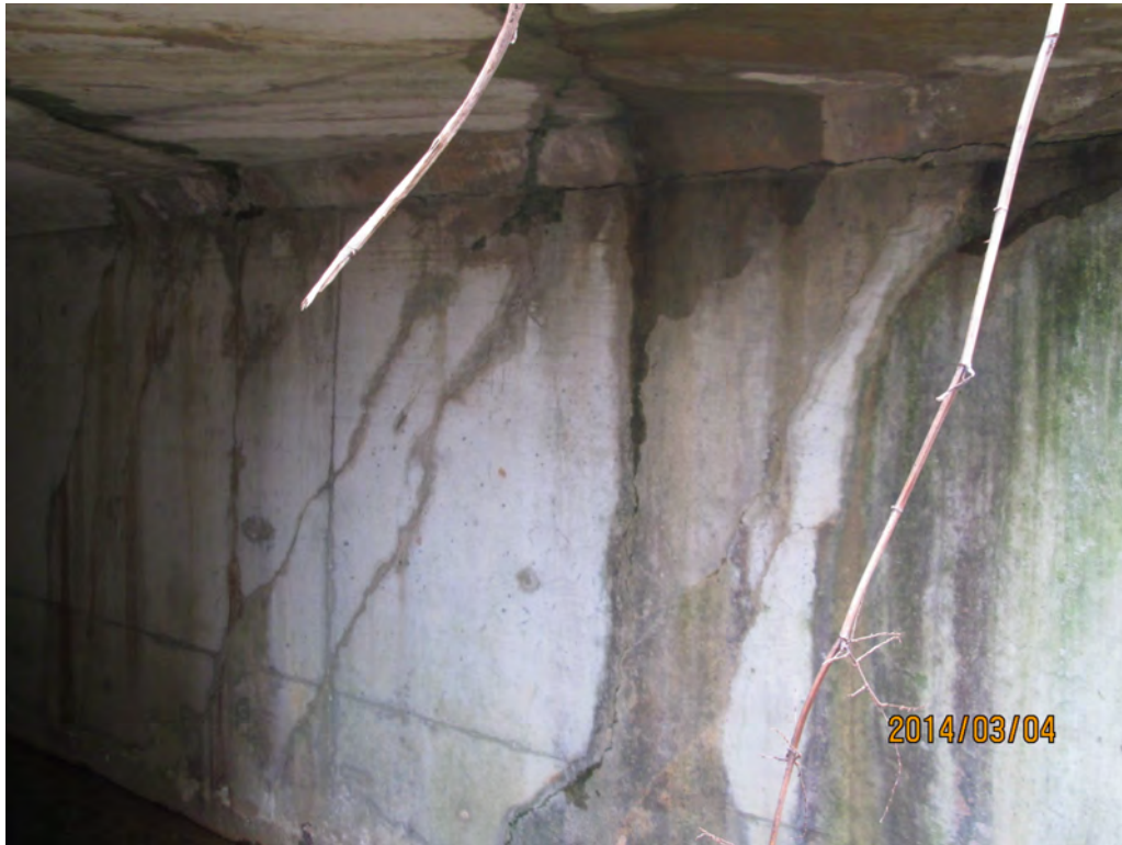
Cracks on Downstream Side and Top Slab of the Barrel
