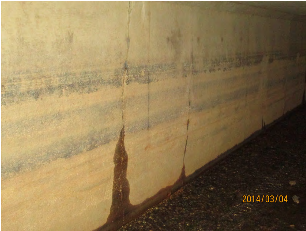
Cracks on the Side of the Wall Inside of the Barrel
