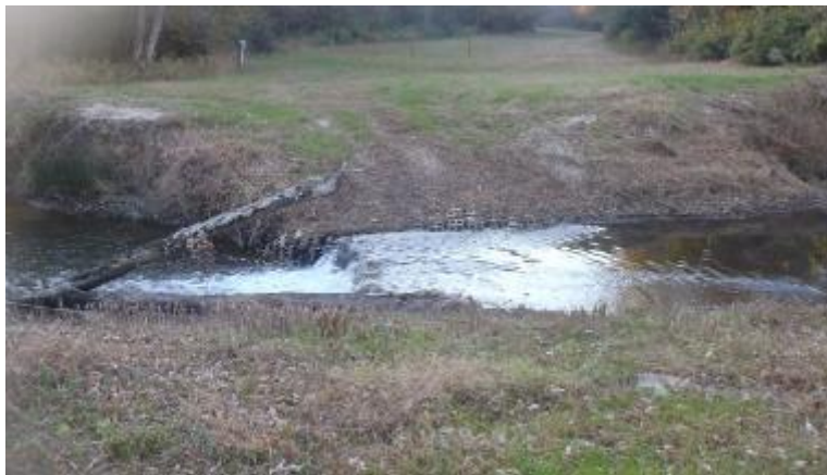
Photo 2. Perched Utility Crossing in East Braid of Swift Creek below NC 42
