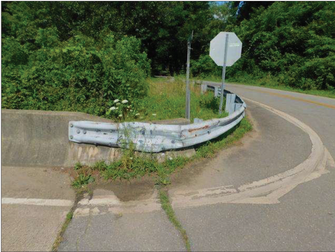
NORTH WEST GUARD RAIL CONNECTION: SCRAPE DAMAGE 10' LONG BEGINNING AT ATTACHMENT TO BRIDGE WITH ONE RAIL POST DISPLACED.
