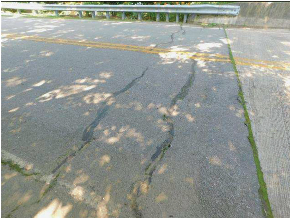
SOUTH APPROACH: SETTLEMENT AND TRANSVERSE CRACKING IN THE APPROACH WEARING SURFACE FOR 8' LONG BEGINNING AT THE FILL FACE.
