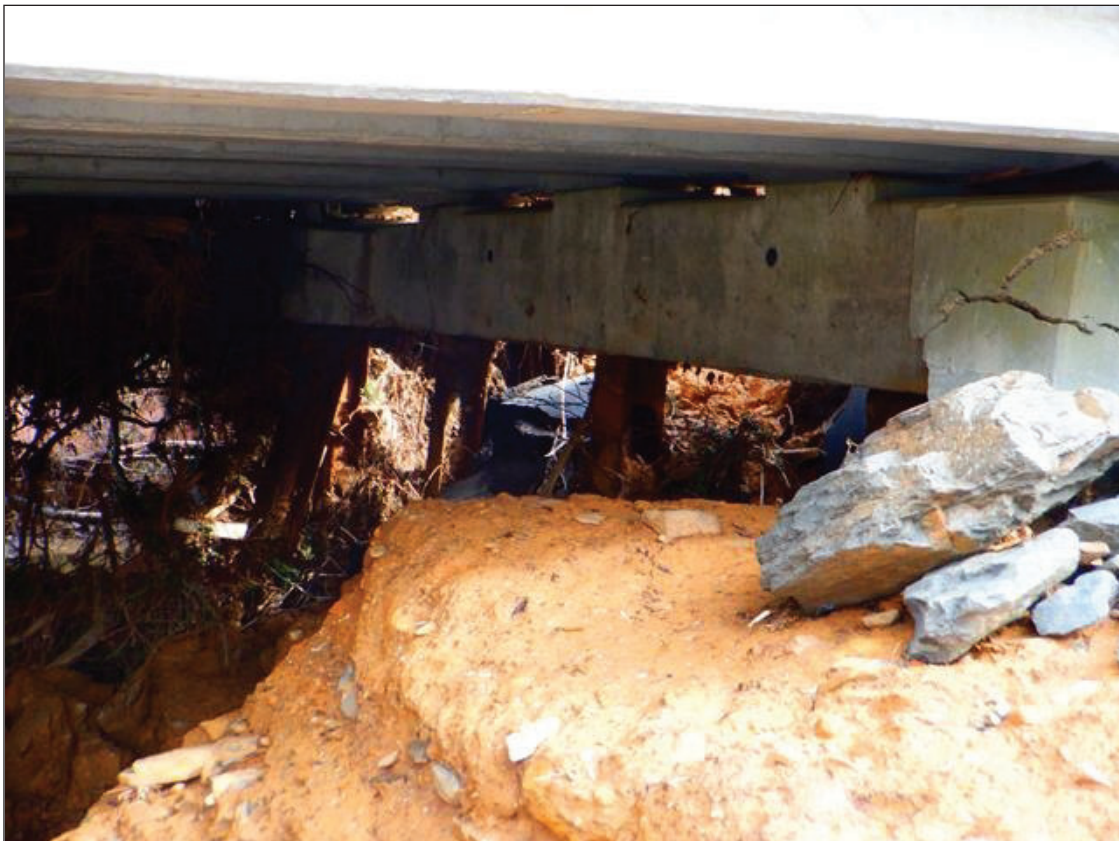
END BENT 1 HAS FAILED. EXPOSED PILES. CAP HAS WIDE CRACKS AND SPALLED AREAS. (PAR)
