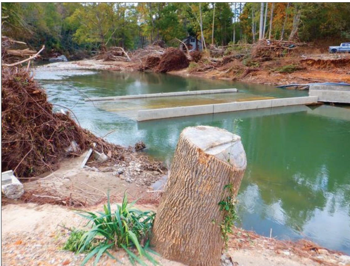
SPAN 2 AND SPAN 3 FAILED. SPANS ARE DOWNSTREAM. (PAR)
