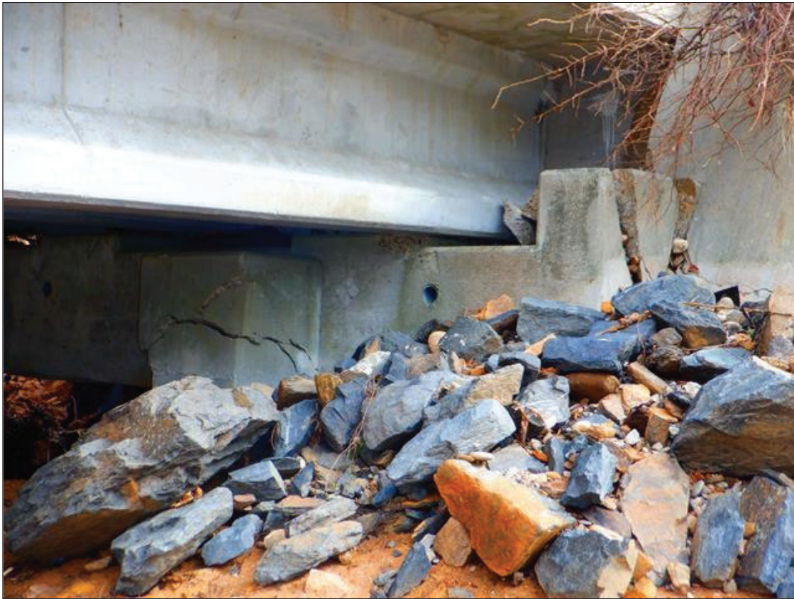
END BENT 1 HAS FAILED. EXPOSED PILES. CAP HAS WIDE CRACKS AND SPALLED AREAS. (PAR)
