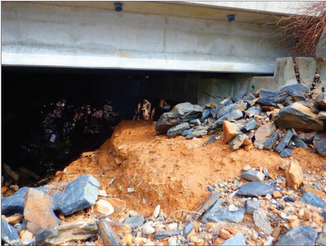
END BENT 1 HAS FAILED. EXPOSED PILES. CAP HAS WIDE CRACKS AND SPALLED AREAS. (PAR)
