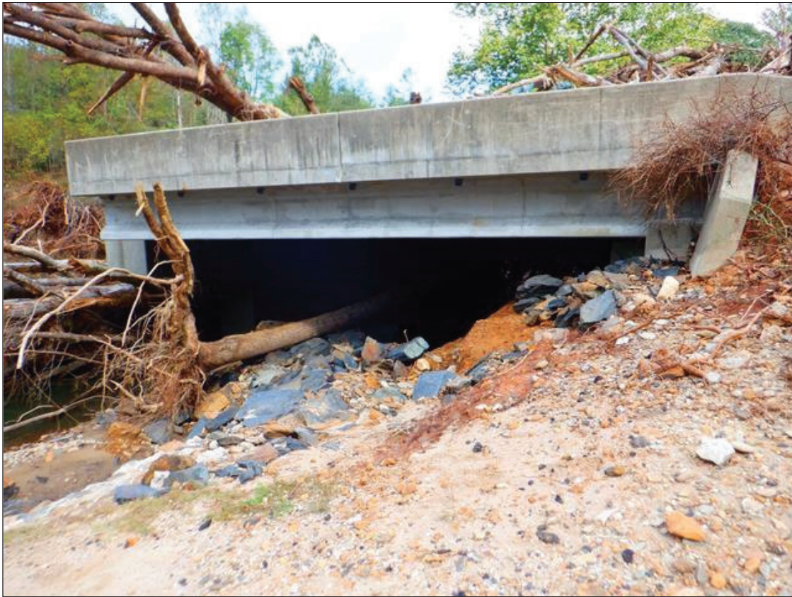
SPAN 1: PRECASTED GIRDER HAS SHIFTED DOWNSTREAM UP TO 2 FEET. (PAR)
