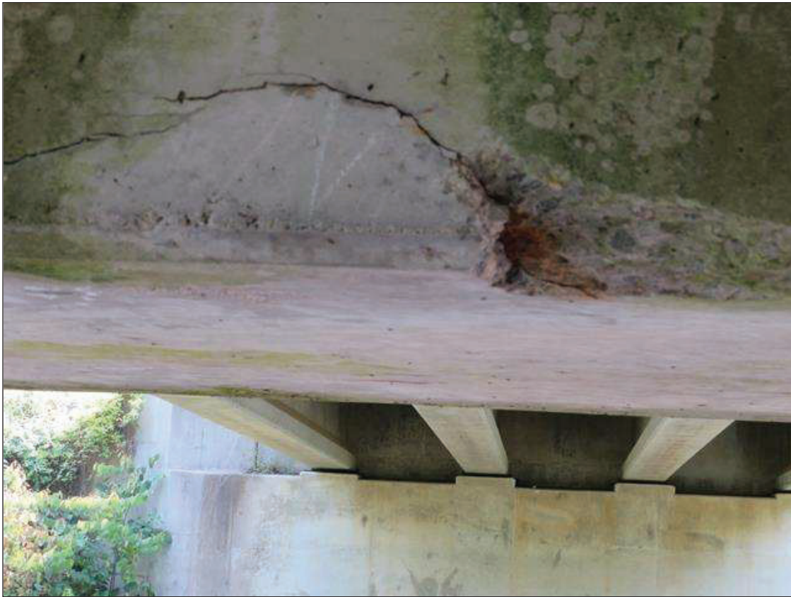
Bent 3 Cap 1: SOUTH FACE AT BOTTOM CORNER, 11 FEET FROM WEST END OF CAP, 3 FEET LONG X 6 INCHES HIGH DELAMINATED/SPALLED AREA UP TO 3 INCHES DEEP (PAR)
