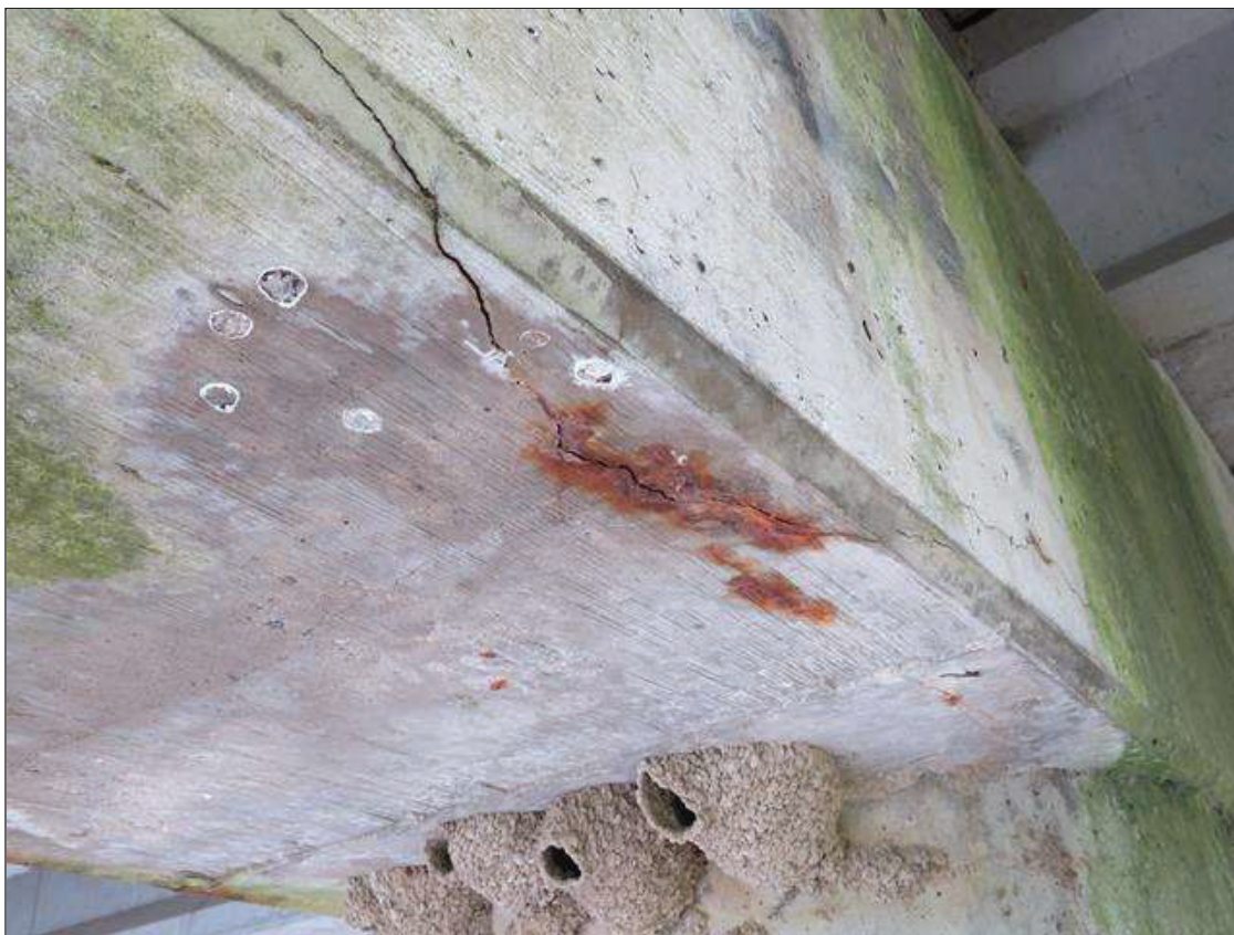
Bent 1 Cap 1: 5 FEET 1/16 INCH WIDE LONGITUDINAL CRACK WITH RUST STAINS ON BOTTOM OF CAP AT WEST END
