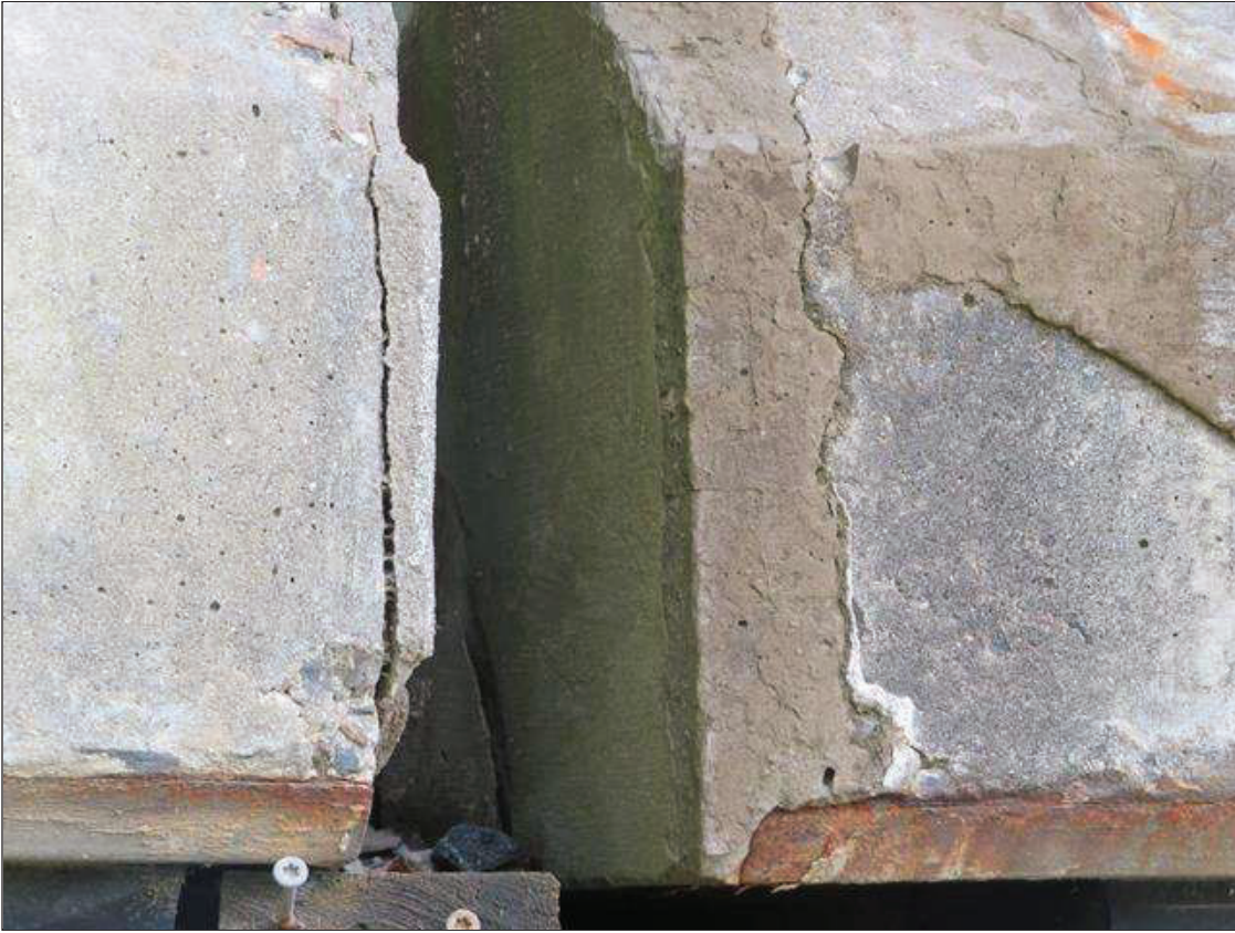
Span 2 Beam 4: SOUND PATCHING, FORMERLY 12 INCHES WIDE X 15 INCHES HIGH X 2 INCHES DEEP SPALL, WITH EXPOSED STRAND ENDS, SOUTH FACE
