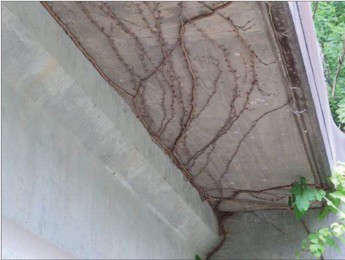
40 FEET OF VEGETATION GROWTH IN WEST OVERHANG
