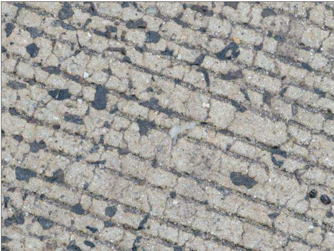
Span 1 Deck: TOP OF THE DECK, MAP CRACKING TO 1/32 INCH THROUGHOUT
