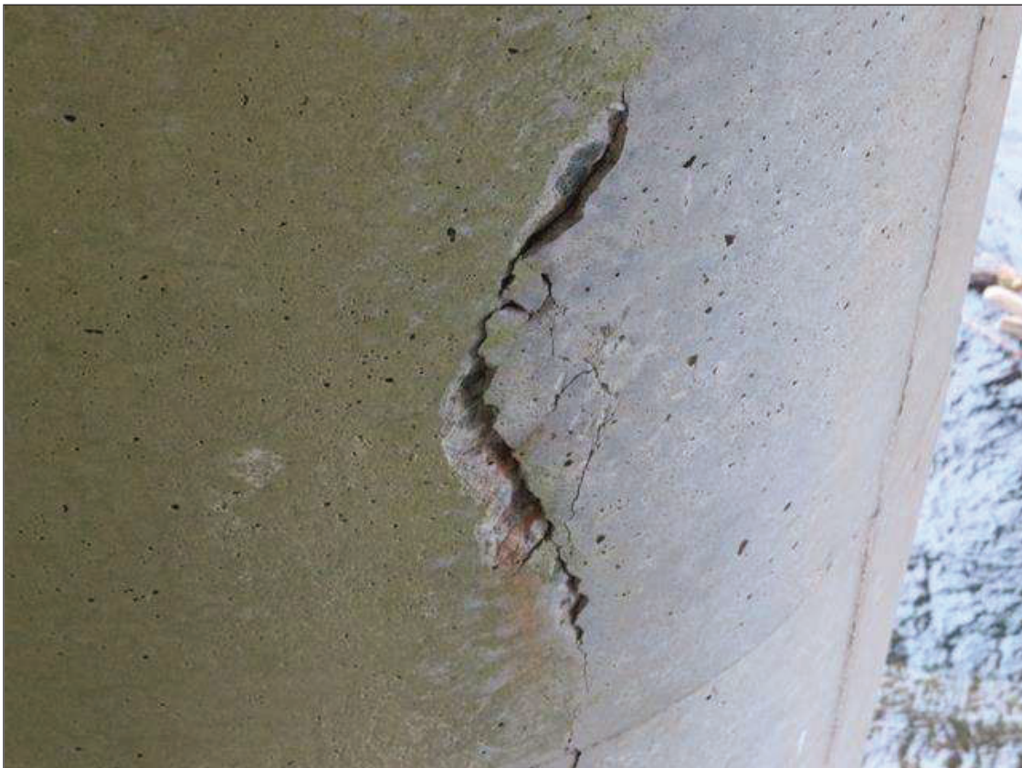
Bent 1 Pile 1: 4 FEET HIGH X 10 INCHES WIDE X 1/2 INCH DEEP SPALL AND AREA OF DELAMINATION WITH EFFLORESCENCE ON SOUTHEAST FACE, 5 FEET FROM BOTTOM OF CAP
