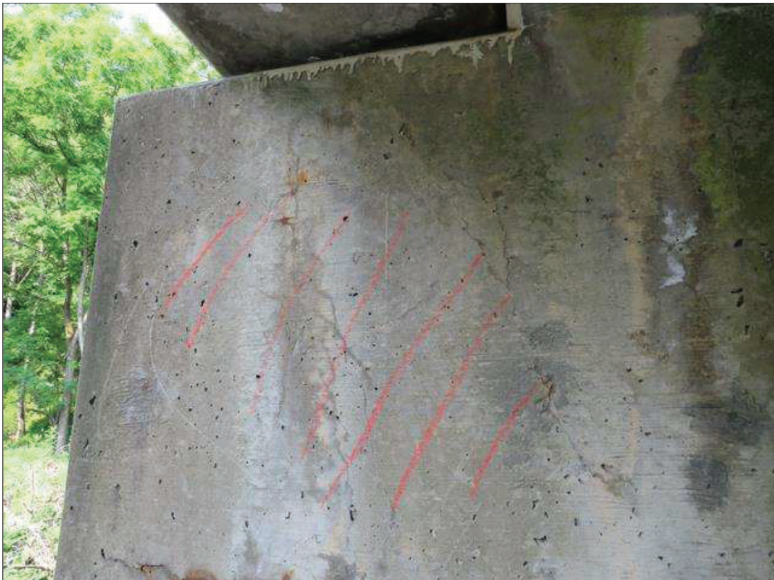
Bent 1 Cap 1: 30 INCHES DIAMETER DELAMINATED AREA WITH RUST STAINING, NORTH FACE, EAST END OF CAP
