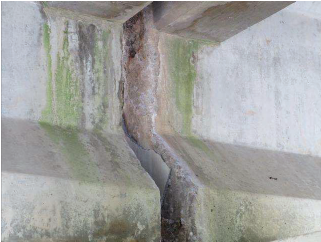
Span 2 Beam 3: GIRDER END AT BENT 2, AT THE END OF THE GIRDER FOR FULL HEIGHT, SPALLING UP TO 1 INCH DEEP. THE TIPS OF THE PRESTRESSING ARE EXPOSED (PAR)
