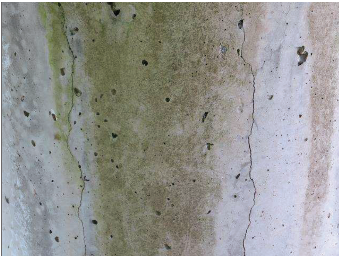
Bent 2 Pile 2: SCATTERED IN THE COLUMN, ON BOTH SIDES, VERTICAL CRACKING AND MAP CRACKING TO 1/16 INCH WIDE WITH ASSOCIATED DELAMINATION
