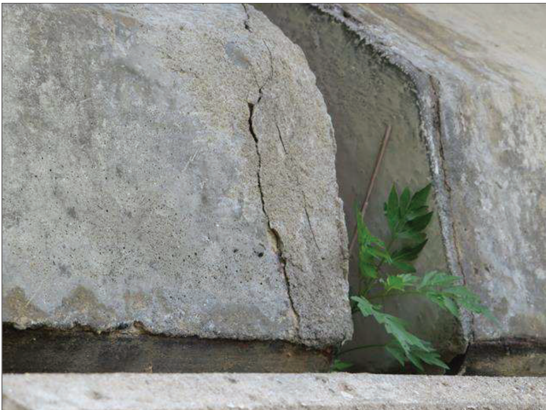
Span 3 Beam 4: GIRDER END ON RIGHT SIDE AT BENT 3 APPROXIMATELY 3 INCHES BACK, VERTICAL CRACKING TO 1/16 INCH WIDE
