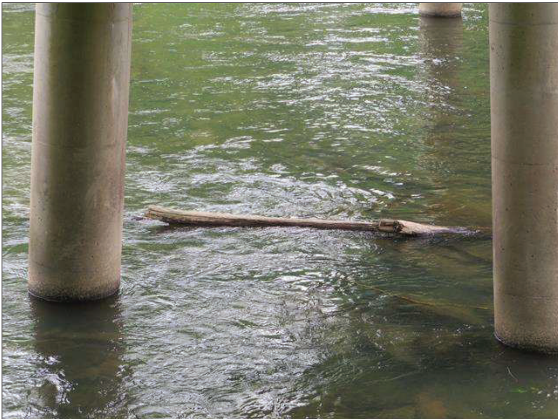
DRIFT AT NORTH SIDE OF BENT 1, 2 INCHES TO 10 INCHES DIAMETER
