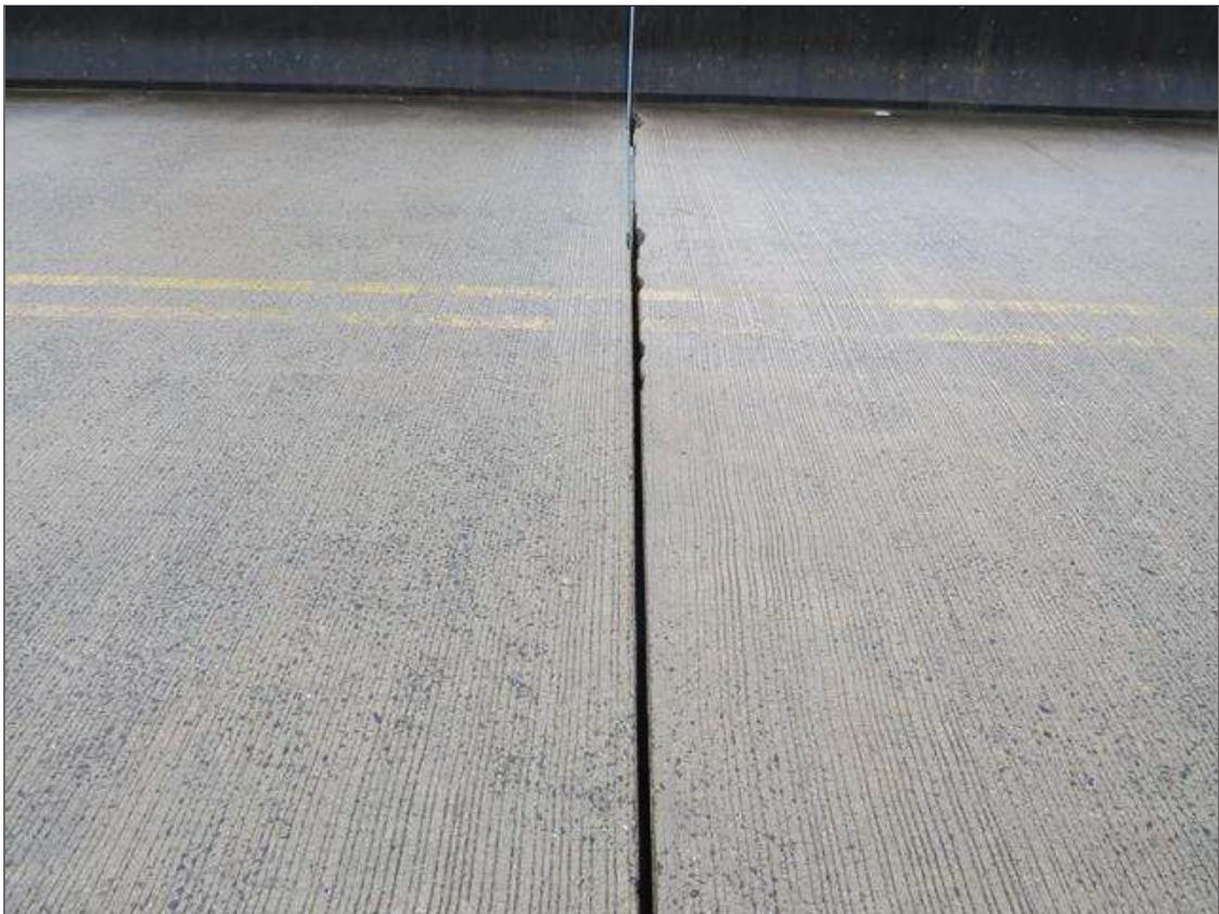
BENT 3 OPEN JOINT
