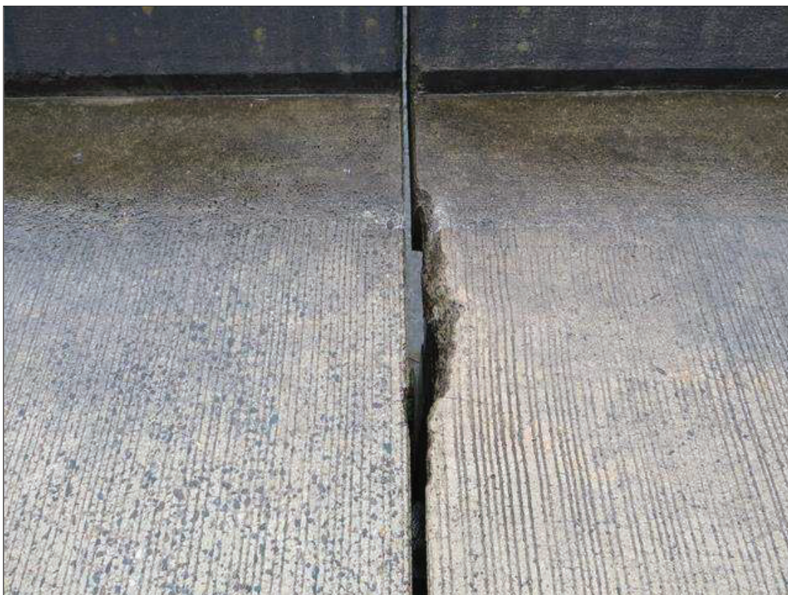
Span 3 Deck: SPALLED AREA (2 FEET WIDE X 3 INCHES LONG X 4 INCHES DEEP) AT NORTH END ADJACENT TO RIGHT RAIL (PAR)
