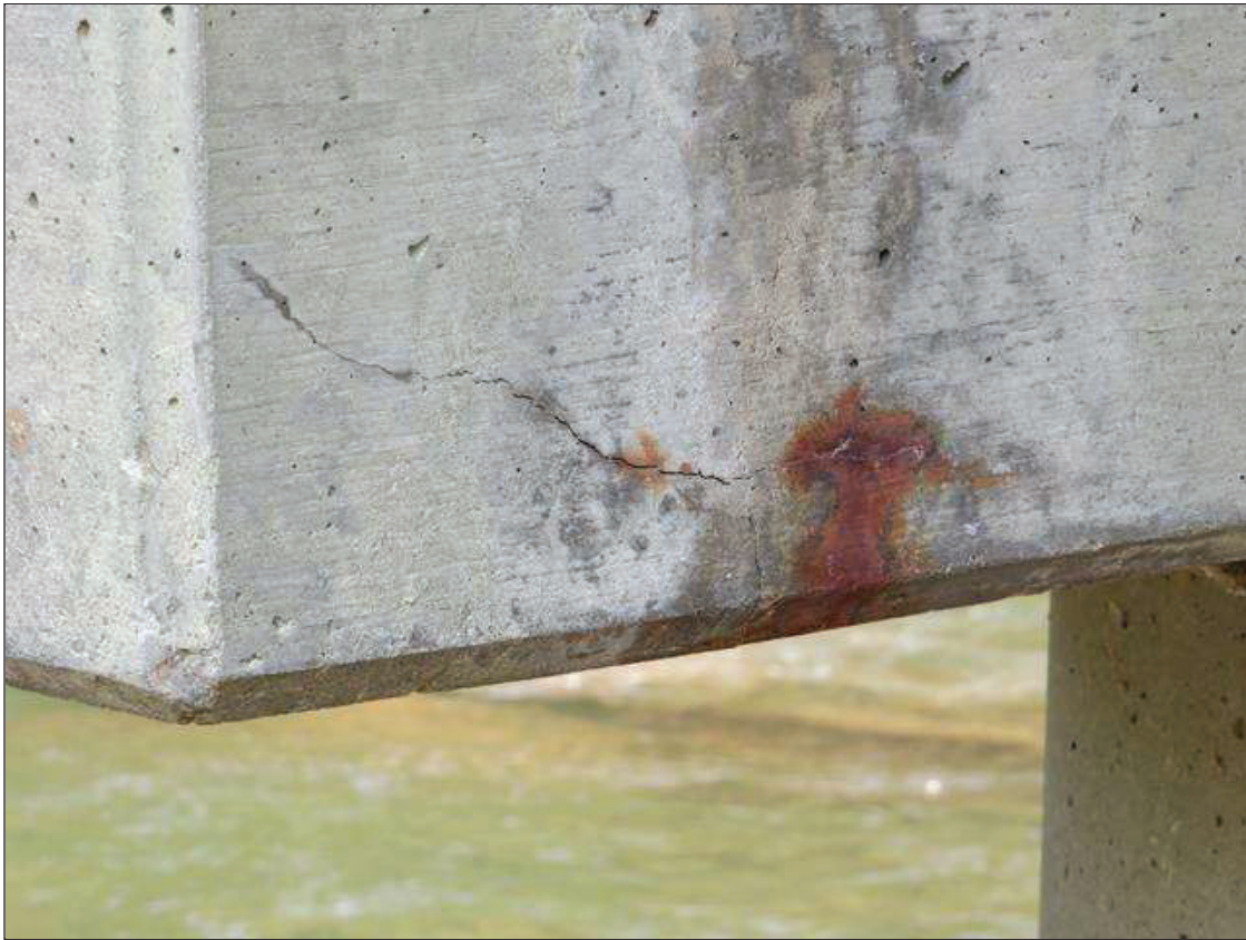
Bent 3 Cap 1: NORTH FACE, LOWER 3 INCHES OF THE CAP AT THE EAST END, HORIZONTAL CRACKING WITH RUST LEAKAGE TO 1/16 INCH WIDE
