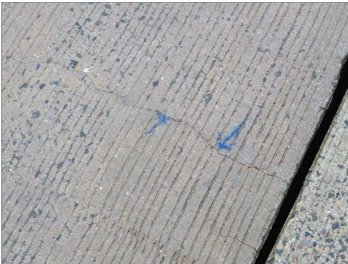
Span 2 Deck: 5 SQUARE FEET HAIRLINE LONGITUDINAL AND TRANSVERSE CRACKS EXTENDING FROM BENT 1 JOINT
