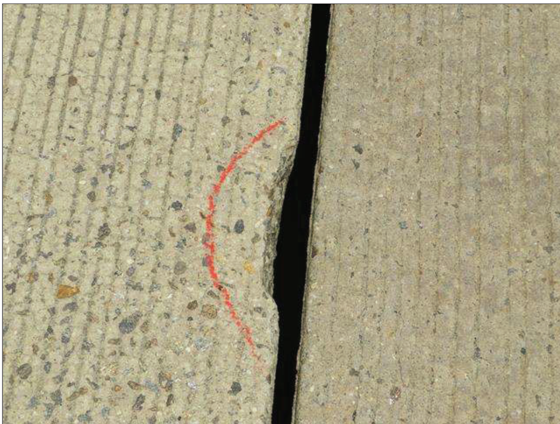
Span 2 Expansion Joint: BENT 1 OPEN JOINT, CHIPPING UP TO 7 INCHES WIDE X 3/4 INCHES LONG X 3/4 INCHES DEEP, SCATTERED
