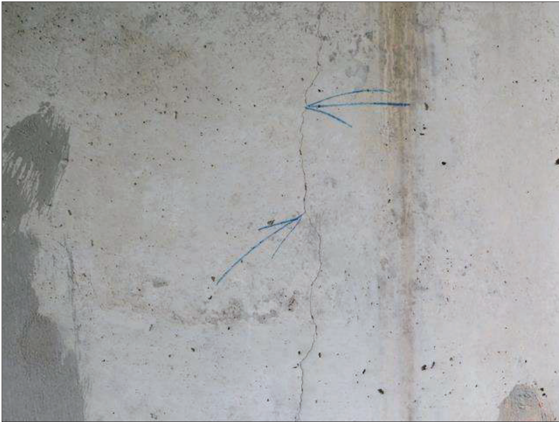
End Bent 1 Abutment: (2) UP TO 12 FEET X 1/64 INCH WIDE VERTICAL CRACKS, AT RANDOM THROUGHOUT NORTH FACE.
