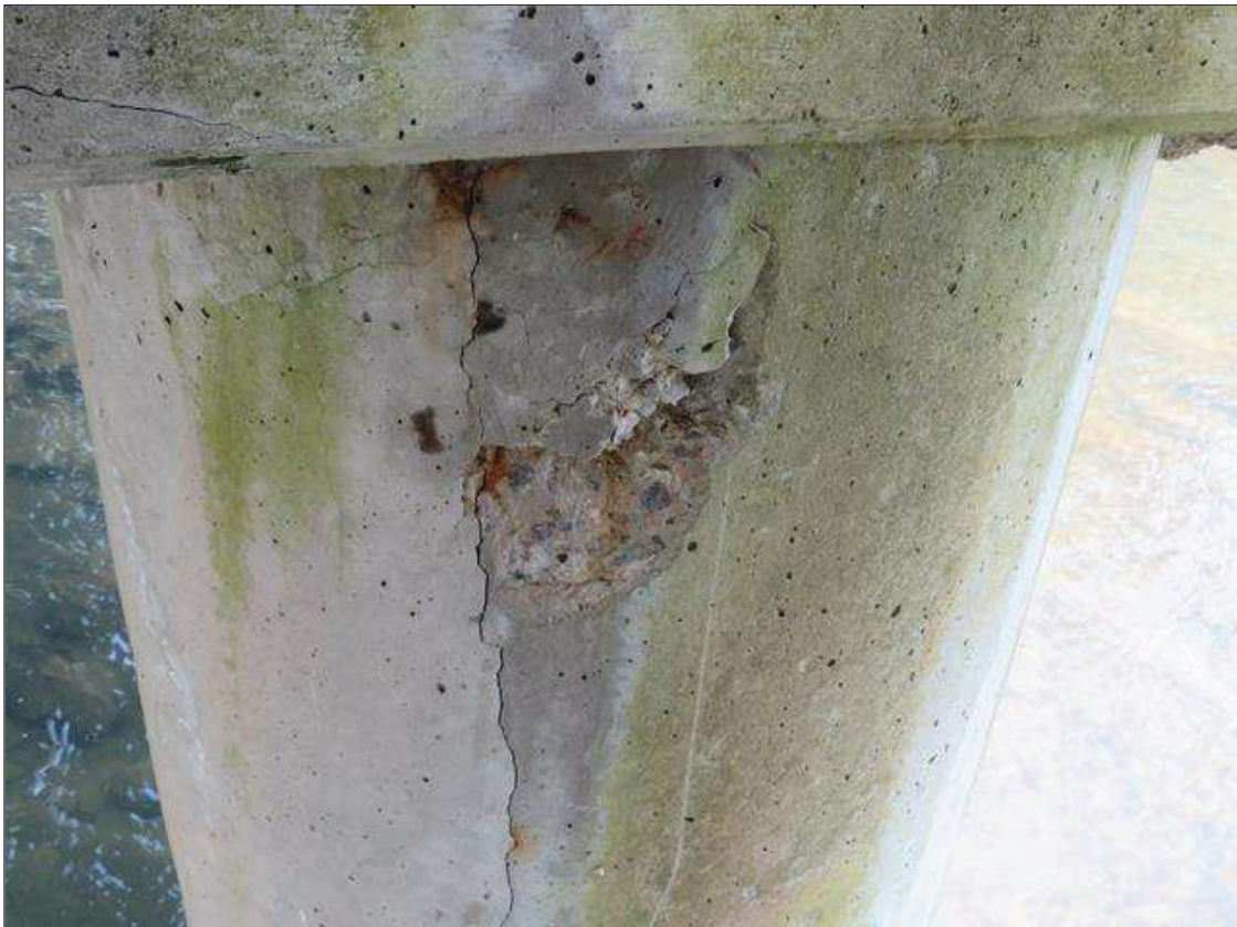
Bent 2 Pile 1: NORTH SIDE ADJACENT TO BOTOM OF CAP, SPALLED AREA WITH ADJACENT DELAMINATION 1 FOOT HIGH X 8 INCHES WIDE X 1 INCH DEEP
