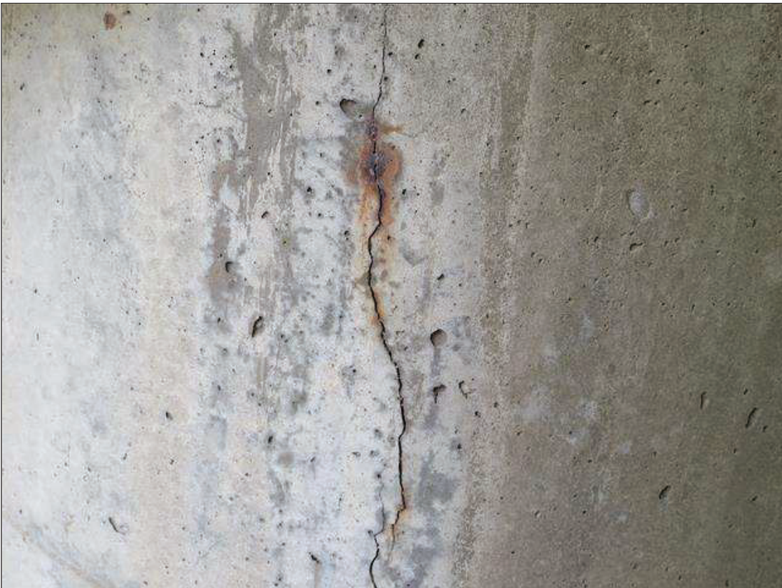
Bent 1 Pile 2: SCATTERED IN THE COLUMN, GENERALLY ON THE NORTH SIDE, VERTICAL CRACKING AND MAP CRACKING TO 1/16 INCH WIDE WITH RUST STAINING
