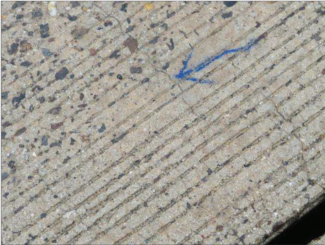
Span 4 Deck: 3 SQUARE FEET HAIRLINE LONGITUDINAL CRACKS EXTENDING FROM BENT 3 JOINT
