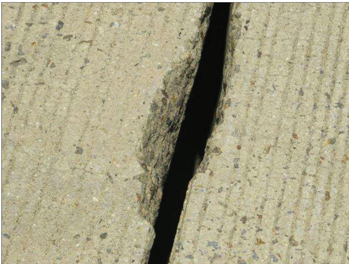
Span 4 Expansion Joint: BENT 3 OPEN JOINT, CHIPPING UP TO 24 INCHES WIDE X 3 INCHES LONG X 4 INCHES DEEP, SCATTERED
