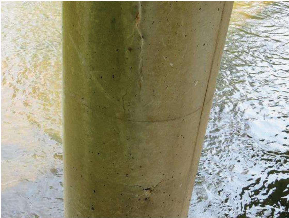
Bent 2 Pile 1: 12 FEET HIGH X 1 FOOT WIDE X 1 INCH DEEP SPALL WITH EXPOSED REBAR AND AREA OF DELAMINATION ON SOUTH FACE
