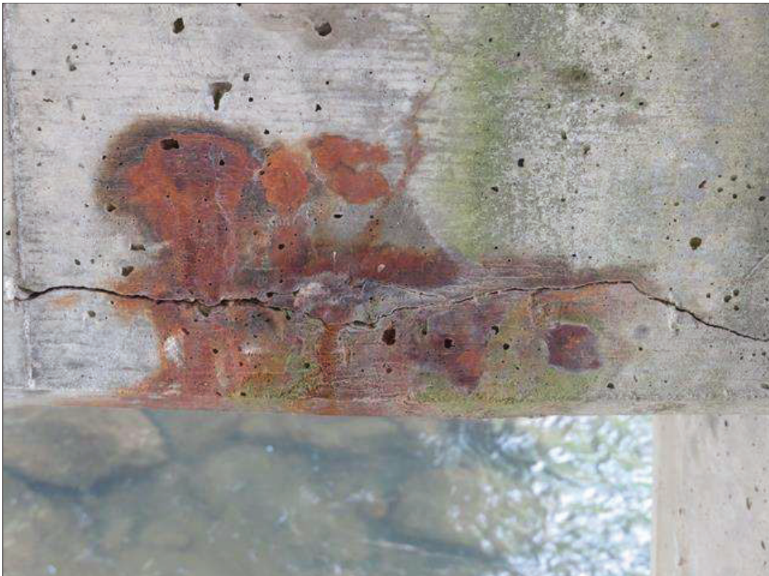
Bent 2 Cap 1: LOWER 3 INCHES OF THE CAP, SCATTERED ALONG THE LENGTH OF CAP UNDER BAYS 1 AND 2, HORIZONTAL CRACKING TO 1/16 INCH WIDE WITH RUST STAINING
