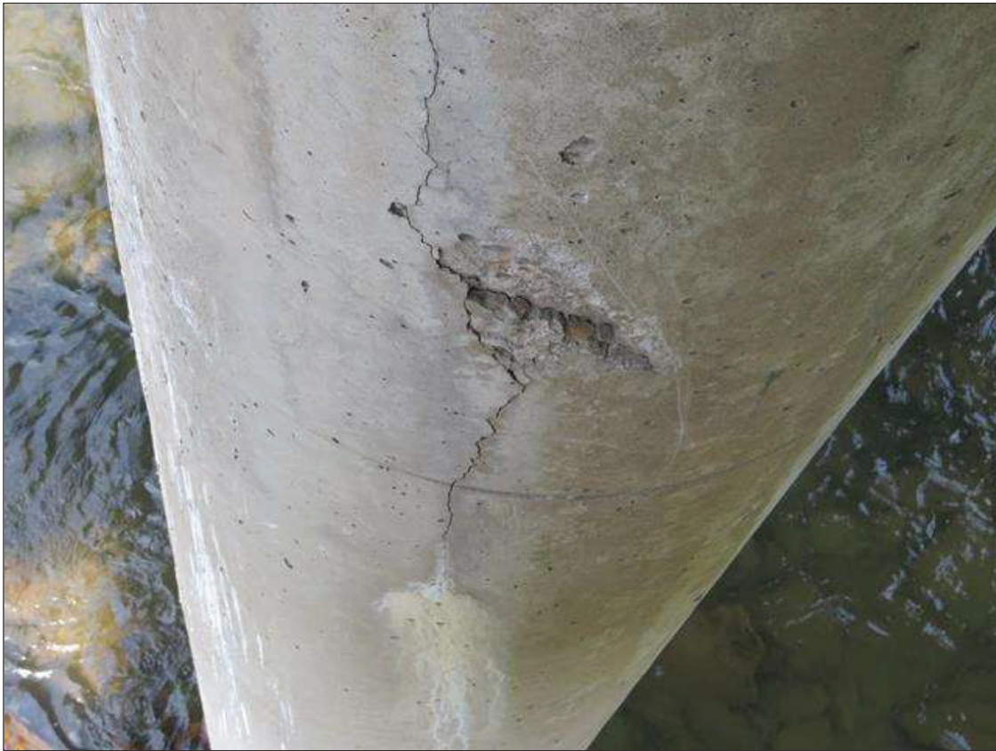
Bent 2 Pile 2: 4 FEET HIGH X 10 INCHES WIDE AREA OF DELAMINATION WITH 8 INCHES HIGH X 8 INCHES WIDE X 1/2 INCH DEEP SPALL ON NORTH FACE
