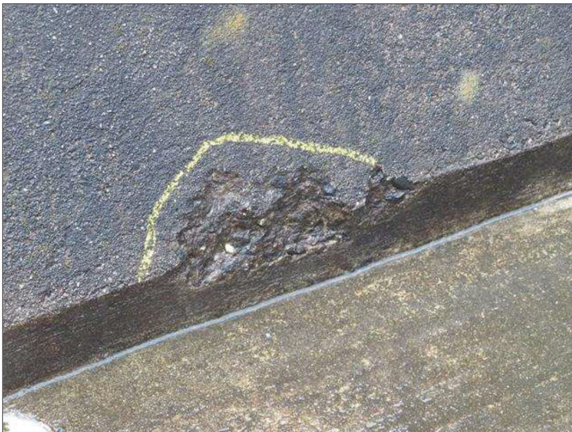
Span 4 Right Bridge Rail: 9 INCHES LONG X 3 INCHES HIGH X 1/2 INCH DEEP SPALL, 17 FEET FROM BENT 3
