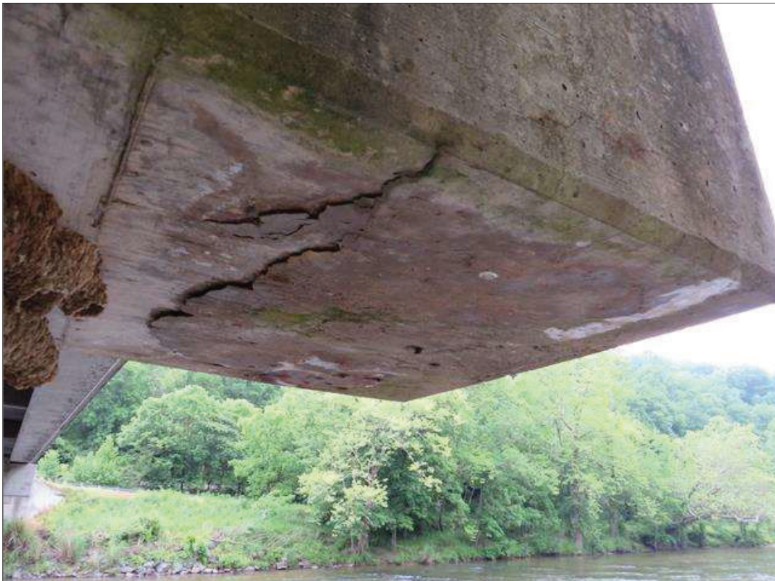
Bent 1 Cap 1: 22 INCHES LONG X 30 INCHES WIDE AREA OF DELAMINATION ON BOTTOM OF CAP AT EAST END
