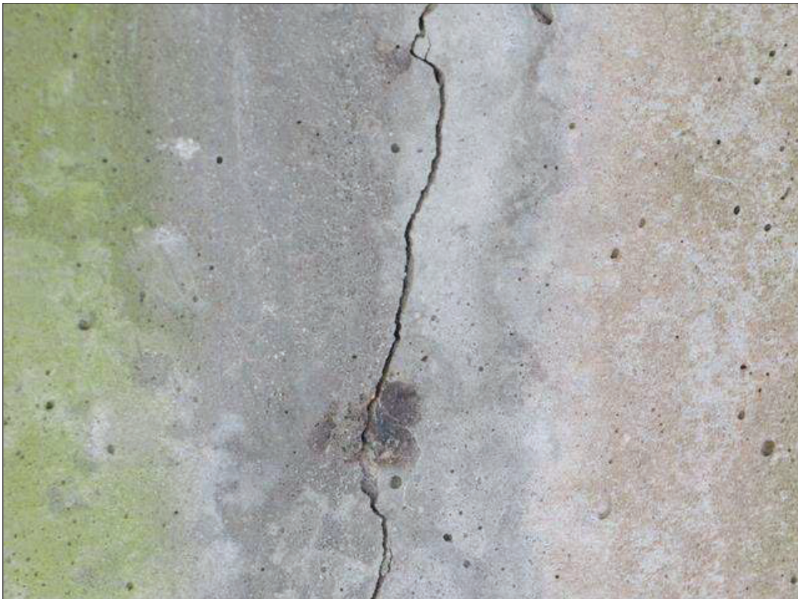
Bent 2 Pile 1: SCATTERED IN THE COLUMN, ON BOTH SIDES, VERTICAL CRACKING AND MAP CRACKING TO 1/16 INCH WIDE AND SCATTERED RUST STAINING
