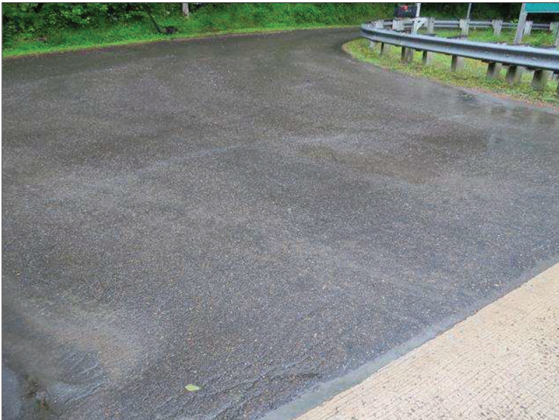
END BENT 1 ASPHALT WEARING SURFACE APPROACH 30 SQUARE FEET OF UP TO 1/4 INCH WIDE CRACKING
