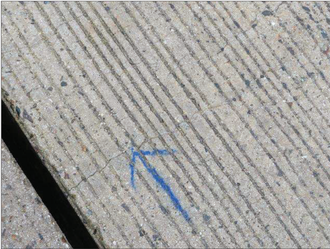
Span 3 Deck: 7 SQUARE FEET HAIRLINE LONGITUDINAL CRACKS EXTENDING FROM BENT 2 JOINT
