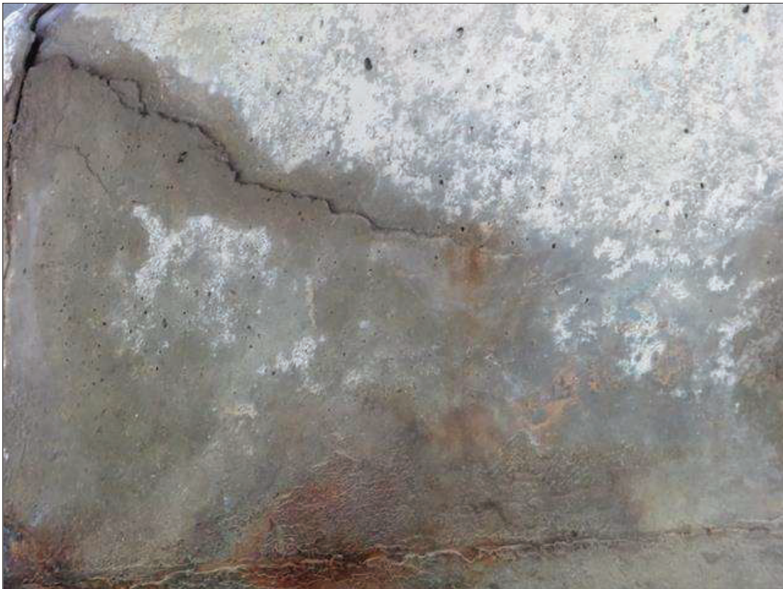
Span 3 Beam 2: GIRDER END AT BENT 2, RIGHT LOWER FLANGE, DIAGONAL CRACKING TO 1/32 INCH WIDE WITH RUST STAINING AND ADJACENT DELAMINATION 10 INCHES LONG X 8 INCHES HIGH
