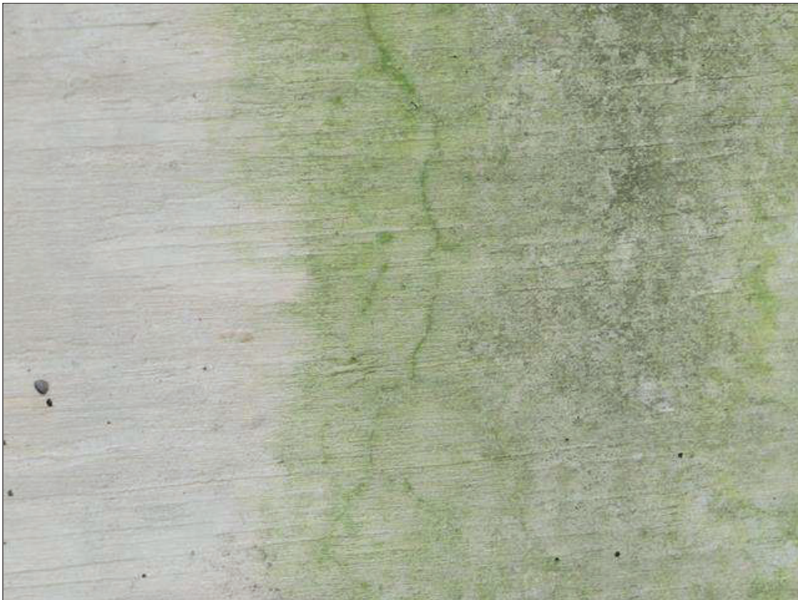
Bent 3 Cap 1: SCATTERED IN THE CAP FACES, HAIRLINE MAP CRACKING
