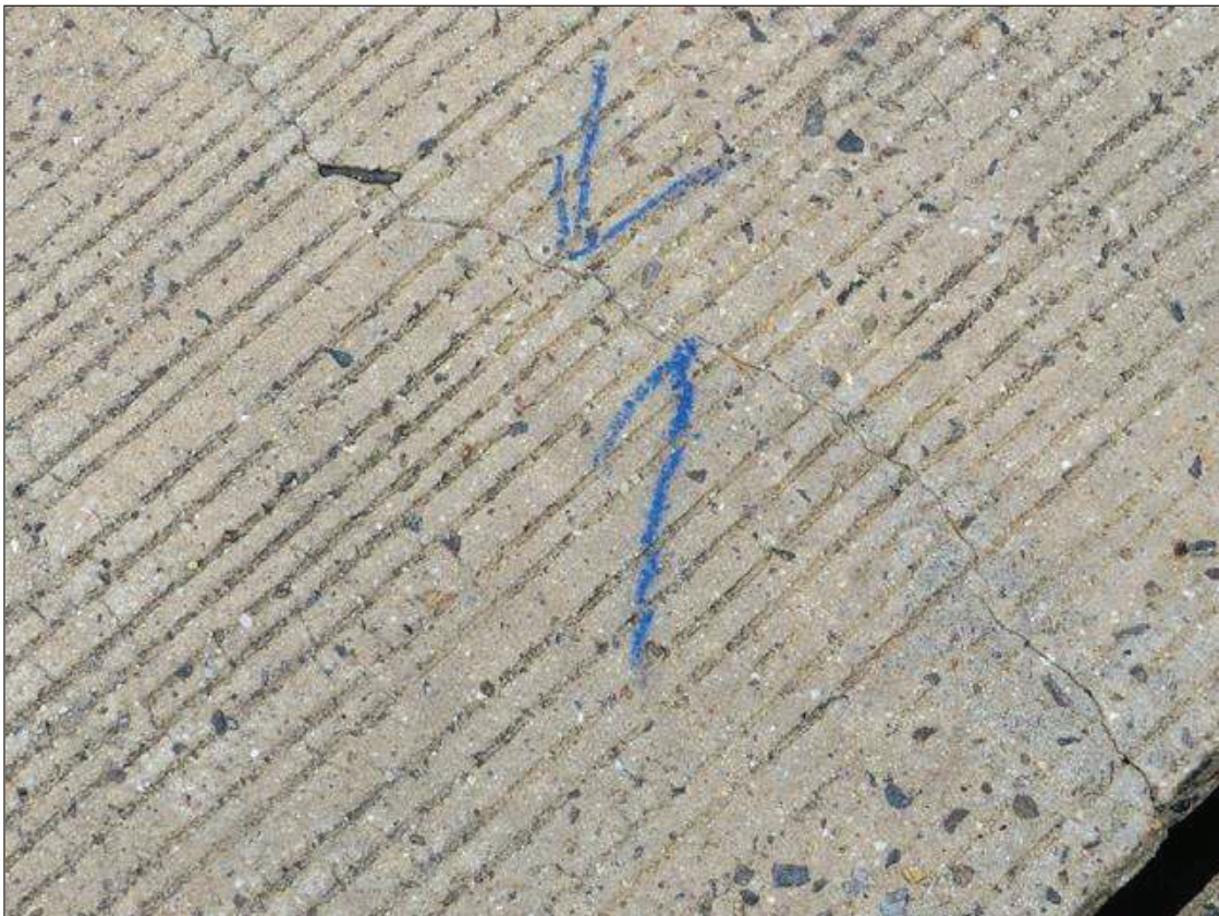
Span 3 Deck: 12 SQUARE FEET HAIRLINE LONGITUDINAL CRACKS EXTENDING FROM BENT 3 JOINT
