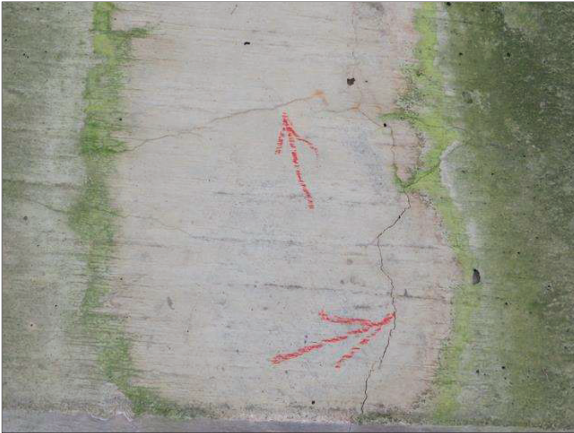
Bent 1 Cap 1: SCATTERED IN THE CAP FACES, MAP CRACKING TO 1/32 INCH WIDE
