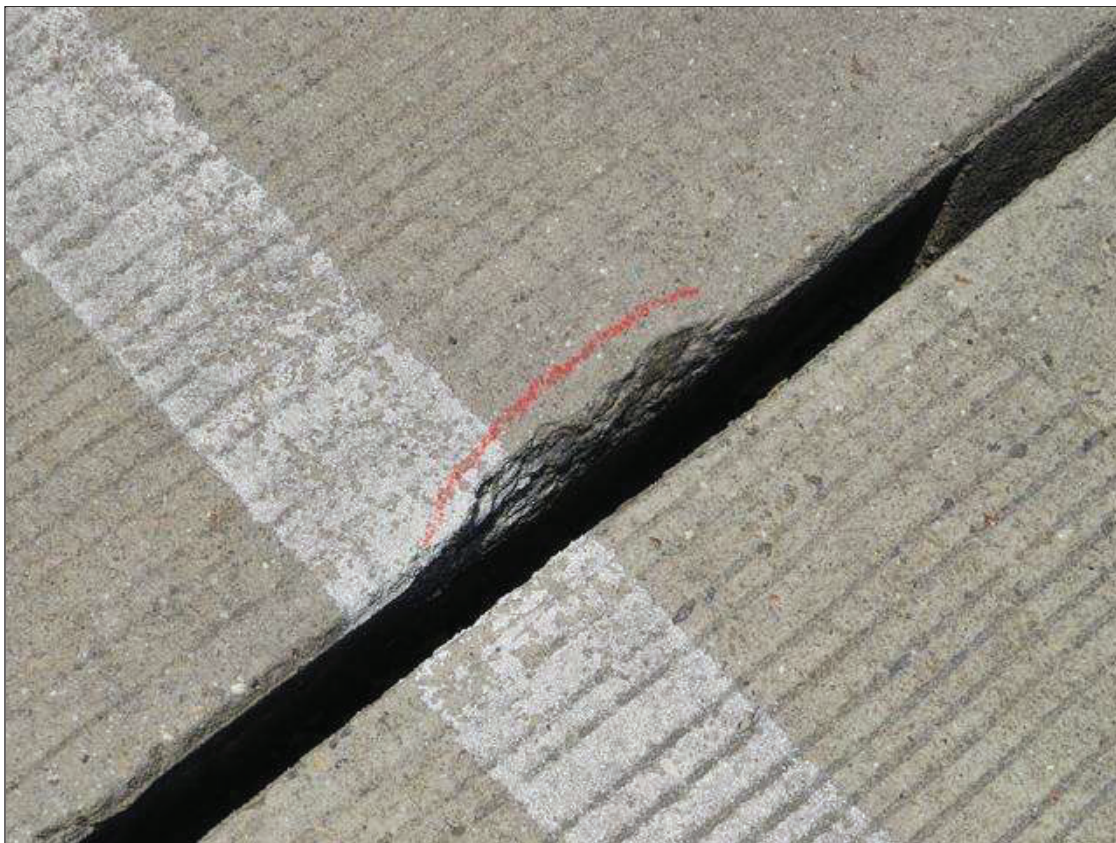
Span 3 Expansion Joint: BENT 2 OPEN JOINT, CHIPPING UP TO 5 INCHES WIDE X 3/4 INCHES LONG X 3/4 INCHES DEEP, SCATTERED
