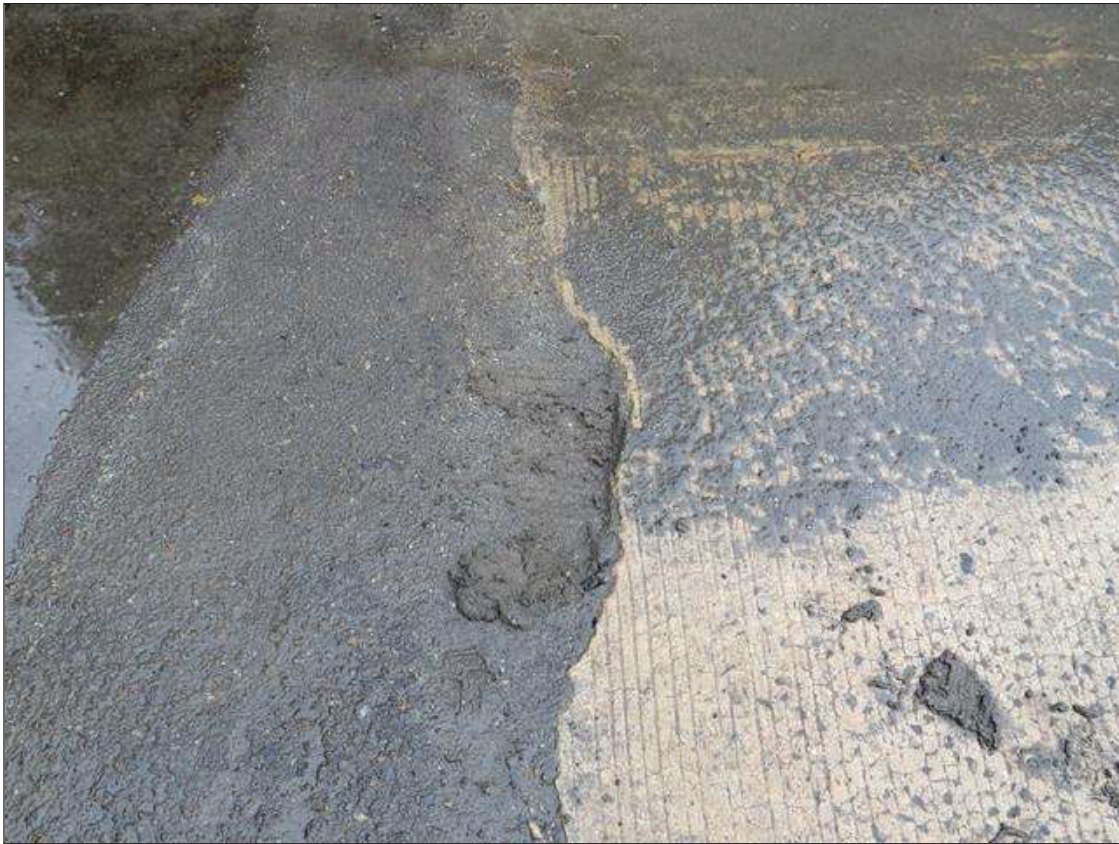
Span 1 Deck: (4) UP TO 32 INCHES WIDE X 7 INCHES LONG X 2 INCHES DEEP SPALLS ALONG END BENT 1
