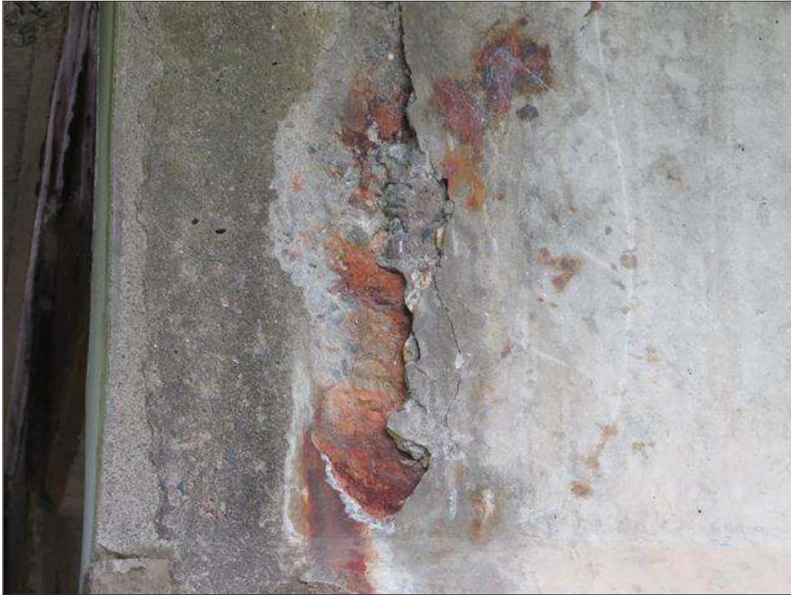
Span 2 Beam 4: GIRDER END AT BENT 1, EAST SIDE OF THE WEB, MAP CRACKING TO 1/16 INCHES WIDE WITH 9 INCHES LONG X 16 INCHES HIGH X 1/2 INCH DEEP SPALL AND AREA OF DELAMINATION WITH EFFLORESCENCE STAINING, AND RUST STAINING (PAR)
