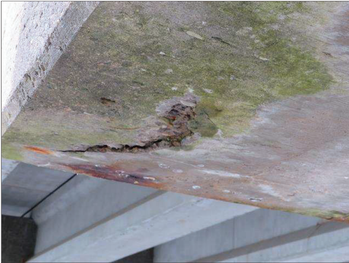
Bent 1 Cap 1: 12 INCHES DIAMETER X 1 INCH DEEP SPALL AND AREA OF DELAMINATION ON BOTTOM OF CAP AT WEST END
