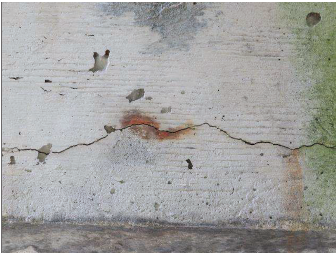
Bent 1 Cap 1: LOWER 3 INCHES OF THE CAP, SCATTERED ALONG THE LENGTH OF BOTH FACES HORIZONTAL CRACKING TO 1/16 INCH WIDE WITH RUST STAINING
