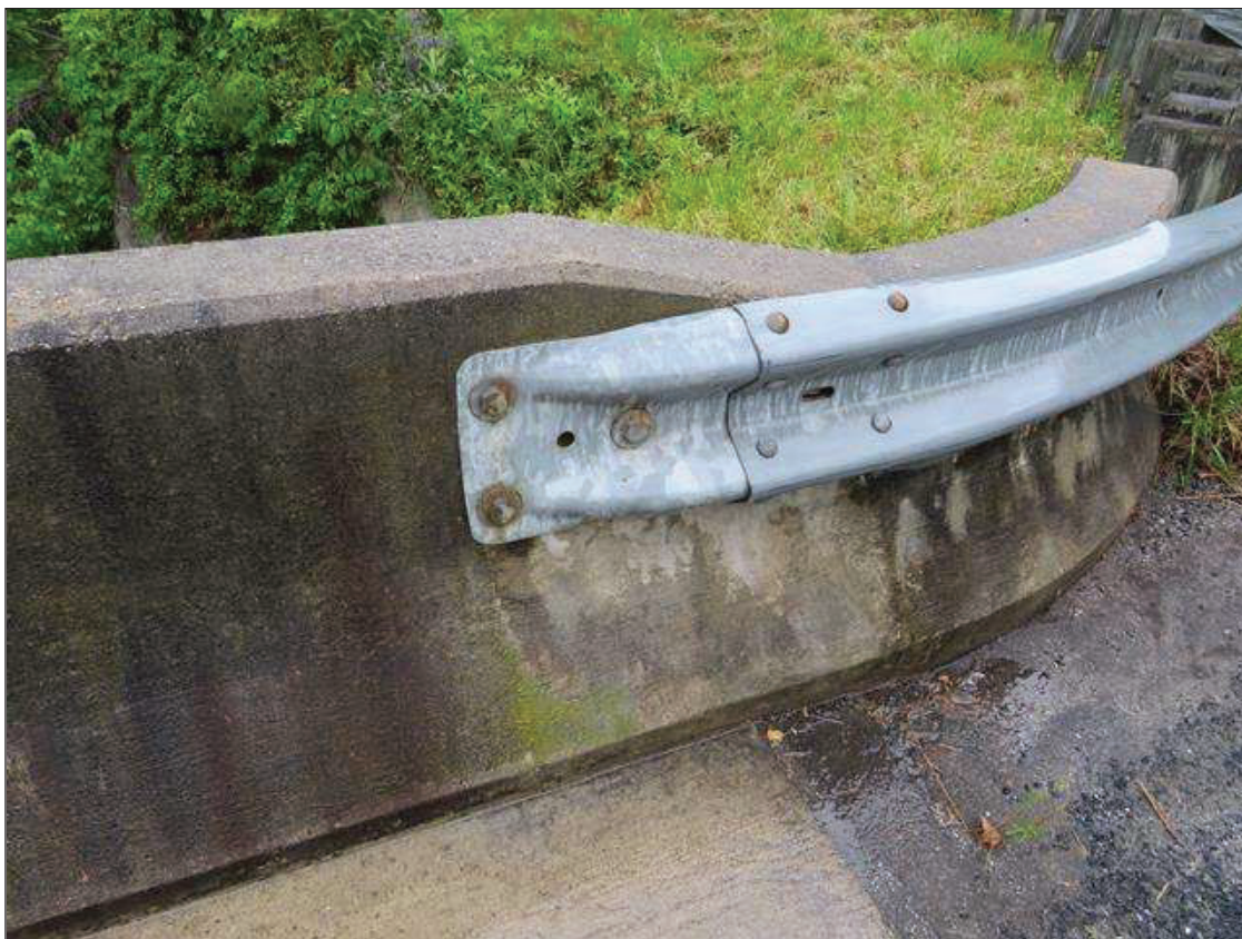
END BENT 2 LEFT SIDE GUARDRAIL ATTACHMENT MISSING 1 CONNECTION BOLT (PAR)
