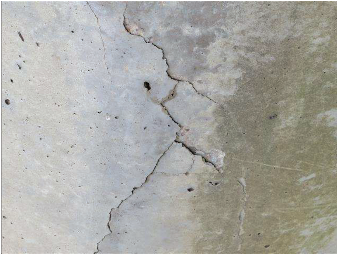
Bent 1 Pile 2: NORTH SIDE OF COLUMN, DELAMINATED AREA WITH ADJACENT SPALLS 15 FEET HIGH X 10 INCHES WIDE X 1/2 INCH DEEP
