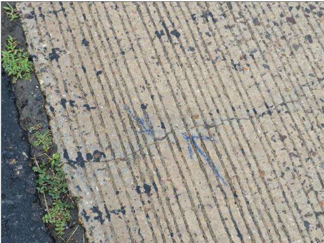
Span 4 Deck: 6 SQUARE FEET HAIRLINE LONGITUDINAL CRACKS EXTENDING FROM END BENT 2
