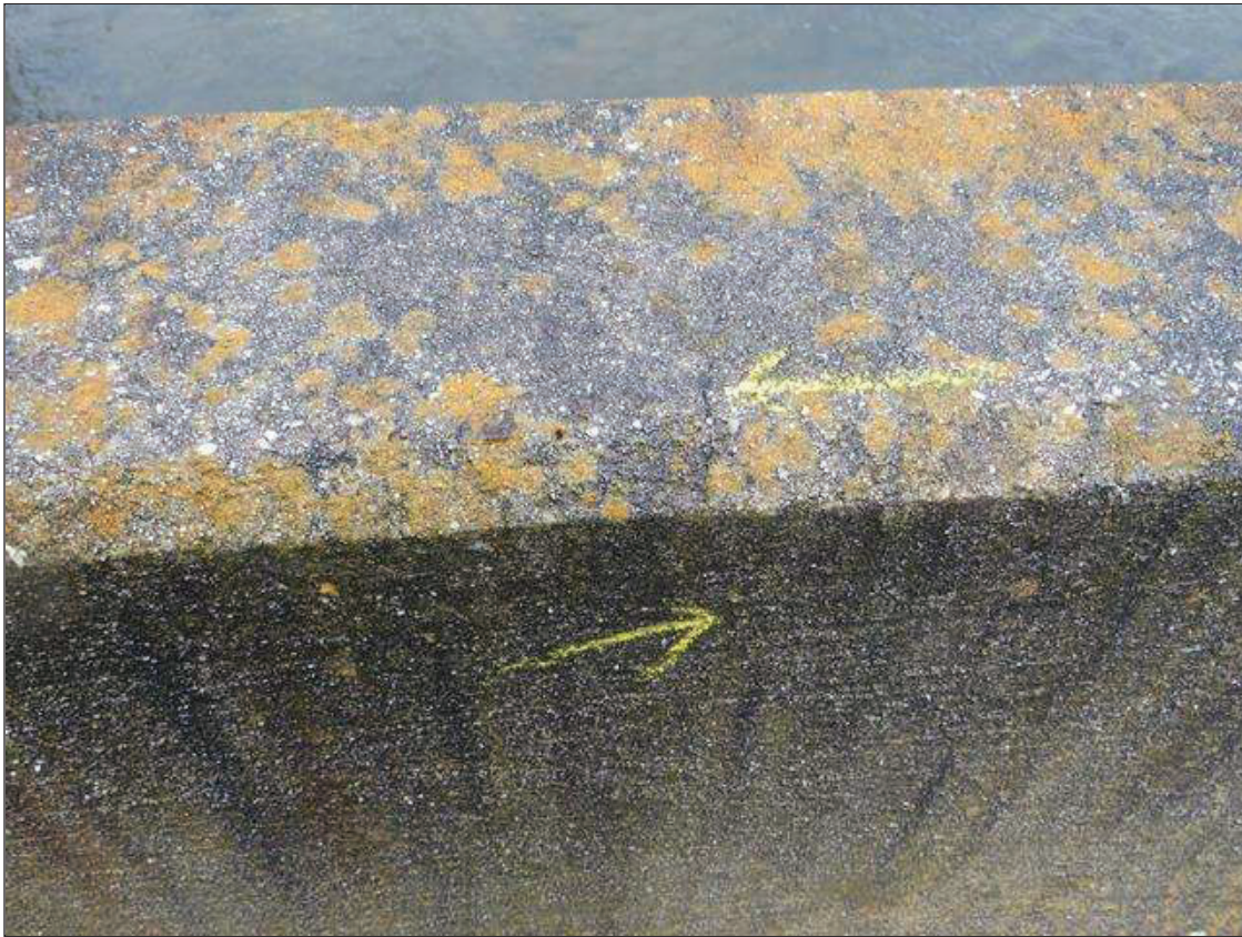
Span 2 Left Bridge Rail: (2) HAIRLINE VERTICAL AND TRANSVERSE CRACKS
