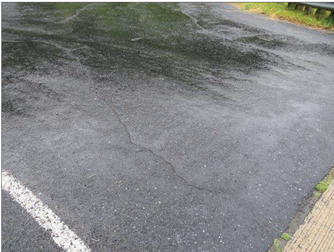
END BENT 2 ASPHALT WEARING SURFACE APPROACH 25 SQUARE FEET OF UP TO 1/8 INCH WIDE CRACKING
