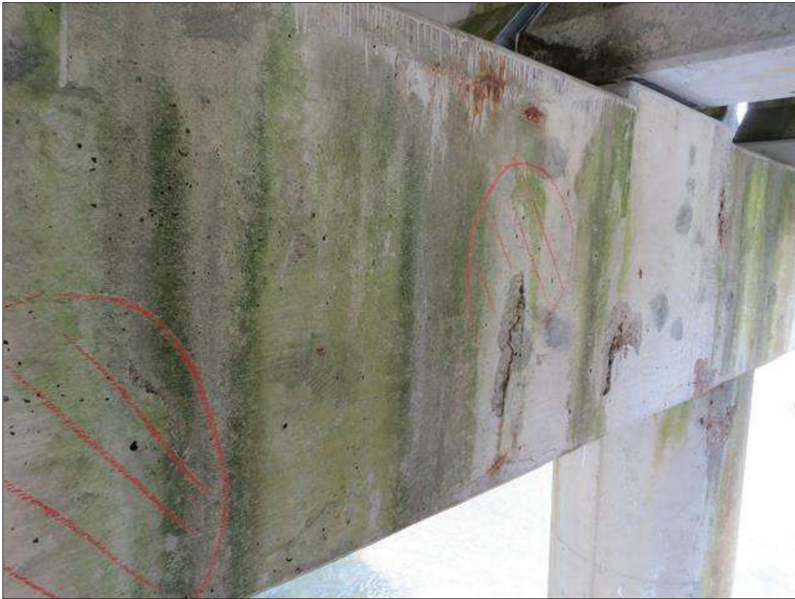
Bent 2 Cap 1: NORTH FACE AT BAY 2 AND UNDER GIRDER 2, (4) AREAS UP TO 12 INCHES DIAMETER X 3/4 INCHES DEEP SPALLS AND DELAMINATION
