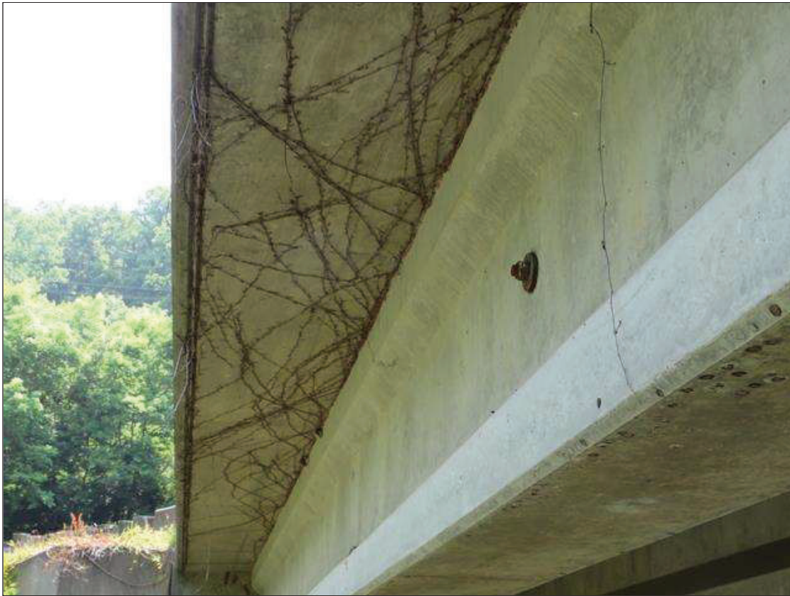
40 FEET LONG VEGETATION GROWTH IN WEST OVERHANG
