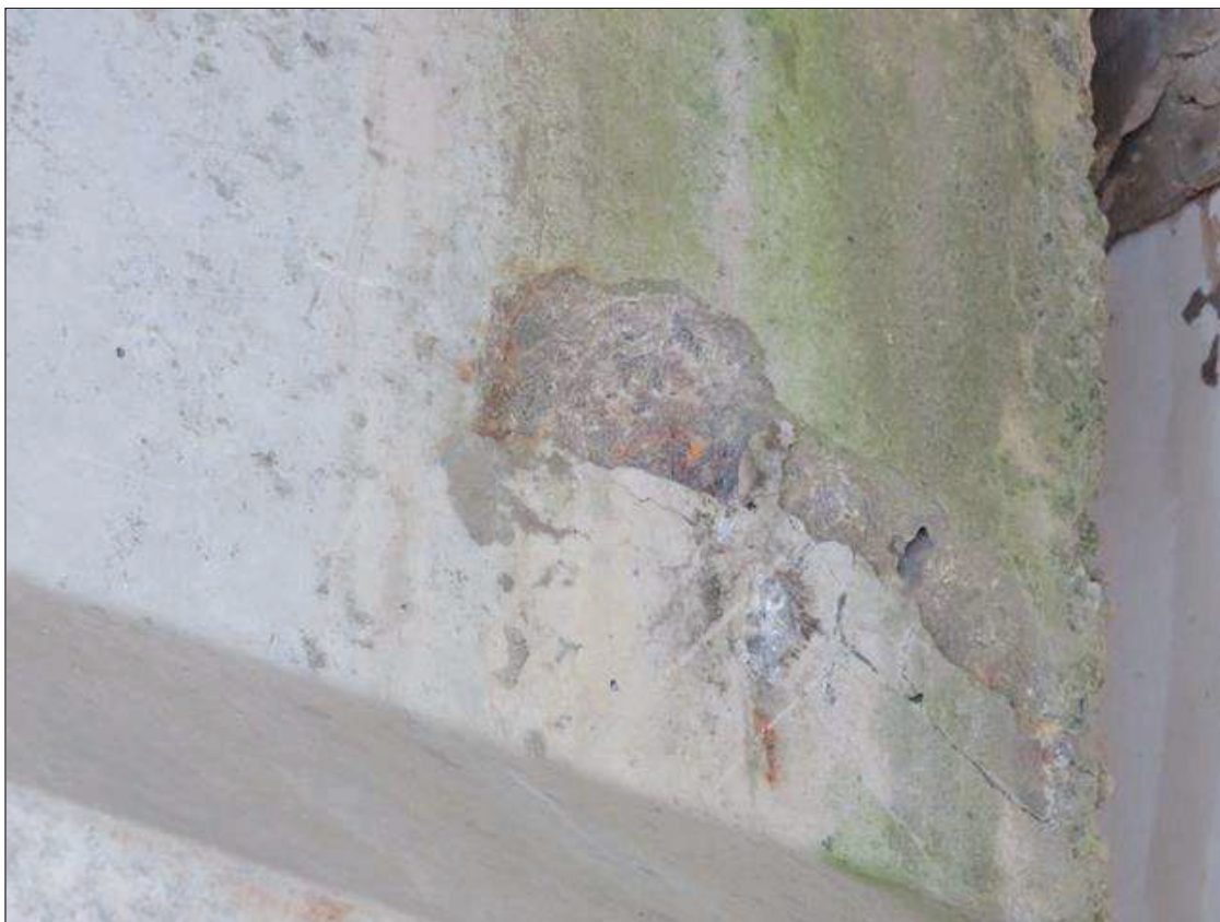
Span 2 Beam 3: GIRDER END AT BENT 1, LEFT SIDE OF THE WEB, MAP CRACKING TO 1/16 INCHES WIDE WITH 9 INCHES LONG X 6 INCHES HIGH X 1/2 INCH DEEP SPALL WITH ADJACENT DELAMINATION
