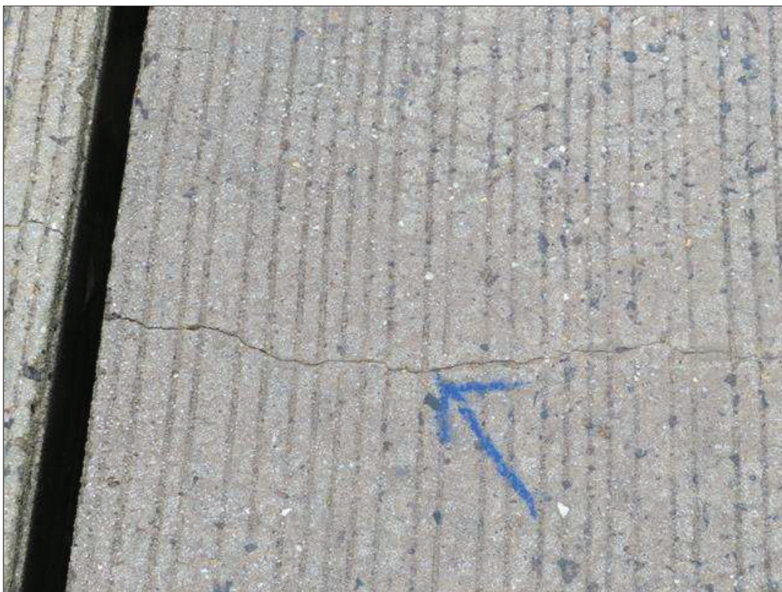
Span 2 Deck: 3 SQUARE FEET HAIRLINE LONGITUDINAL CRACKS EXTENDING FROM BENT 2 JOINT
