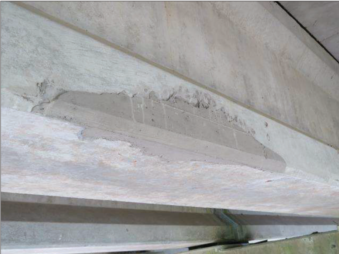
Span 4 Beam 2: PATCH AREA, FORMERLY 3 FEET LONG X UP TO 5 INCHES HIGH X 3 INCHES DEEP SPALL WITH EXPOSED STRAND, WEST FACE, 8 FEET FROM BENT 3
