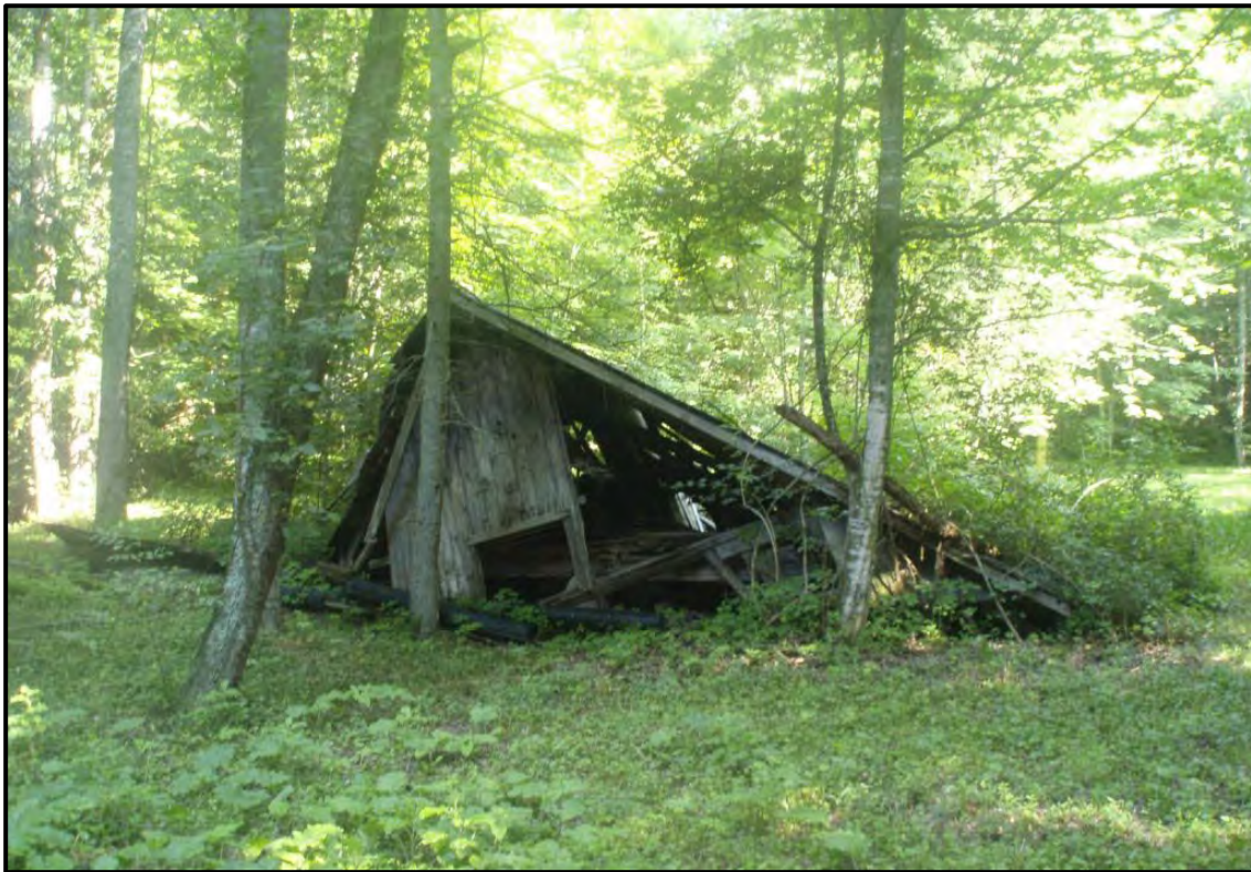
Figure 27: Northwest view of collapsed structure at 31WT371**.
