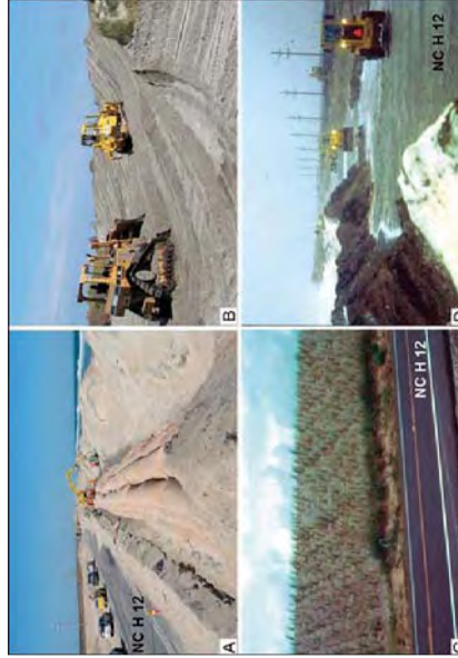
Figure 17. Photographs show the modern rebuilding of constructed barrier dune ridges to protect Highway 12 (A-C). (A) Recently adopted practice of building a sandbag core buried in the dune ridge. Because the constructed dune ridges are out of equilibrium with natural beach dynamics, the beach becomes increasingly steeper and narrower, resulting in more frequent storm surges eroding and overtopping the constructed dune ridge and jeopardizing Highway 12 (D). Photos in A, B, and C are by S.R. Riggs; photo in D is from Pilkey and Thieler (1992).
