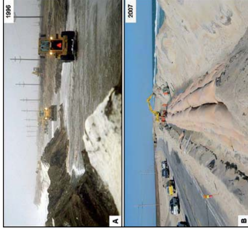
FIGURE 15. Panel A is a photograph that shows NC Highway 12 on Pea Island "gone-to-sea" in a 1996 storm. Panel B shows the late 2007 effort to anchor the constructed barrier dune ridge along NC Highway 12 with an internal core of sand bags. Panel A photograph is from Pileky and Thaler (1992). Panel B photograph is by D. Stewart, Pea Island Wildlife Refuge.
