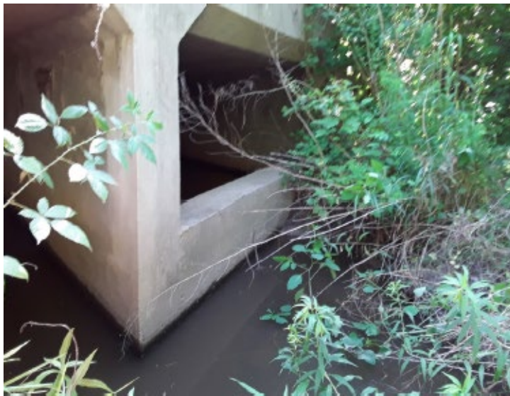
Image 3. Site 1 - 10' X 6' RCBC inlet looking downstream with 2-foot sill
