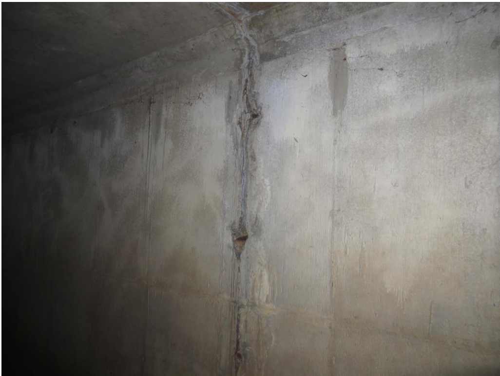
Cracking in Right Barrel
