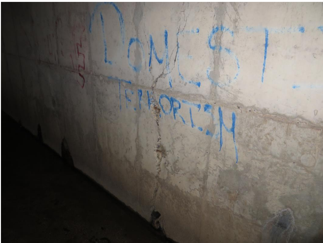
Cracking in Culvert
