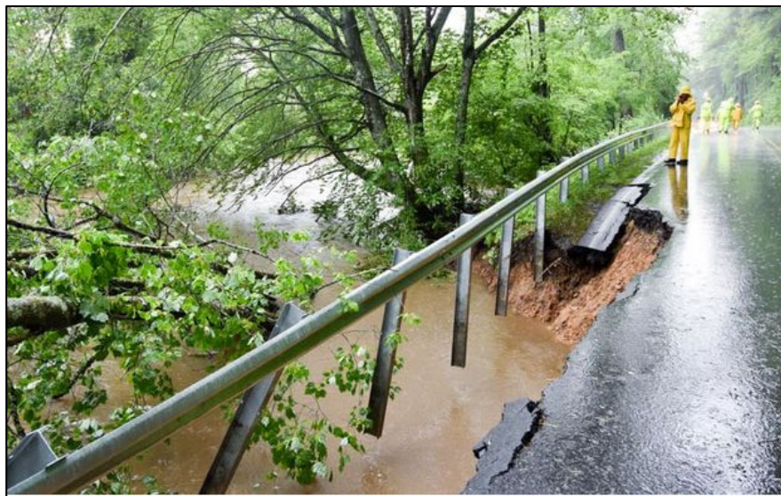
Exhibit 3. Wilson Road, between US 276 and Elm Bend Road, collapses after heavy rains May 2018 ( Transylvania Times ).
