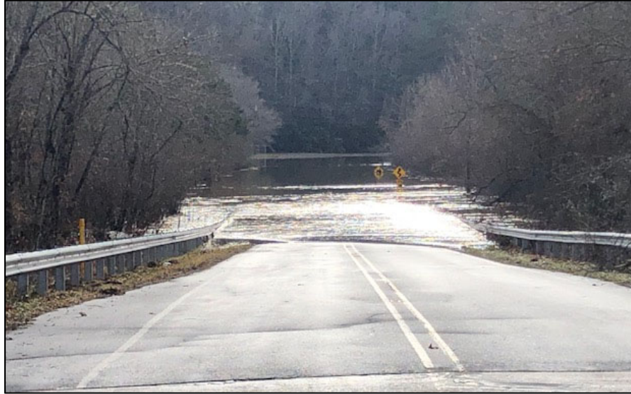
Exhibit 2. Wilson Road closure at the bridge abutment (facing south) due to flooding December 2018 (NCDOT).
