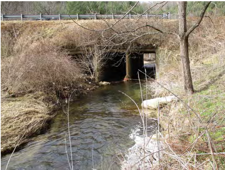
Site 2 – Brushy Fork Creek at US 321 / US 421; upstream face. Note sediment filled barrel at left.
