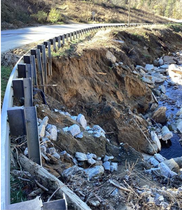
Eroded bank along Grassy Creek looking downstream (11/12/2024).
