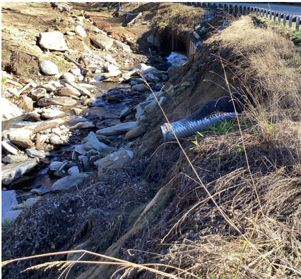
Eroded bank along Grassy Creek looking upstream (11/12/2024).
