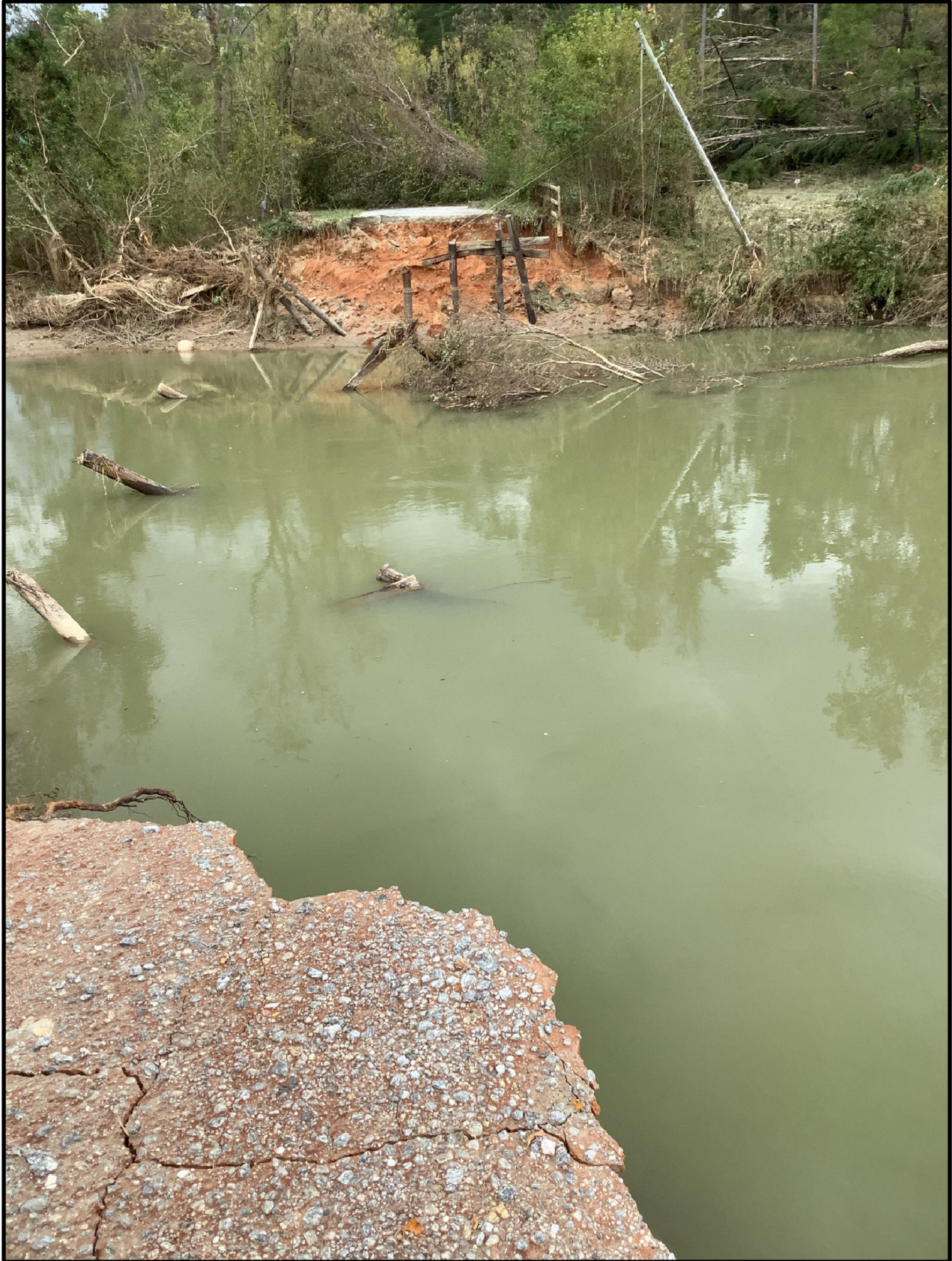
Figure 3. Detail of Bridge No. 0109 on SR 1578, Townsend Road, showing complete loss of the bridge from flooding (Helene 2024).
