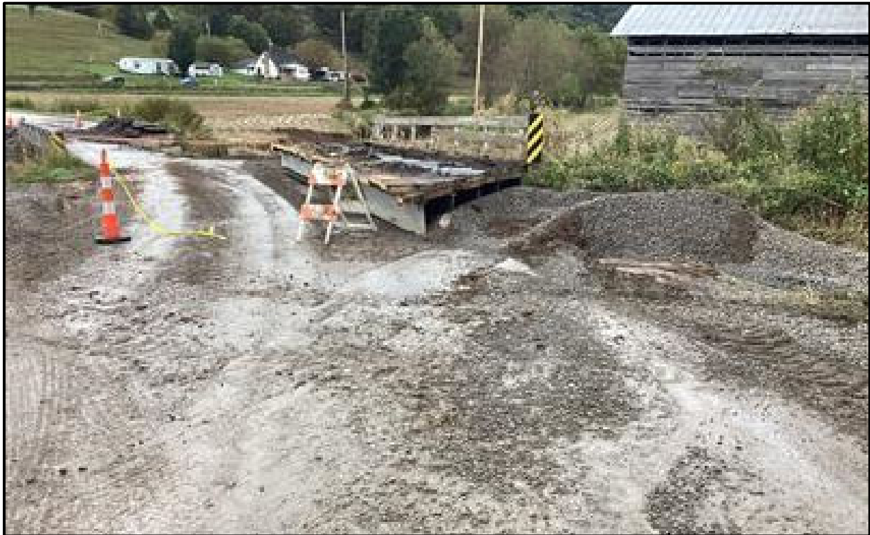
Figure 7. General View of damaged bridge and debris along with material being kept in the northeast quadrant after Hurricane Helene.
