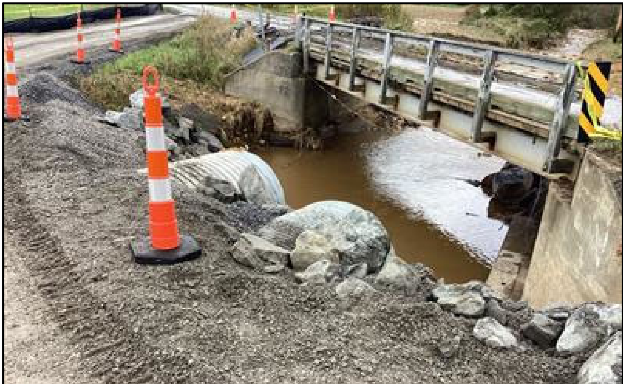
Figure 6. General View of the temporary crossing/detour south of the damaged bridge.
