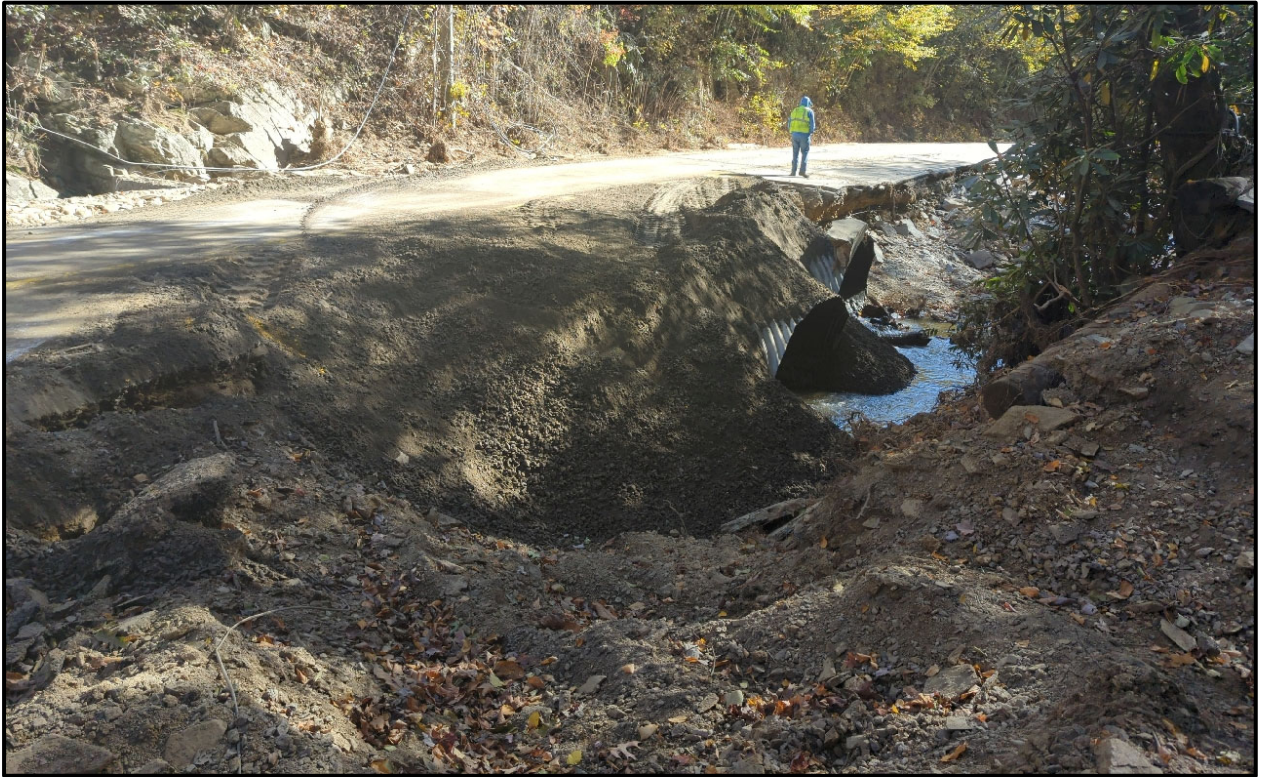
Figure 3. Hurricane Helene damage to Bridge No. 846 and landforms along Chestnut Hill Road.
