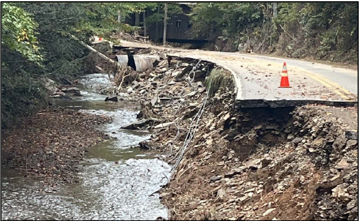
Figure 4. Hurricane Helene damage to Bridge No. 846 and landforms along Chestnut Hill Road.
