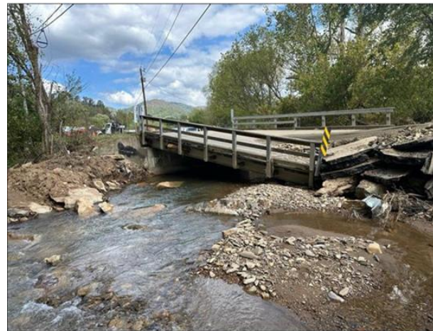
(PAR) bridge failure at end bent 1 north end
