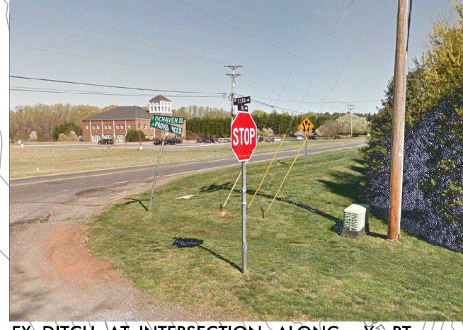
EX DITCH AT INTERSECTION ALONG -Y- RT. NO DEFINED DITCH AROUND CURVE TO TIE INTO OUTFALL
