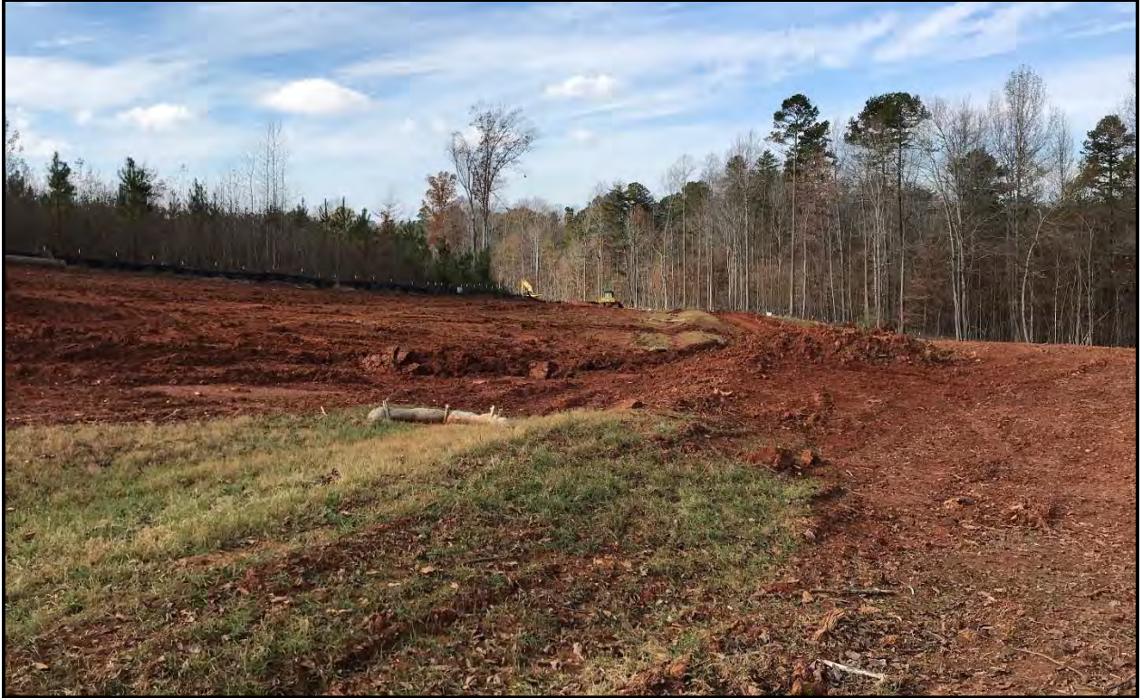
Figure 7. General View of construction activities relating to the Collins Ridge Development project adjacent to U-5848, looking west.
