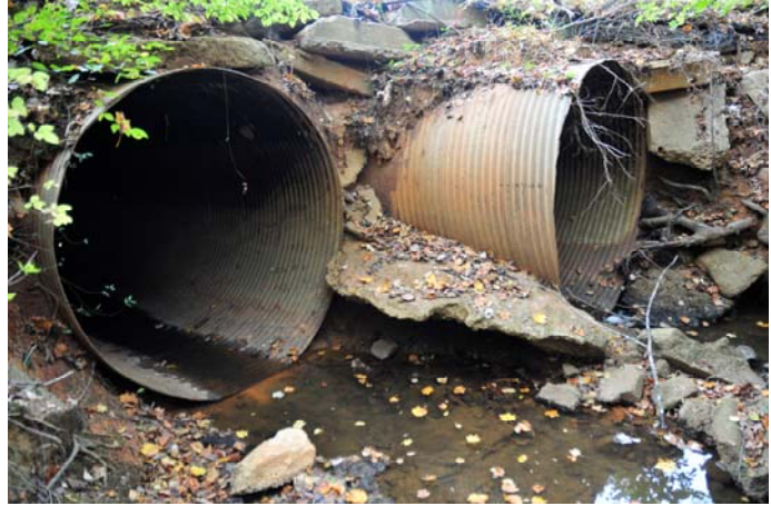
Deteriorating pipes carrying Williams Creek under Lake Pine Drive
