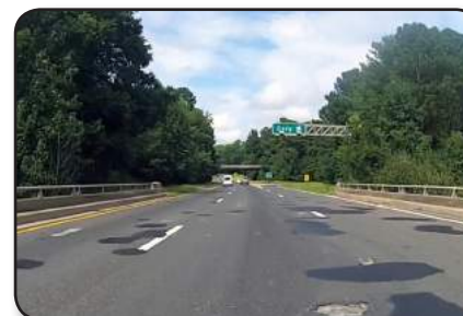
Rough pavement on I-440 near Western Boulevard
