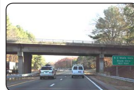
Melbourne Road bridge - rated structurally deficient
