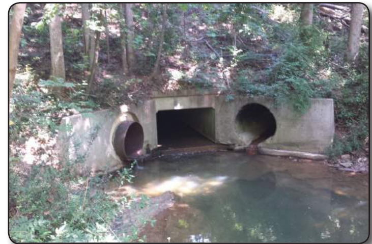
Outfall of existing drainage system into Brushy Creek at Western Boulevard interchange
