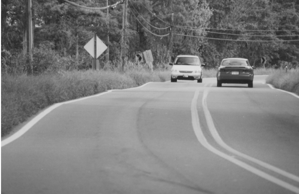
Figure II-1 Differential settling has caused damage to the roadway in the past.
