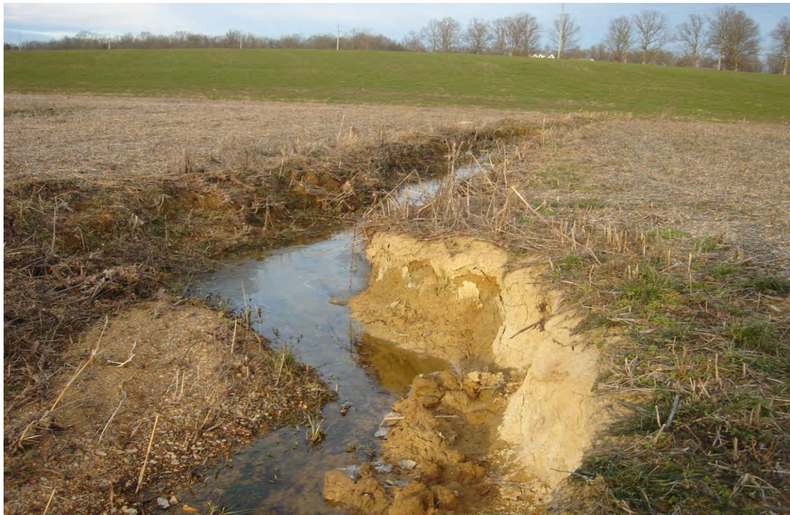
Photo 6: View of southwestern tributary exhibiting severe bank erosion and non-existent riparian buffer within Site 3.
