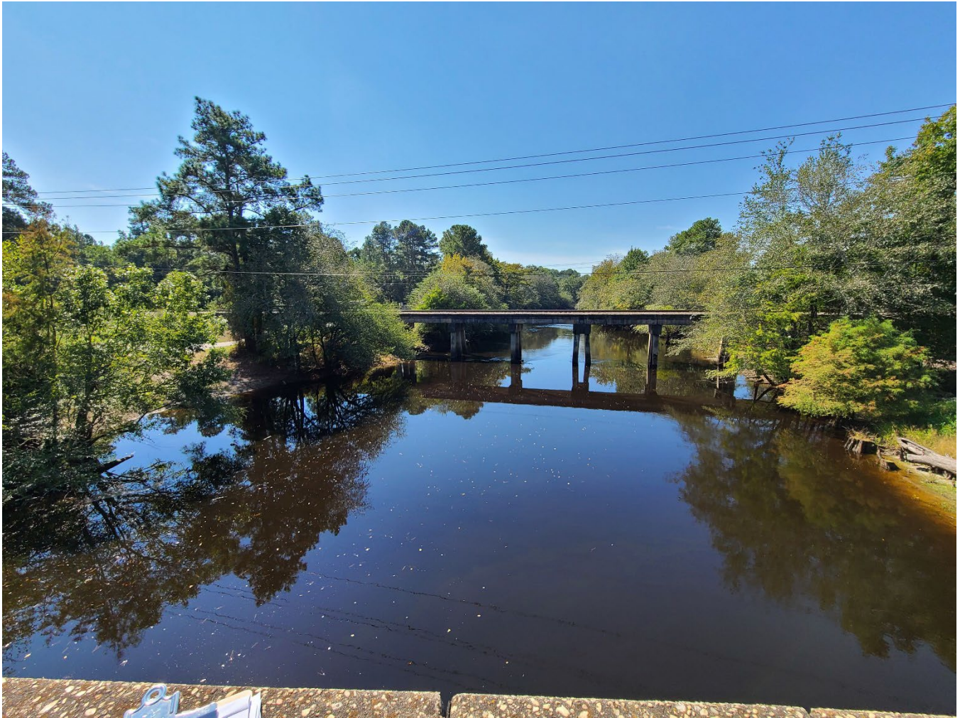
Figure E – Downstream view of the Lumber River corridor from the NC-41/NC-72 bridge sidewalk
