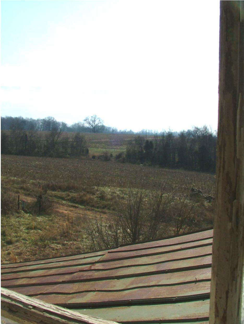
Plate 18: Looking southwest from second story of McKee House across porch roof; junction of I-40 and I-77 in distance obscured by elevation of land
