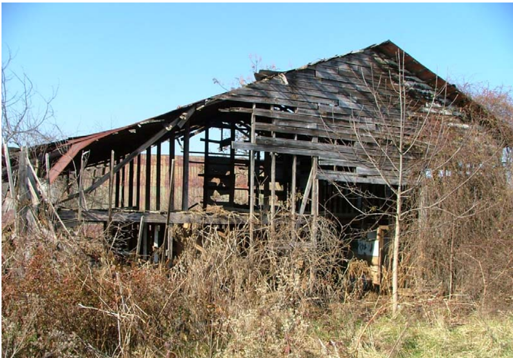
Plate 13: Looking west at ruinous livestock barn to west of McKee House
