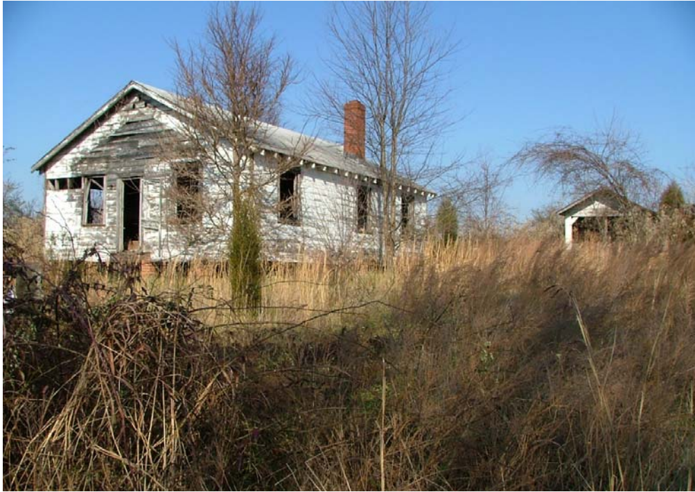
Plate 8: Looking northwest at deteriorated twentieth-century house and garage to east of McKee House
