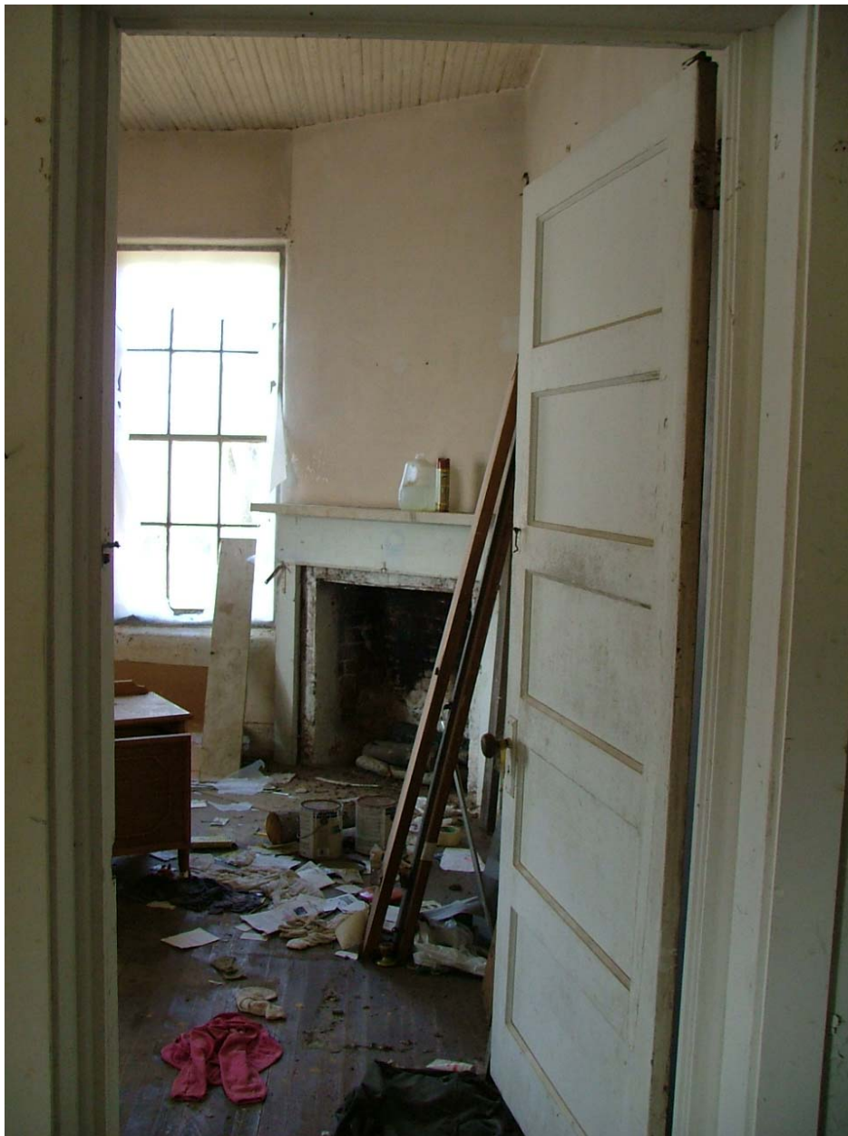
Plate 5: Southeast downstairs front room of McKee House from principal room; note corner hearth and twentieth-century door, mantel, and woodwork
