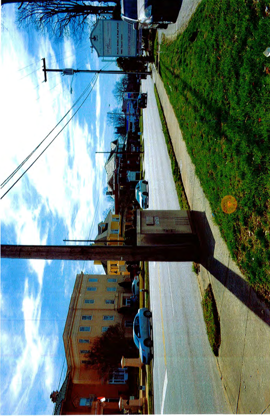
Upgraded Signal Box located Southeast Corner of Main St. and Farris Ave
