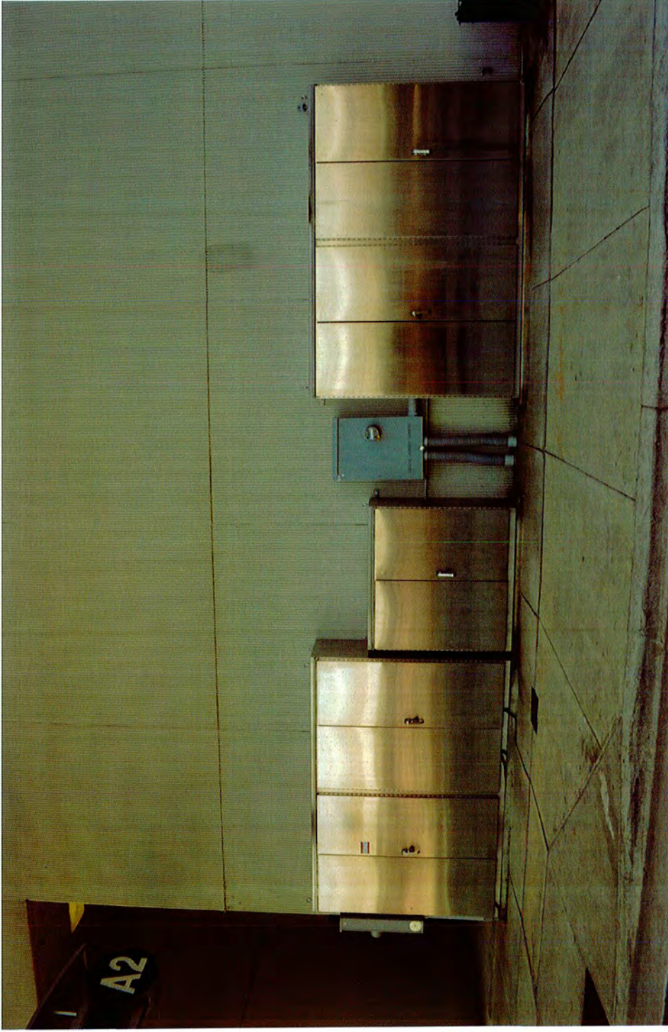
S. Wrenn St Location of Upgraded Signal Boxes
