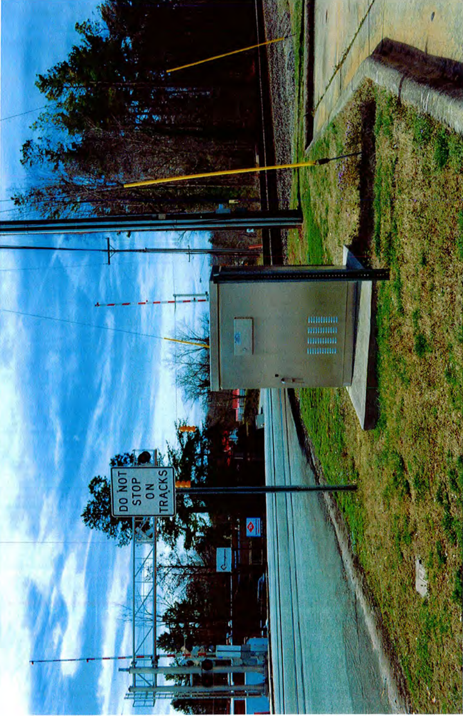
Upgraded Signal Box on Ragsdale Rd in the Quick Mart Parking Lot
