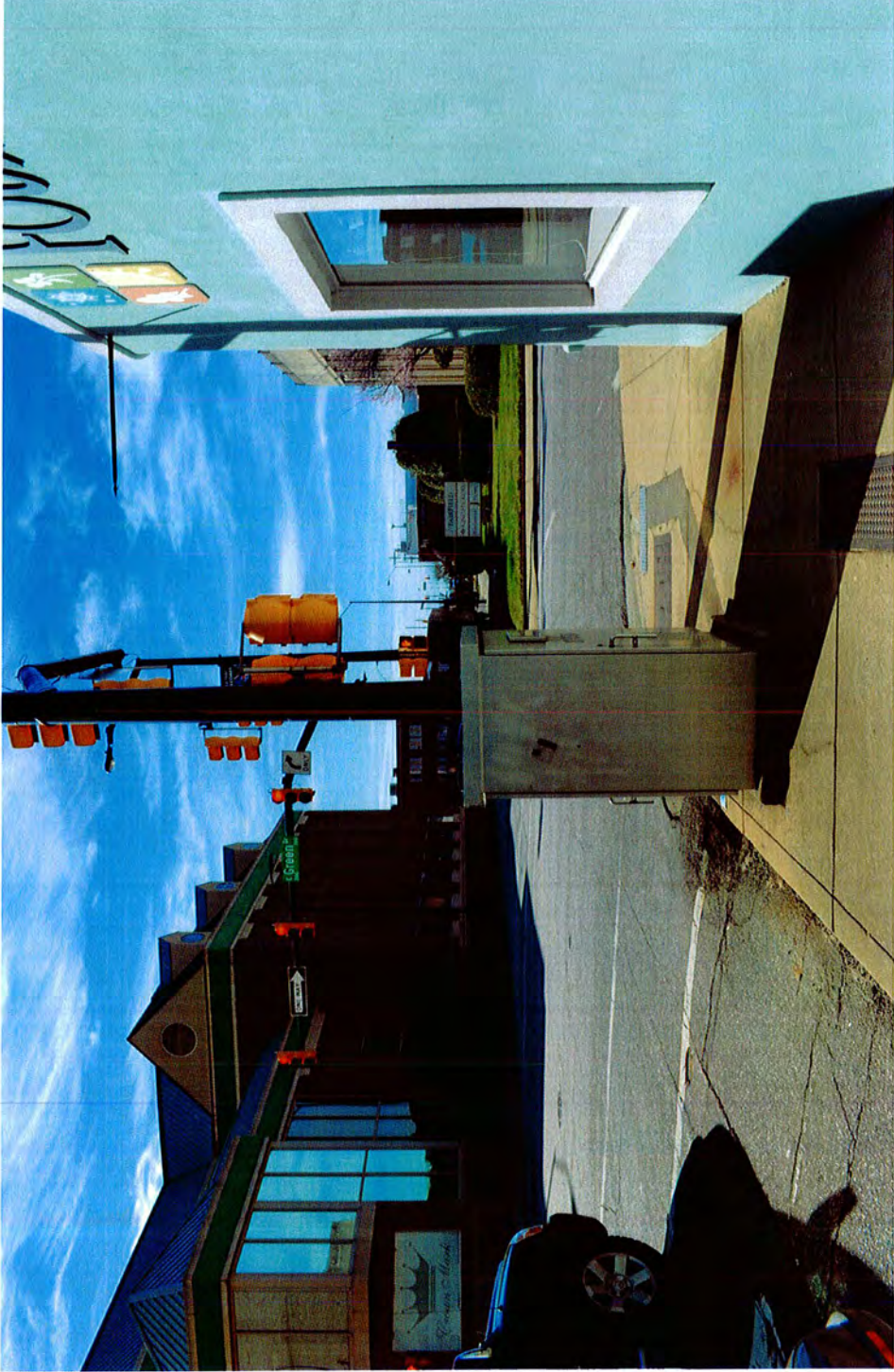
Green St. and Main St. Locations of Upgraded Signal Cabinets
