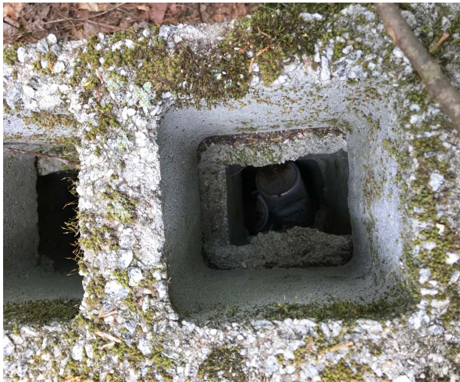
B) Cans Located Within the Block Wall
