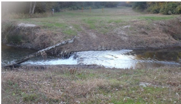
Photo 3. Perched Utility Crossing in East Braid of Swift Creek below NC 42
