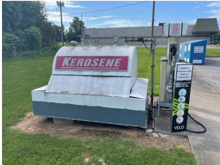
An approximately 500-gallon kerosene AST in the eastern area of the Project Study Area adjacent to the BP parking lot. Stressed vegetation and a slight petroleum odor were noted in the vicinity of the AST.
