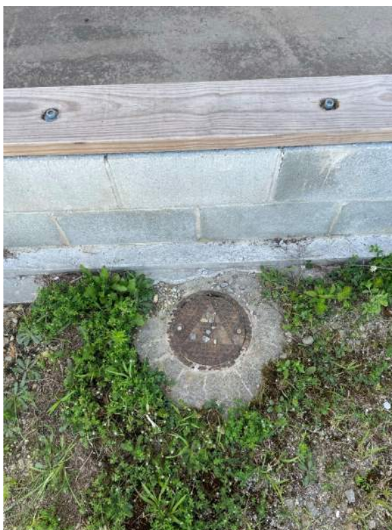
A groundwater monitoring well located outside of the northern edge of the concrete wall that bounds the area under the former fuel canopy, in the northern portion of the Project Study Area. Original in Color
