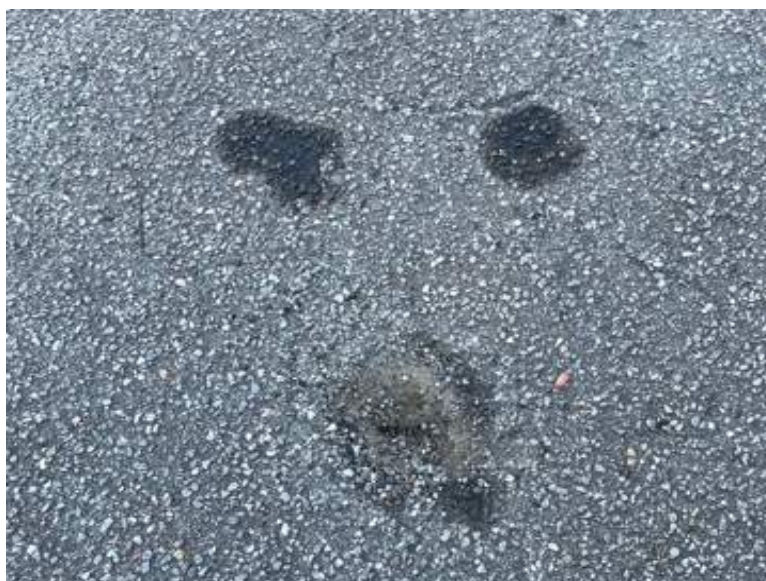
Petroleum surface staining in the eastern portion of the Project Study Area.
