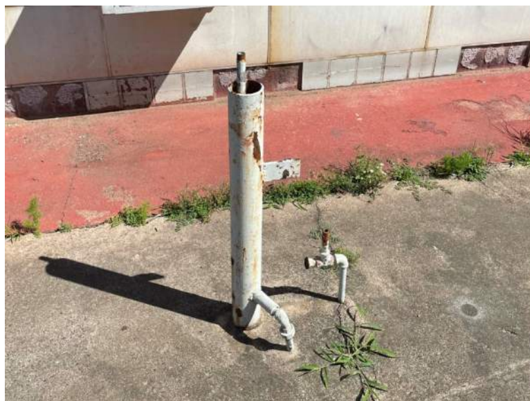
Inactive product pipe located along the southern side of the convenience store structure.
