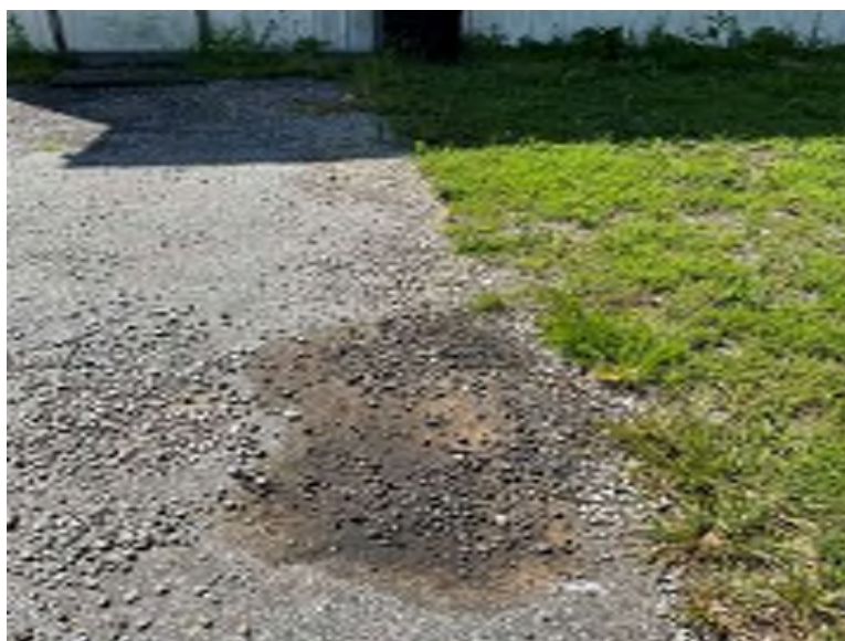
Surface staining in the northwestern portion of Parcel 73 west of the Project Study Area.
