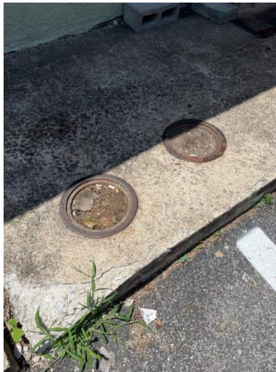
Former fuel ports associated with an inactive UST bed in front of the convenience store facing NC 115.
