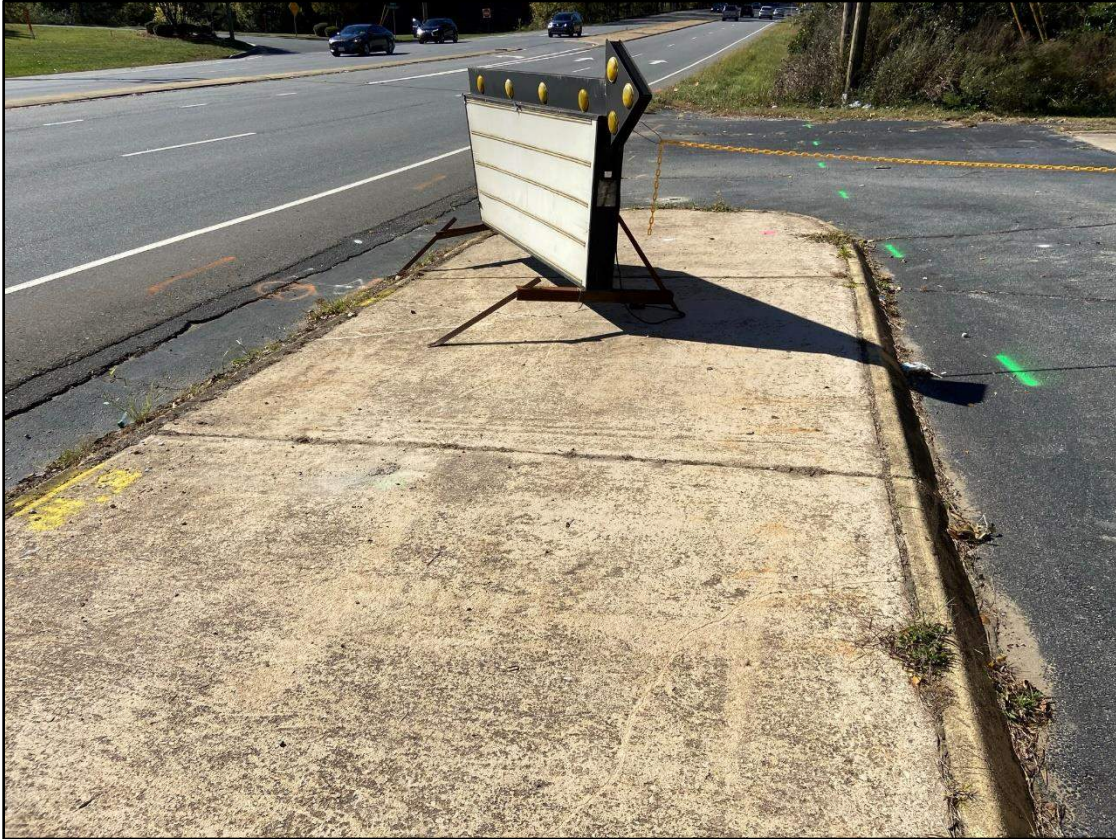
Photo 7: Condition of roadside island, looking west.
