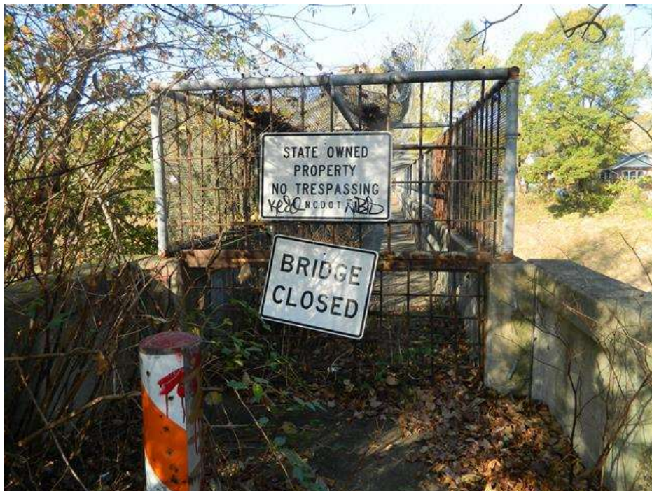
LOOKING NORTH (BRIDGE CLOSED, REBAR WELDED ACROSS APPROACH TO
