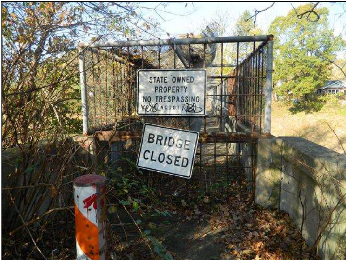
LOOKING NORTH (BRIDGE CLOSED, REBAR WELDED ACROSS APPROACH TO PREVENT PEDESTRAIN ENTRANCE TO STRUCTURE)
