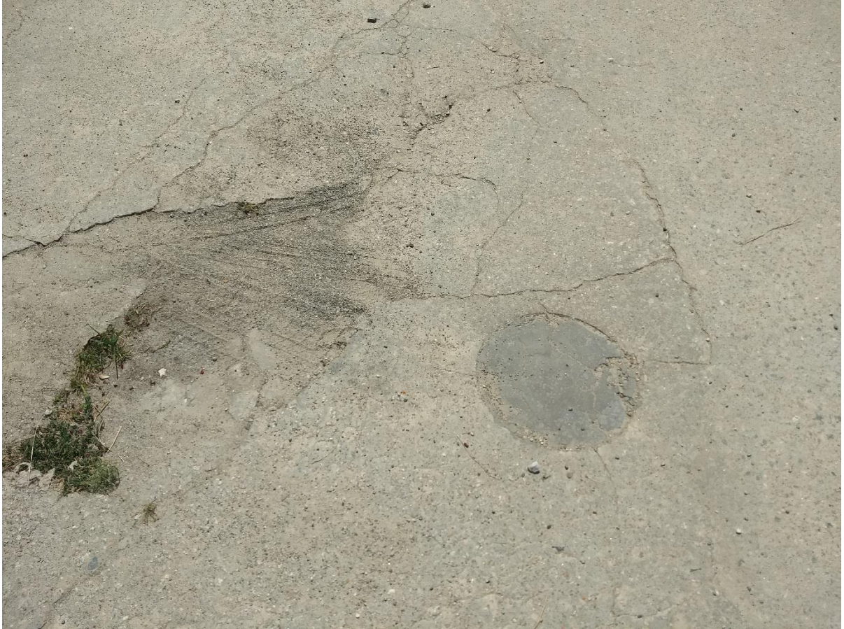
Monitoring well abandoned.
