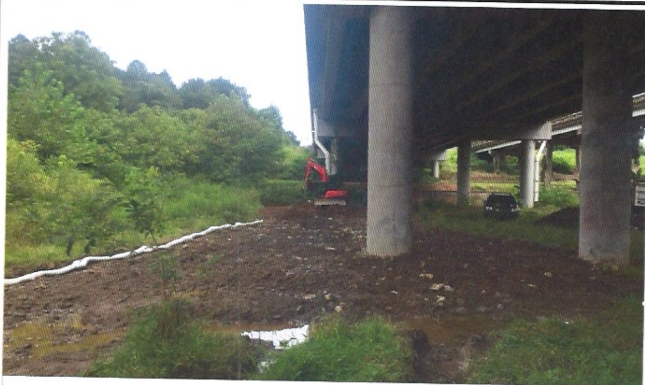
View of the spill site-looking north
