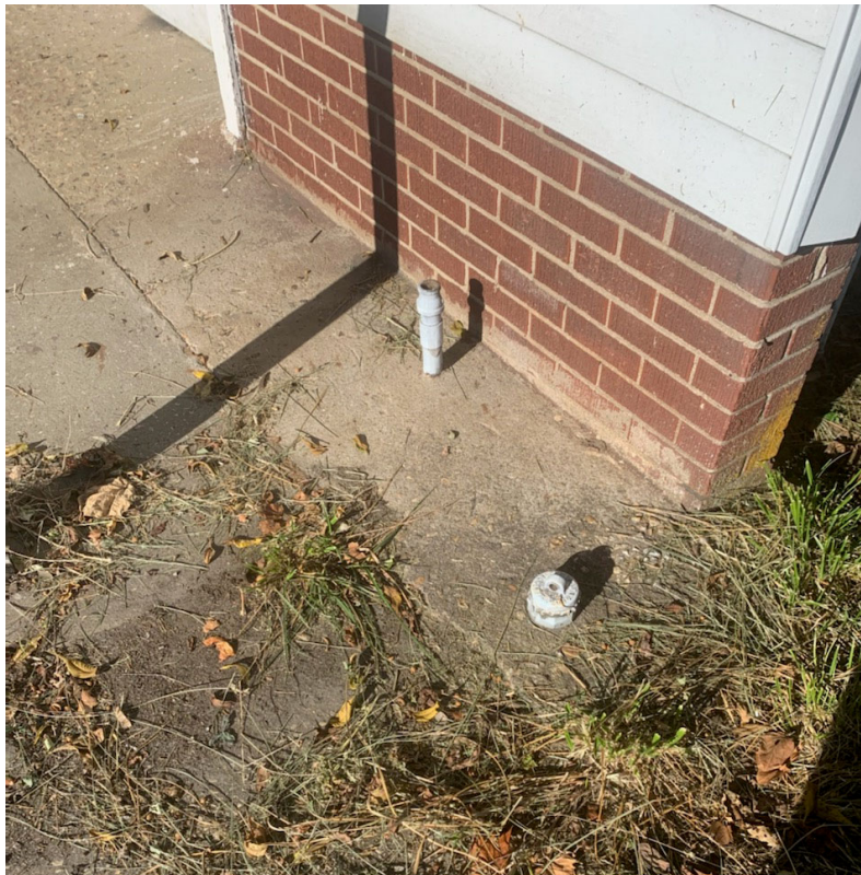
Photograph 2: View of potential fill port near UST #3.
