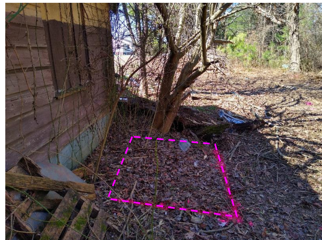
D. Photograph of approximate location of UST-1 located on the north end of the building, looking west.
