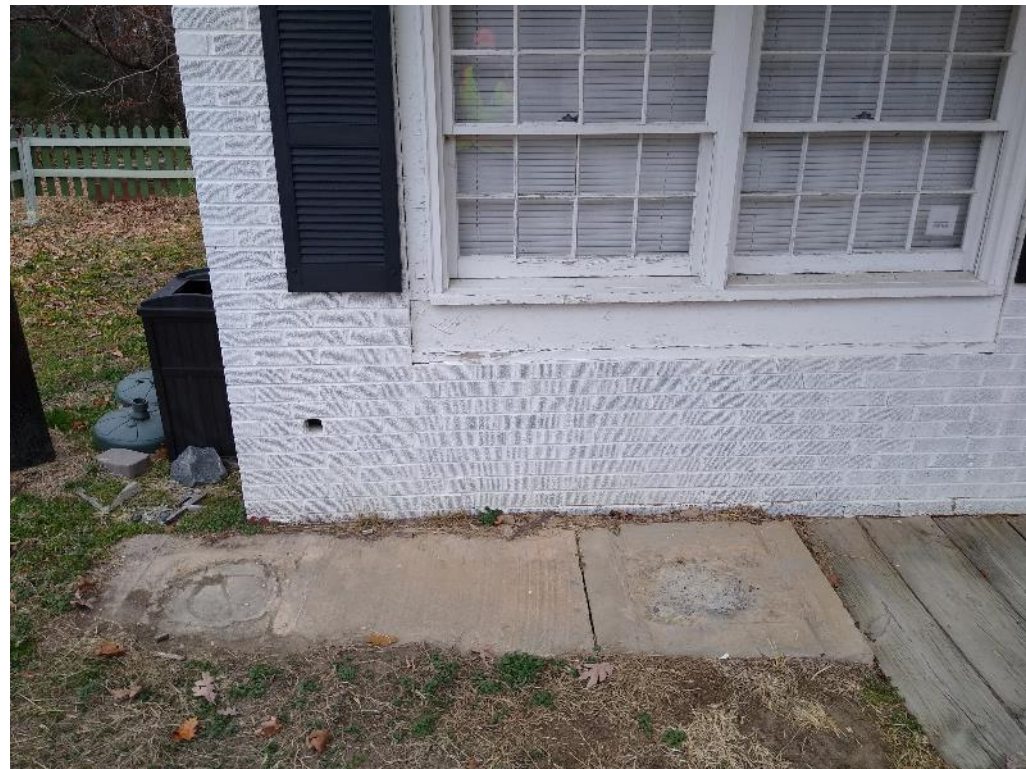
G. Photograph of probable former dispenser island for UST-3 and UST-4, looking north.
