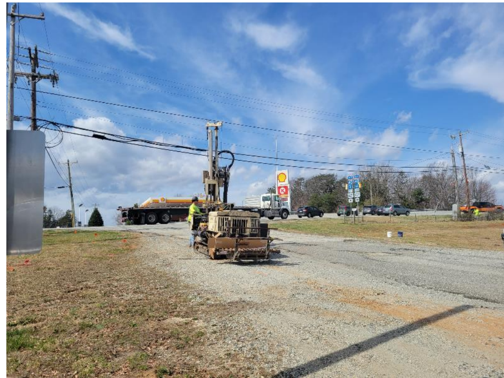
C. Photograph of drilling Boring B175-1 on west side of parcel, facing west.
