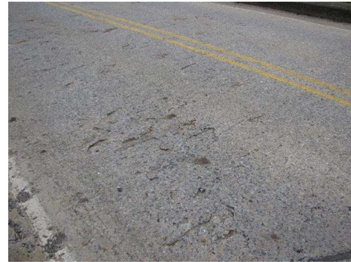
SPAN E CONDITION PHOTO FROM 2016 INSPECTION REPORT
