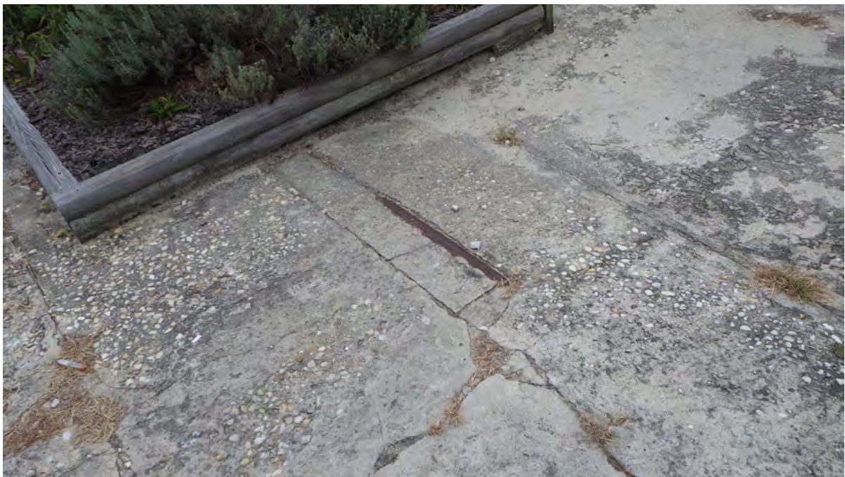
Possible abandoned product line/pipe.
