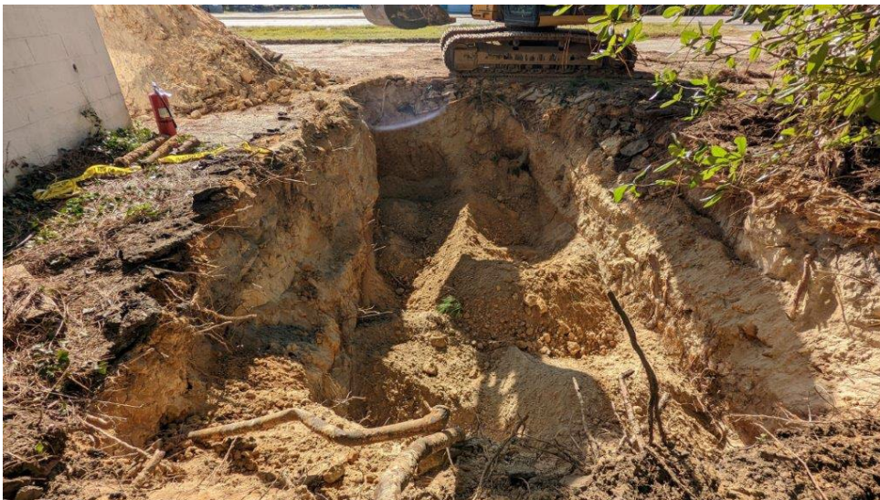
Photograph 4: Excavation following removal of USTs, vent pipes visible in bottom of photo.
