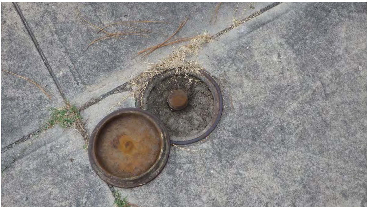
UST fill port uncovered.
