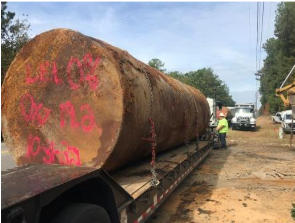
Photograph 8: Evo loading UST#3 on to trailer. UST in good condition, no pitting or holes.
