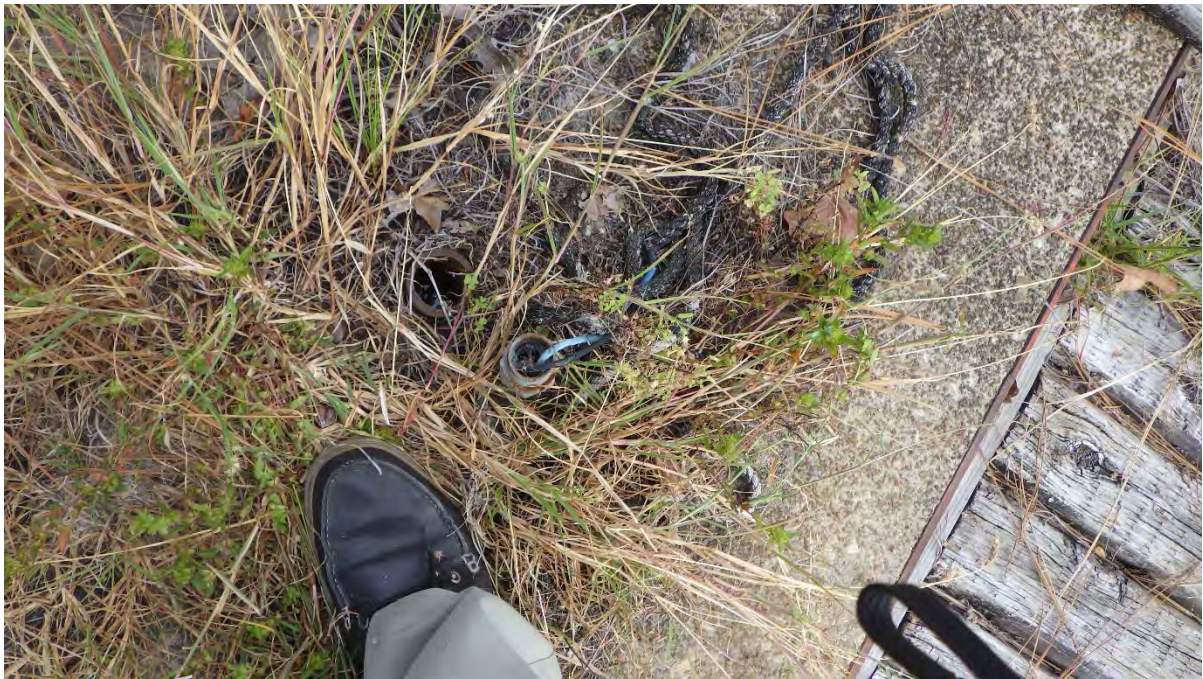
Possible abandoned UST product line/pipe
