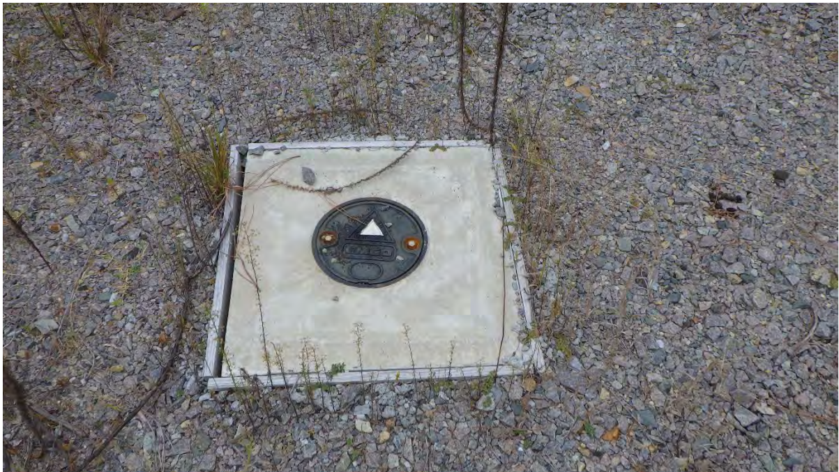
Recently installed monitoring well
