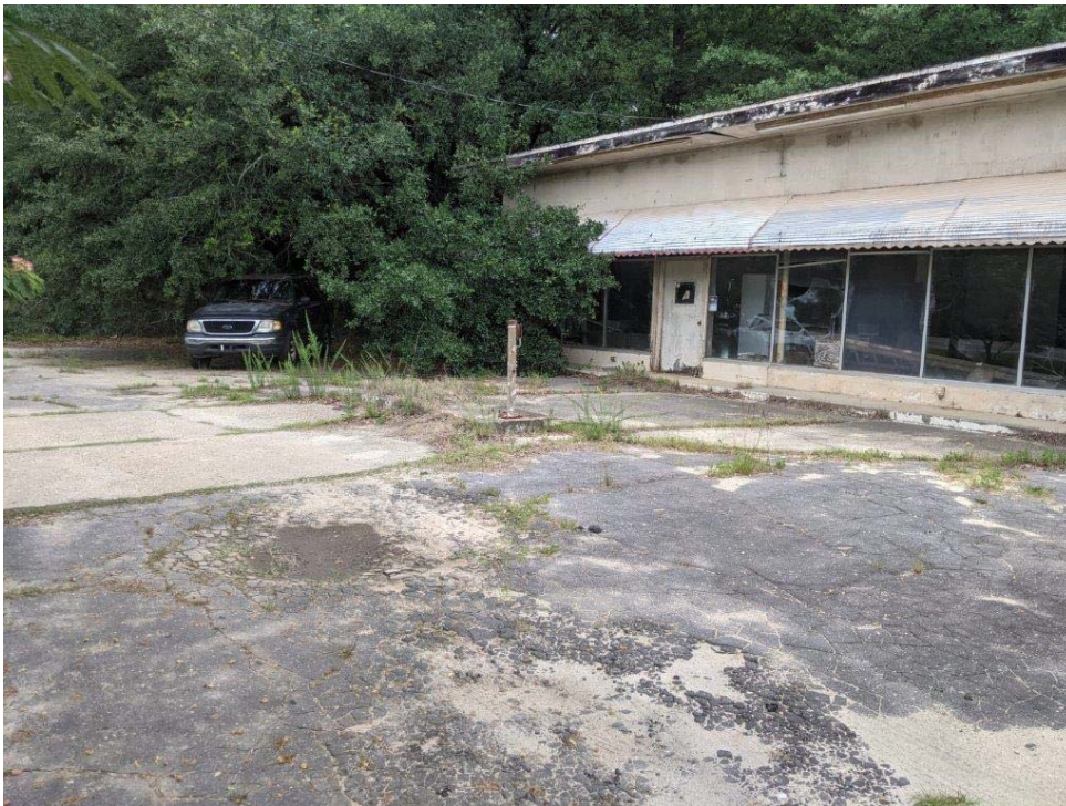
Photograph 2: Dilapidated building and suspected dispenser island at parcel 368, facing northeast.
