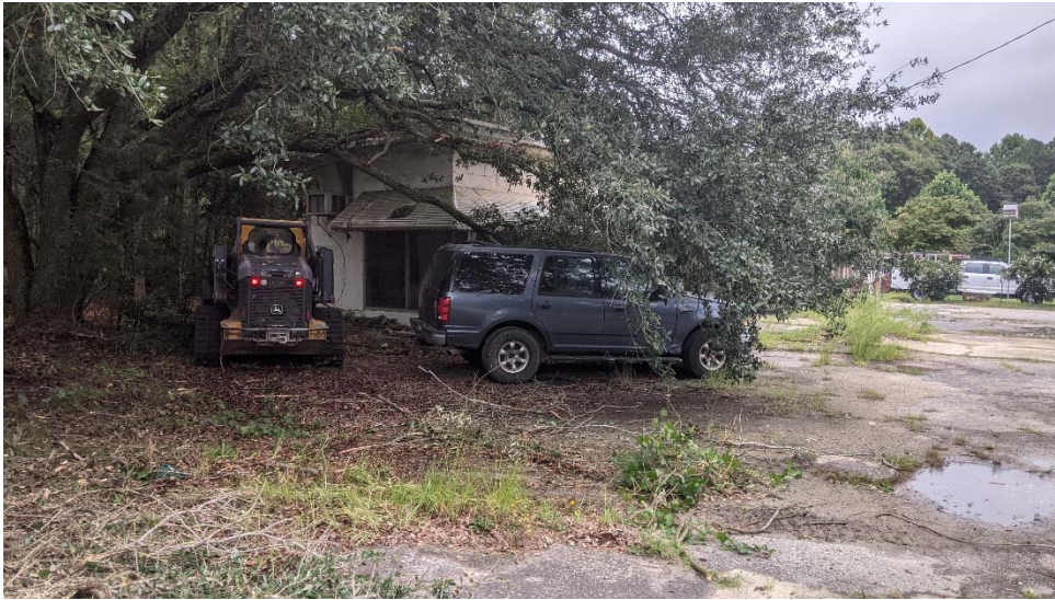
Photograph 5: Vegetation clearing to the west and northwest of dilapidated Site building, facing southeast.
