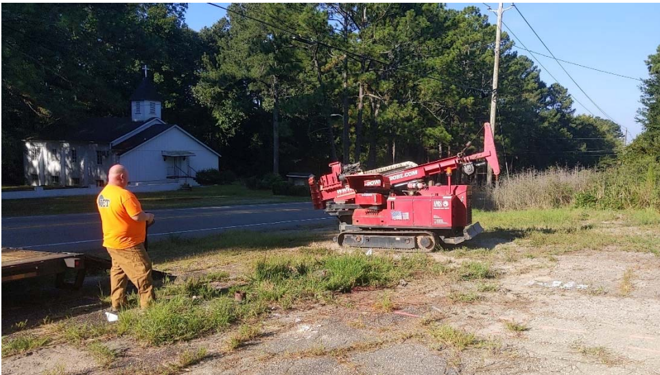
Photograph 4: View of IET maneuvering direct- push rig to collect soil samples, facing southwest.
