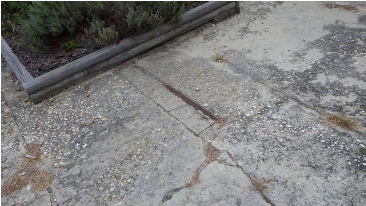
Possible abandoned product line/pipe.
