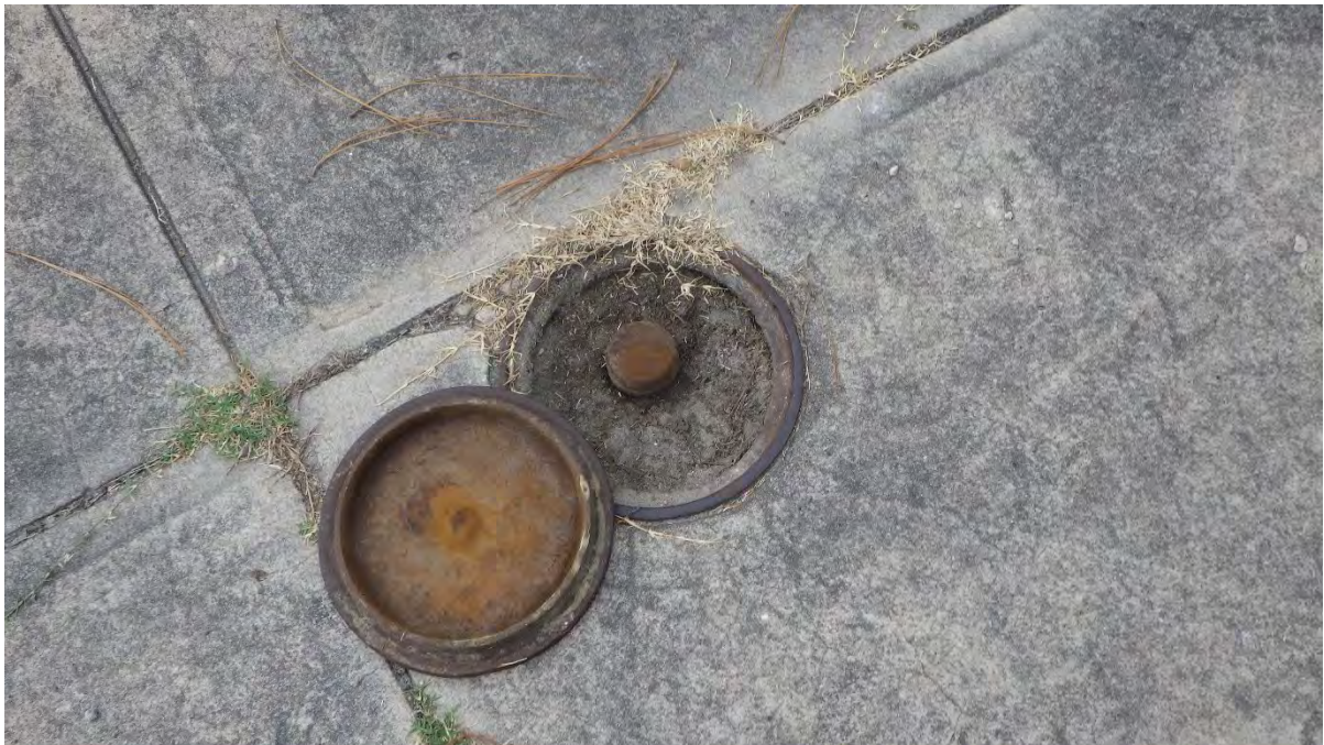
UST fill port uncovered.
