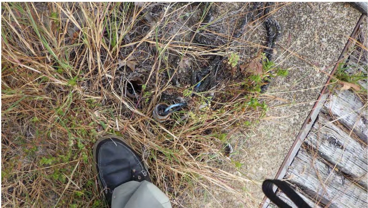
Possible abandoned UST product line/pipe
