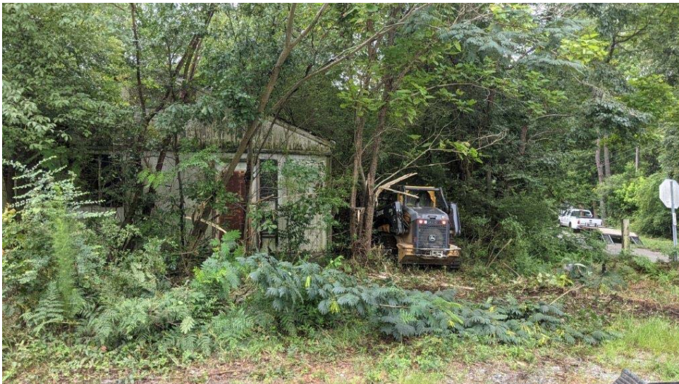
Photograph 2: Vegetation clearing around dilapidated building at the parcel, facing south.
