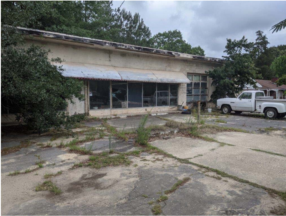
Photograph 1: Dilapidated building and suspected dispenser island at parcel 368, facing southeast.
