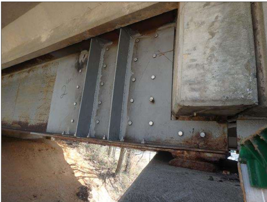
Span 4 Beam 1 at Bent 3, Temporary Repair to Section Loss, 1/4" thick plates bolted to both sides of web and bottom flange.
