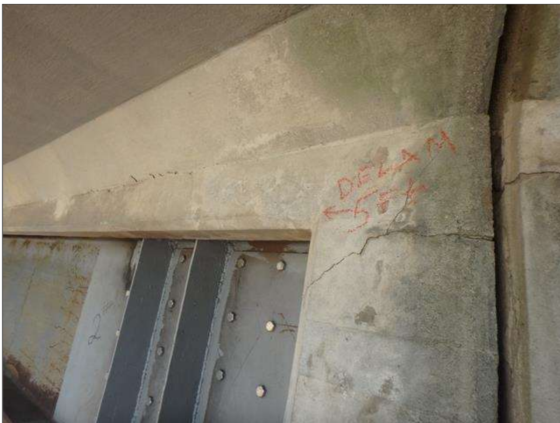
Span 4 RC Deck underside left overhang at Bent 3, Delamination in build up 5' long x 6" x 4".
