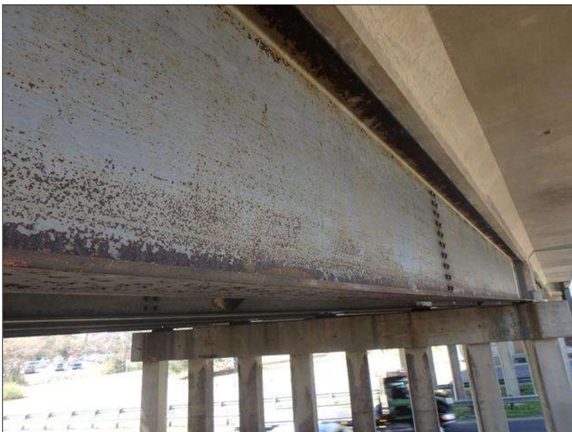
Span 4 Beam 1 Surface Corrosion and peeling paint along length of beam.
