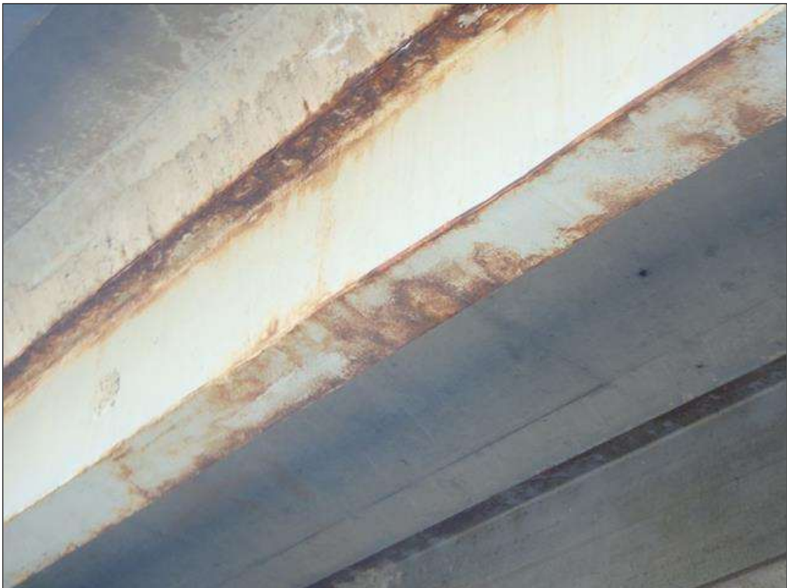
Span 2 Beam 1 above Right South bound lane, impact damage previously straightened/repaired.
