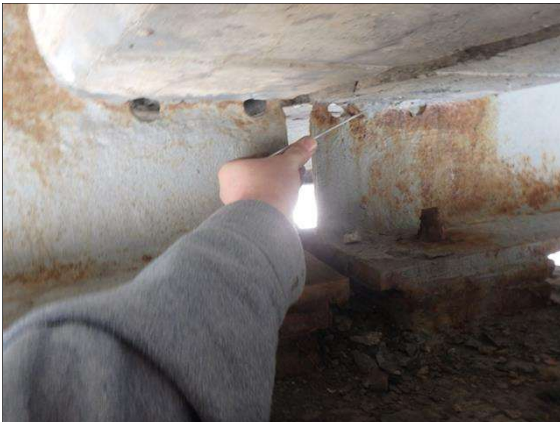
Spans 2 and 3 Beam 2 at Bent 2, end of beams below diaphragm has Section Loss, Surface Corrosion/Freckled Rust initiated since beam was cleaned and painted.
