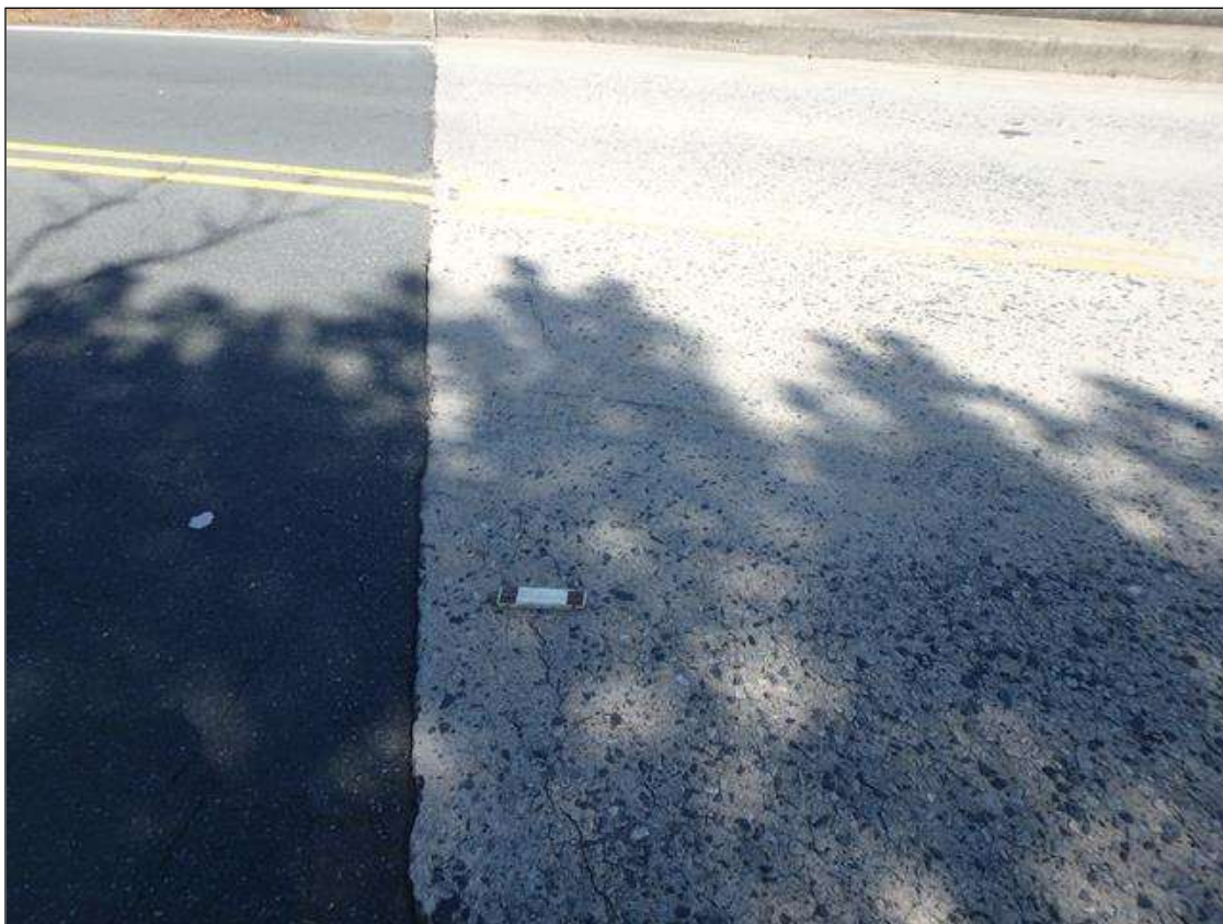
Span 1 RC Deck surface near End Bent 1 has transverse cracks 1/16" wide, abrasion/wear with coarse aggregate exposed and intact in the concrete.
