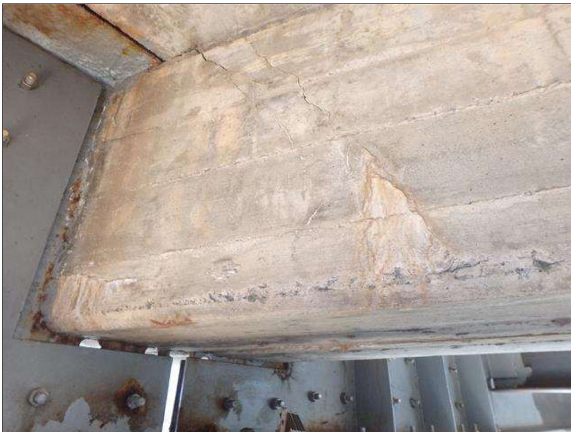
Span 4 RC intermediate diaphragm at Bent 3 in bay 4, Diagonal cracks up to 1/8" wide with efflorescence.
