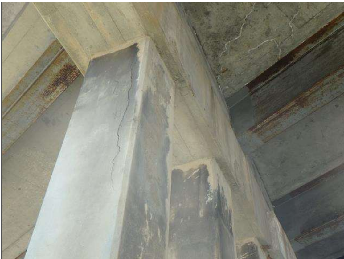
Bent 2 RC column 6 Southeast Corner vertical crack up to 3/16" wide with Delamination
