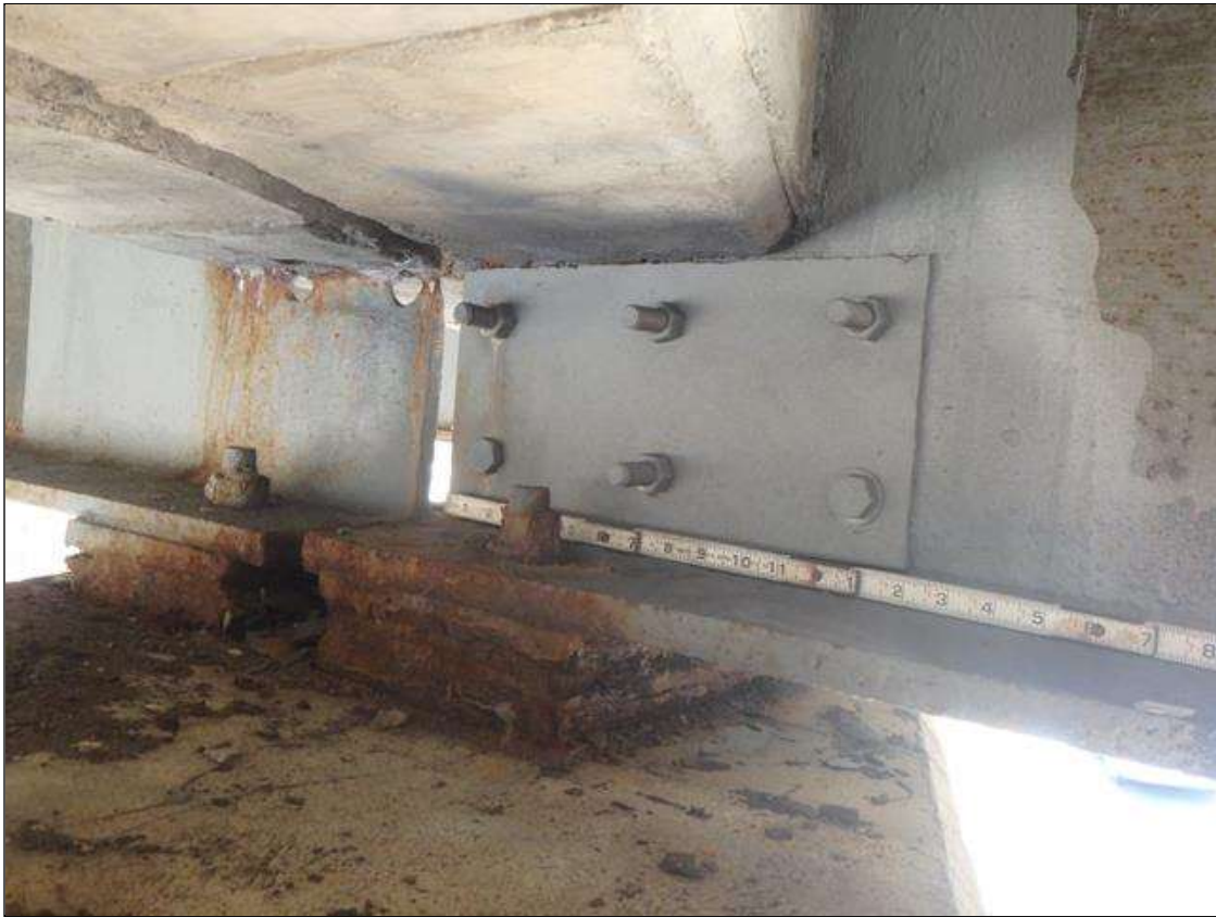
Span 2 Beam 4 at Bent 2, Temporary repair, 1/4" x 7" x 14" plates bolted to web at end of beam, both sides.
