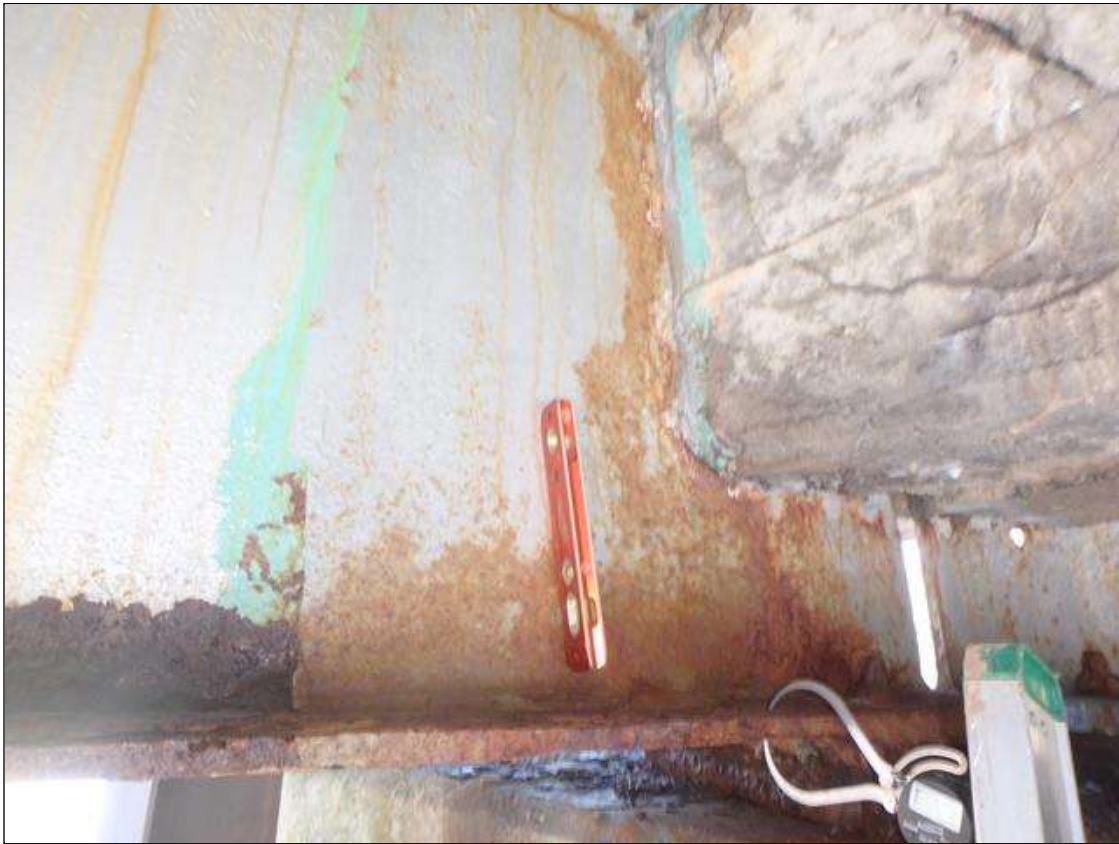
Span 2 Beam 1 at Bent 2, right side, Section Loss in web and bottom flange, Surface Corrosion/ Freckled Rust initiated since beam end was cleaned and painted.
