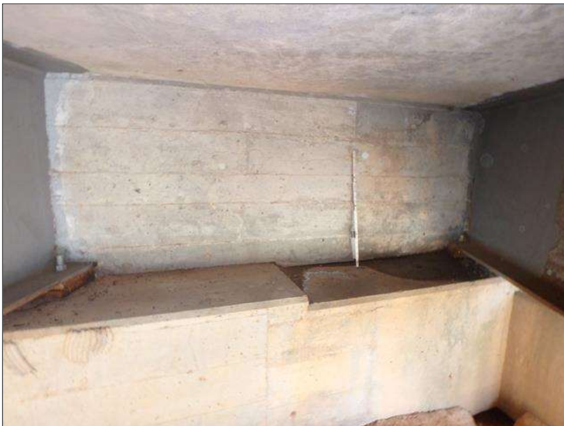
Abutment 2 in bay 4, 1/32" cracks.
