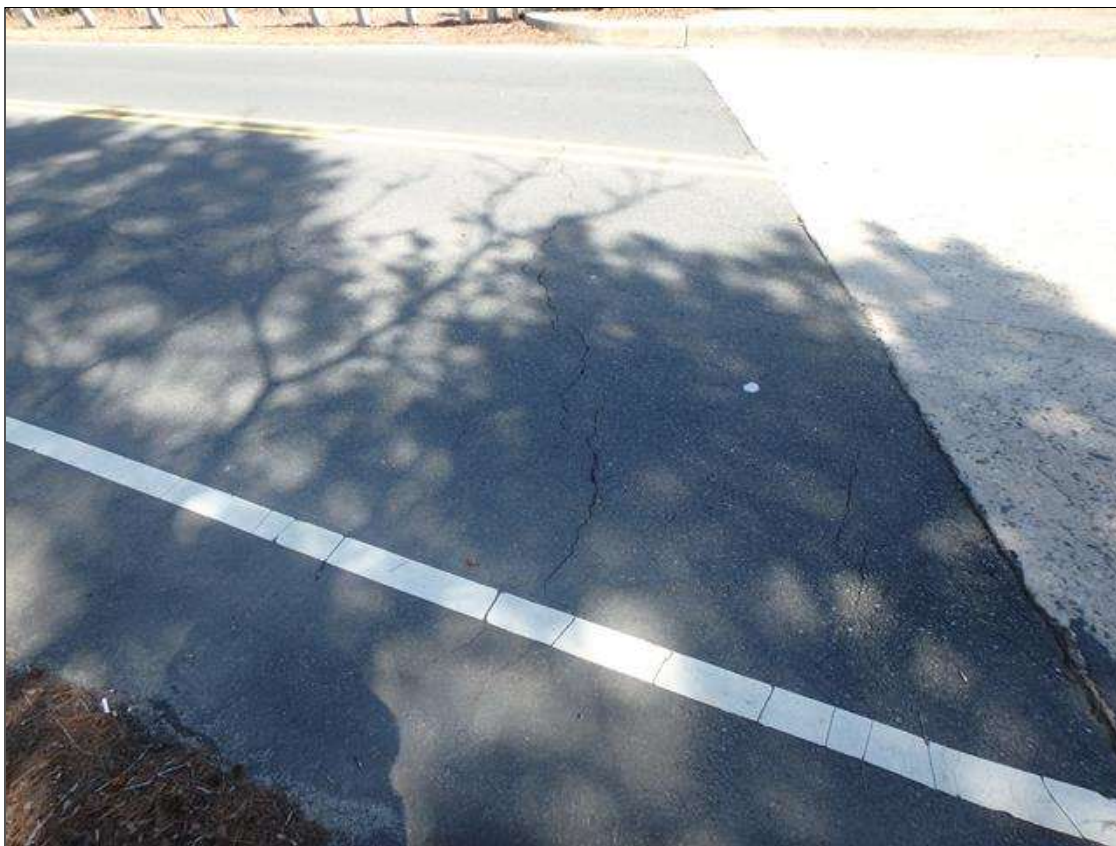
West Approach pavement at bridge has transverse cracks up to 1/8" wide, full width of roadway.
