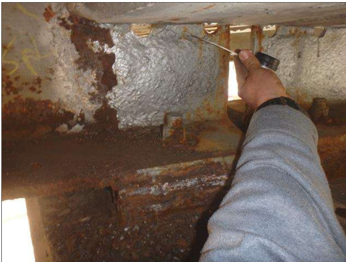
Spans 3 and 4 Beam 3 at Bent 3, end of beams Section Loss in the web below diaphragm, Freckled Rust initiated since beam was painted.
