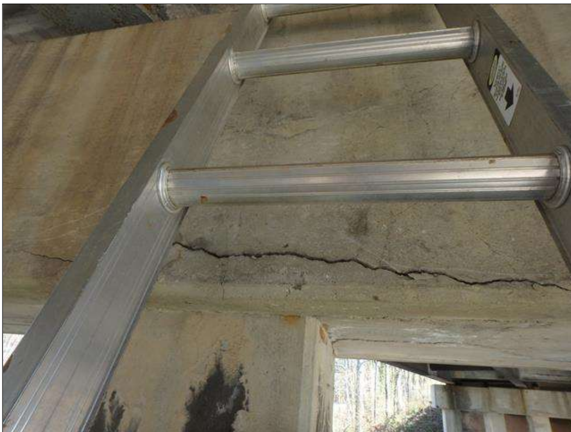
Bent 2 Cap west side bottom corner from column 3 to 4, 1/8" longitudinal crack and Delamination.
