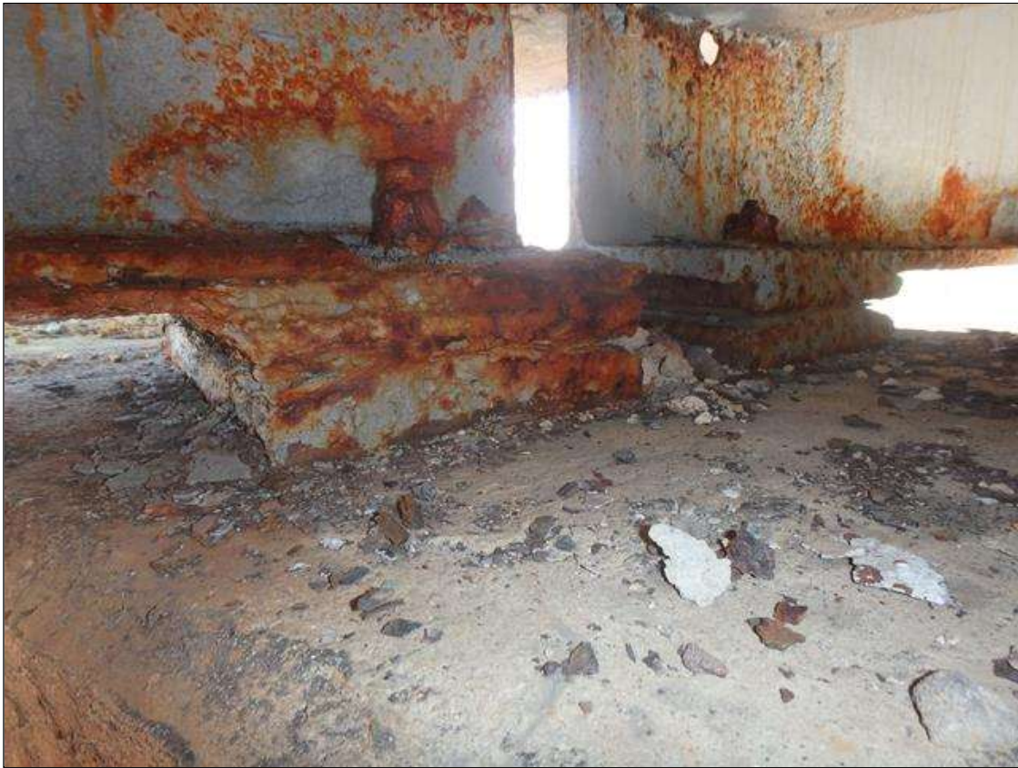
Spans 1 & 2 Bearing Assembly seat 1 at Bent 1, Active Corrosion & Section Loss <25% in the plates, fasteners 1/4" Remaining.
