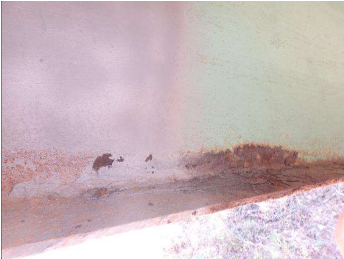
PRIORITY MAINTENANCE: Span 1 Beam 5 at 3' from end of beam at Bent 1, left bottom flange has Active Corrosion and Section Loss.
