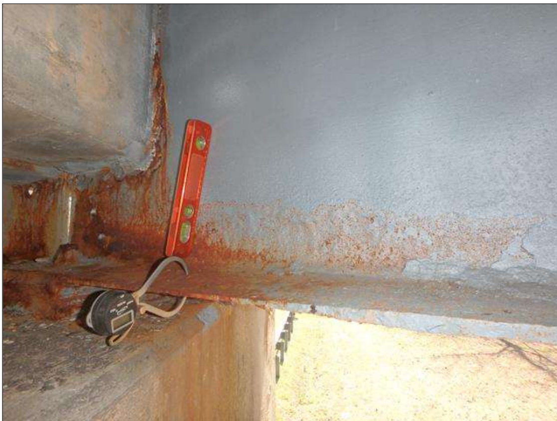
Span 1 Beam 5 at Bent 1, left side, Section Loss in bottom flange and lower web, Surface Corrosion/ Freckled Rust initiated since beam cleaned and painted.
