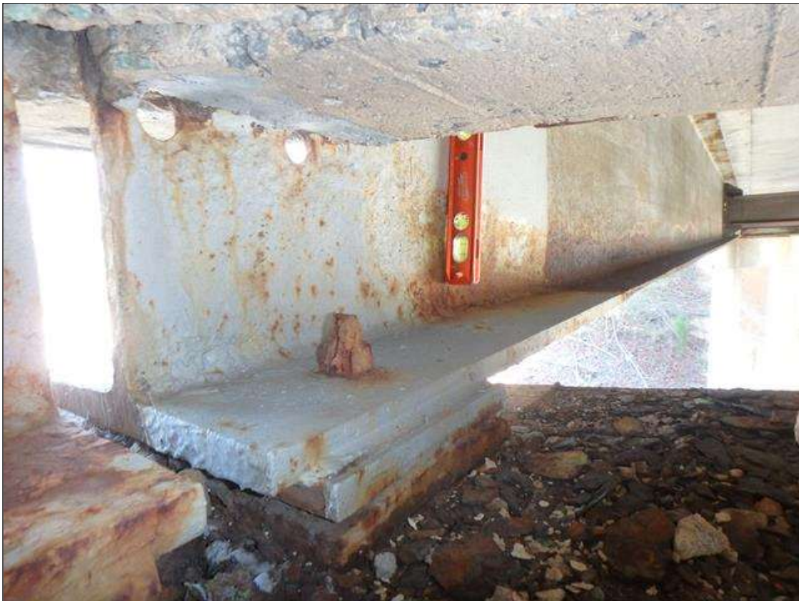
Span 3 Beam 1 at Bent 2, Section Loss in web below diaphragm, Section Loss in lower web along bottom flange.
