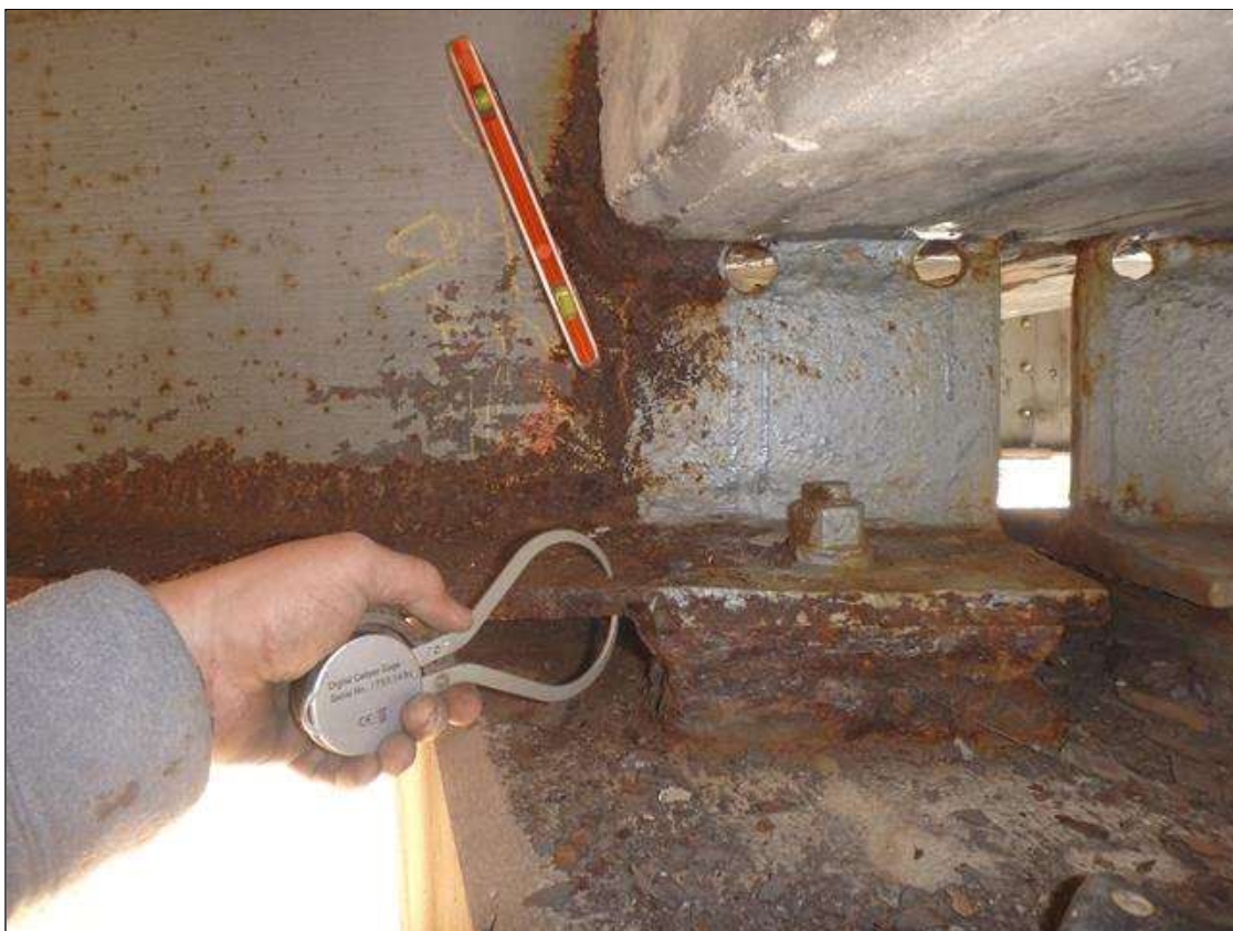
Span 4 Beam 4 at Bent 3 Section Loss in the web below diaphragm and in bottom flange in front of bearing.
