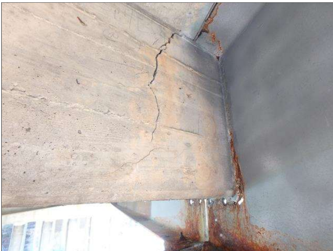
Span 1 RC end diaphragm in bay 4 adjacent beam 5, vertical crack up to 1/4" wide.
