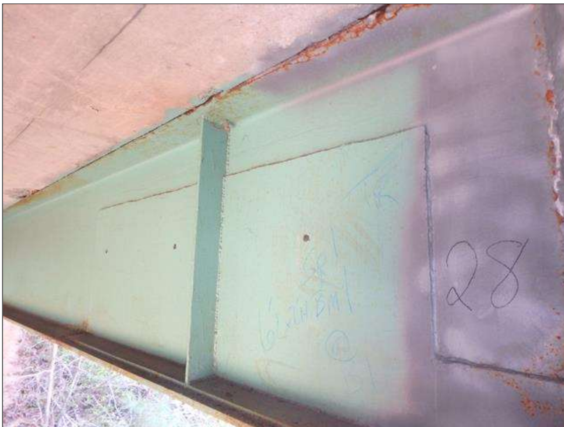
Temporary Repair Plate welded to Beam 1 right side Web and bottom flange at Bent 1.
