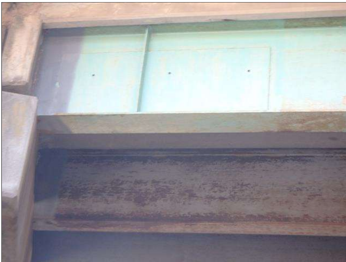
Span 1 Beam 1 at Bent 1, left side, Temporary Repair to Section Loss, 3/8" thick plates welded to web.
