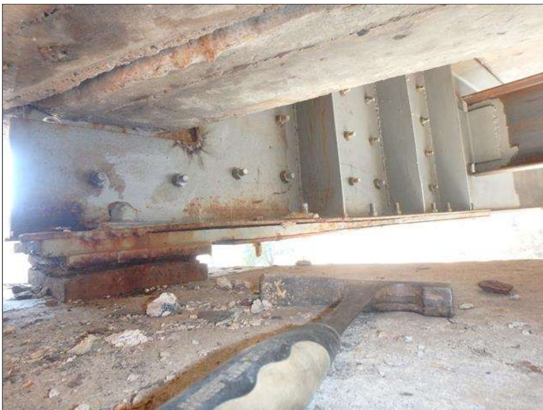
Span 3 Beam 5 at Bent 3, Temporary Repair to Section Loss, 1/4" thick plates bolted to web and bottom flange.
