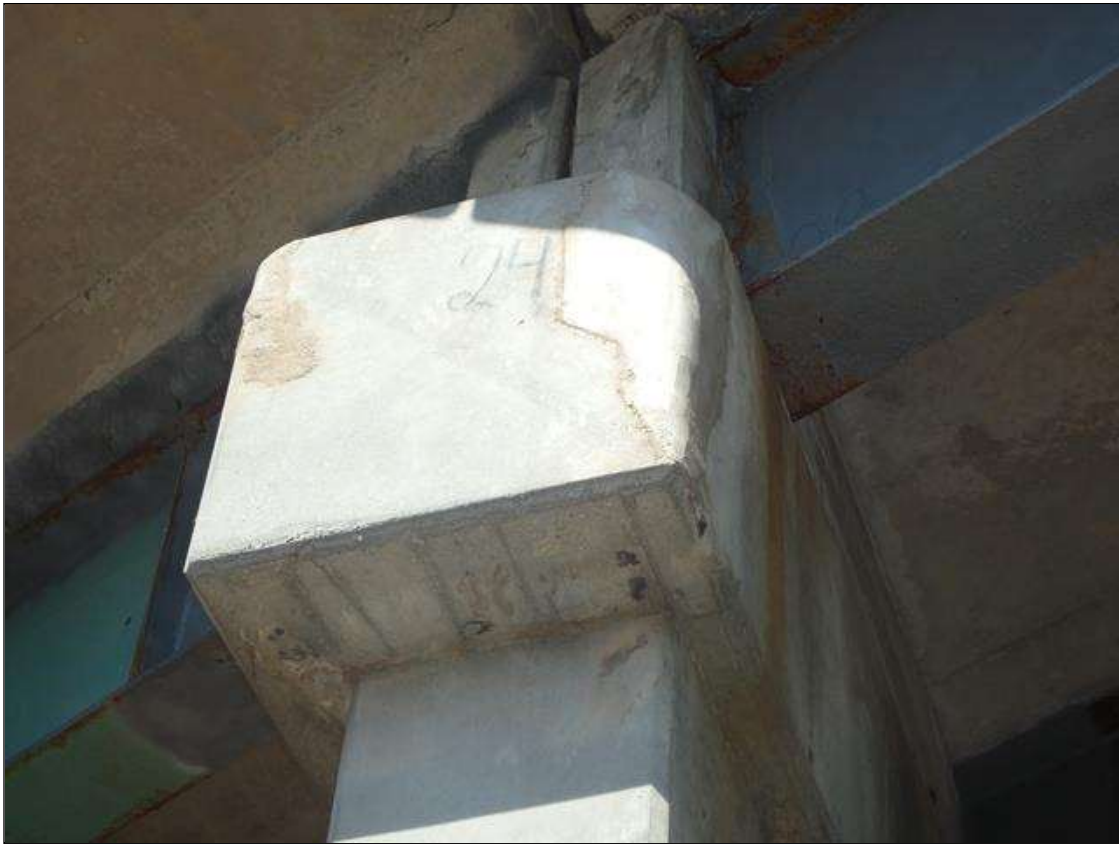
Bent 1 cap right end, sound patches.
