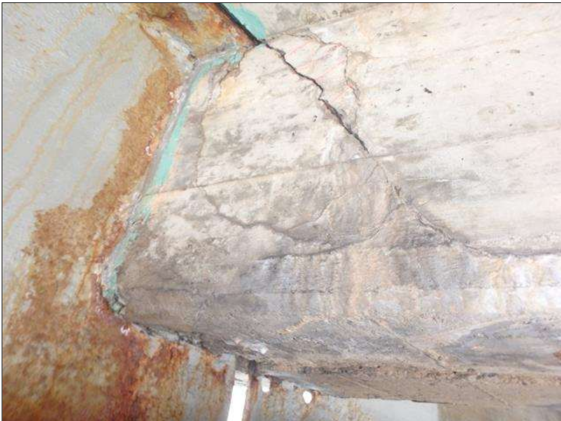
Span 2 RC end diaphragm at Bent 2 in bay 1 diagonal crack 1/8" wide and Delamination.
