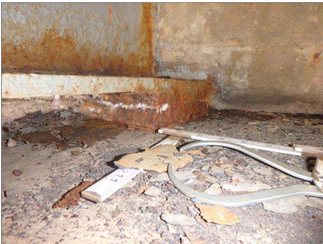
Span 4 Bearing Assembly seat 1 at End Bent 2: Active Corrosion and Section Loss <25% in the plates.
