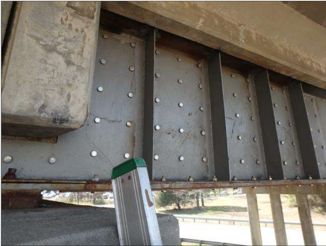
Span 3 Beam 1 at Bent 3, Temporary Repair to Section Loss, 1/4" thick plates bolted to both sides of web and bottom flange.
