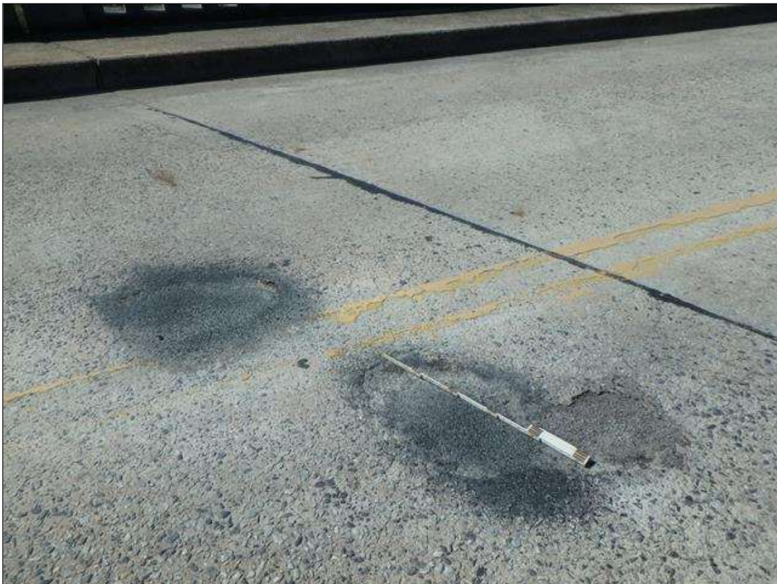
Span 3 Deck surface near Bent 2 joint at c/l, (2) sound patches to spalls.
