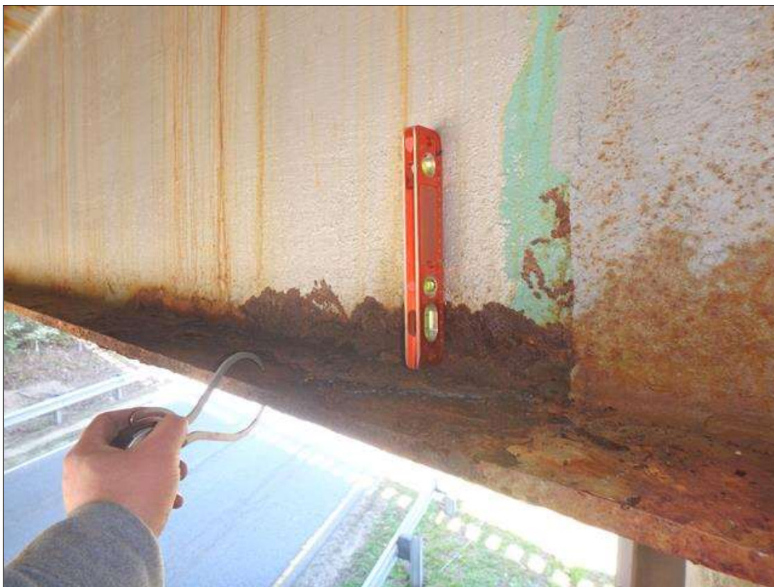
PRIORITY MAINTENANCE: Span 2 Beam 1 at 2' from Bent 2, Active Corrosion and Section Loss in lower web and bottom flange.
