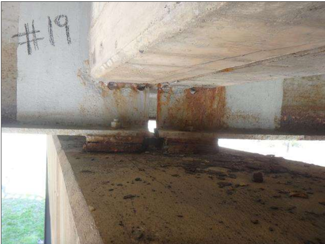
Spans 2 and 3 Beam 3 at Bent 2, end of beams below diaphragm has Section Loss, Surface Corrosion/Freckled Rust initiated since beam was cleaned and painted.
