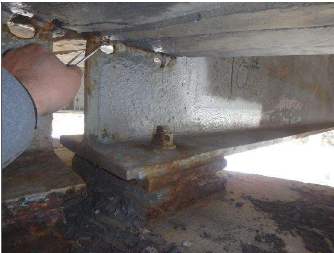
Span 3 Beam 4 at Bent 3 Section Loss in the web below diaphragm, Freckled Rust initiated since beam was cleaned and painted.
