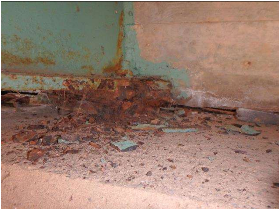
Span 1 Bearing Assembly seat 5 at End Bent 1, Active Corrosion and Section Loss <25% in the plates.
