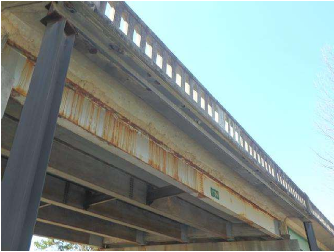
Temporary Repair: Span 2 Deck left overhang supported by steel H-Pile crutch from bents 1 to 2.
