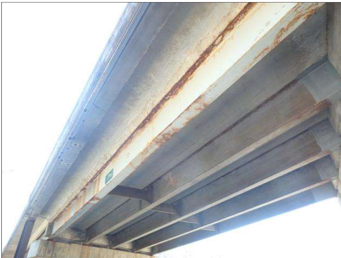
Span 2 Beam 1 above Right South bound lane, impact damage previously straightened/repared.
