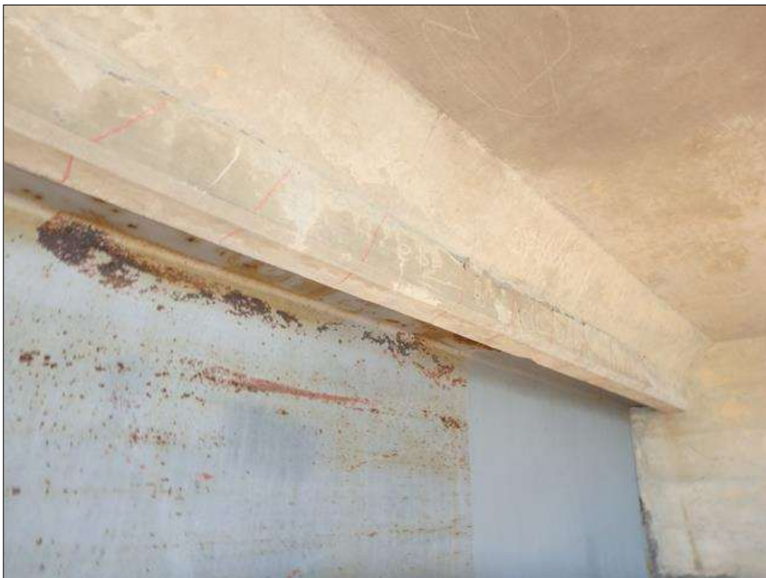
Span 4 Deck underside in right overhang, beginning at End Bent 2, Delamination in build-up adjacent to beam 5.
