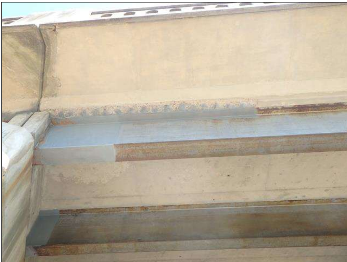
Span 2 Deck underside at Bent 1 in right overhang, spall no exposed steel in build-up along beam 5.
