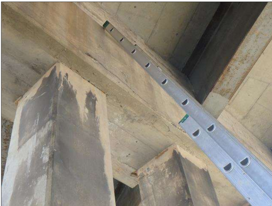
Bent 2 Cap west side bottom corner from column 3 to 4, 1/8" longitudinal crack and Delamination.
