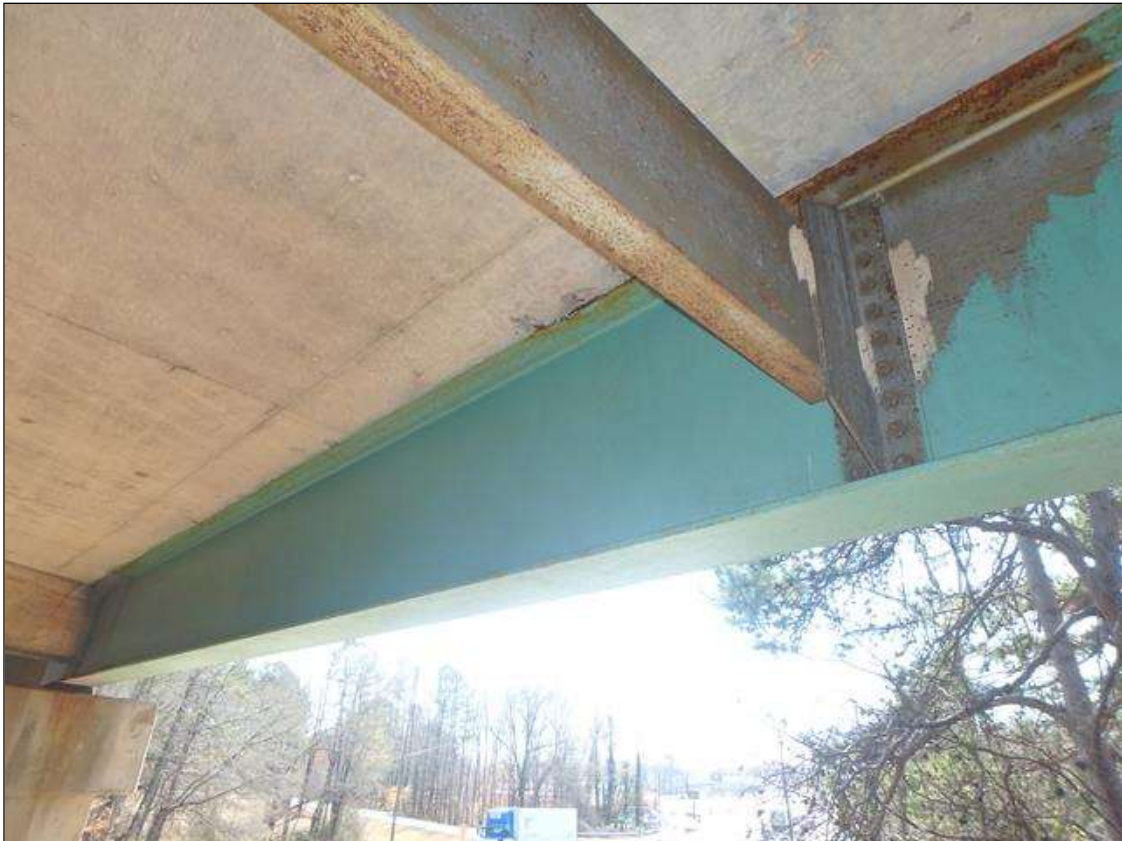
Span 1 Beam 5 Freckled Rust /Surface Corrosion in the flanges and web.
