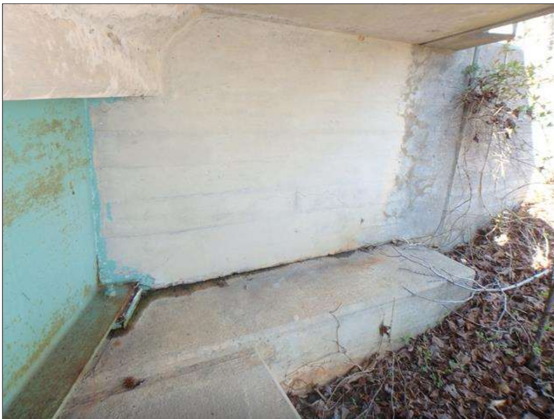
Abutment 1 in left overhang has up to 1/32" cracks.
