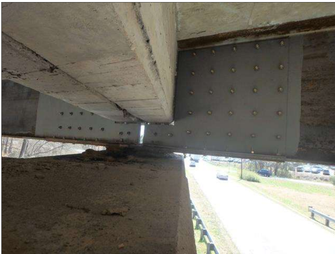
Spans 2 and 3 Beam 5 at Bent 2, Temporary Repair to Section Loss, 1/4" thick plates bolted on both sides of beam in web and bottom flange.
