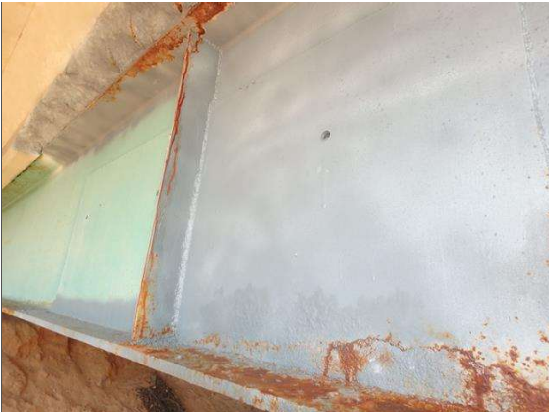
Span 1 Beam 5 at Bent 1, Temporary repair, plates welded to right side of web
