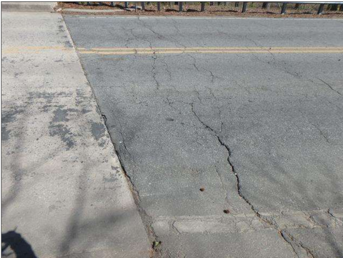
East Approach Pavement at bridge settled up to 1" with transverse cracks 1/8" to 1/2" wide.
