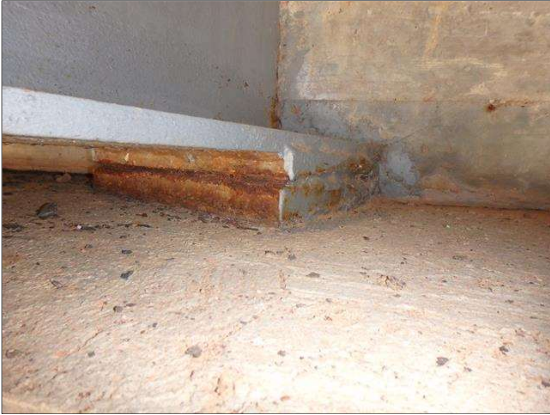
Span 4 Bearing Assembly seat 2 at End Bent 2: Active Corrosion and Section Loss <25% in the plates.
