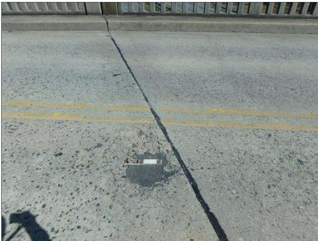
Span 1 Deck surface at Bent 1 joint near c/l, sound patch and spall with alligator cracks, loose concrete.
