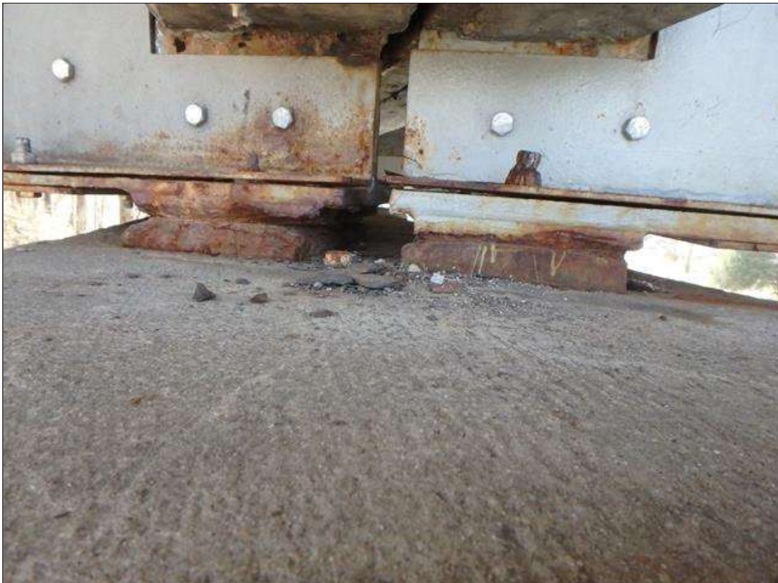
Spans 3 and 4 Bearing Assembly seat 1 at Bent 3, Active Corrosion and Section Loss in plates, Section Loss in anchor rods down to 3/8" Remaining.
