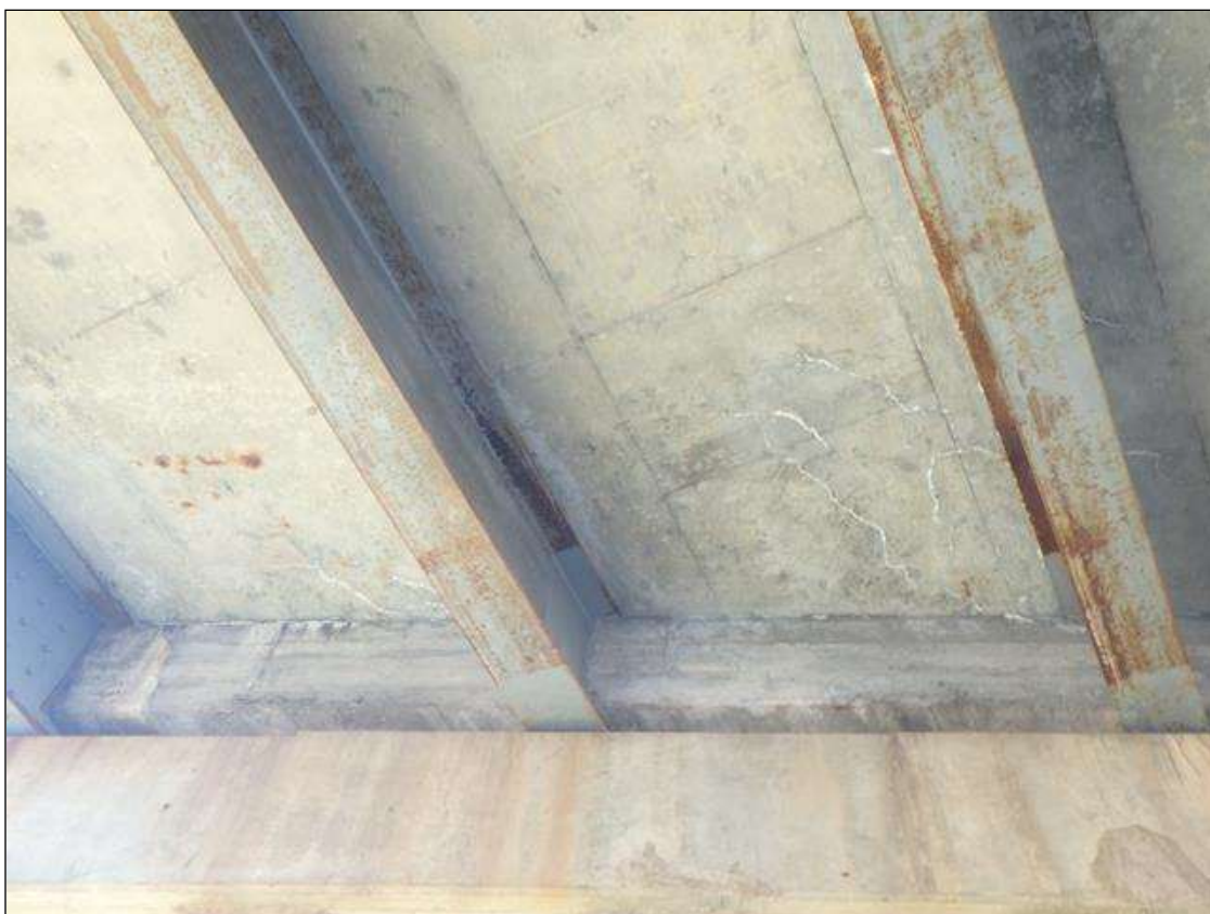
Span 3 Deck underside at Bent 2, 1/32" map cracks with surface efflorescence in bays 2 thru 4.
