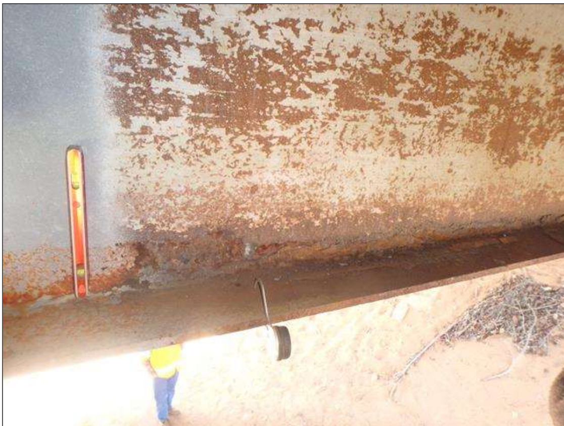
PRIORITY MAINTENANCE: Span 1 Beam 2 near Bent 1, Active Corrosion & Section Loss in the lower web and bottom flange.
