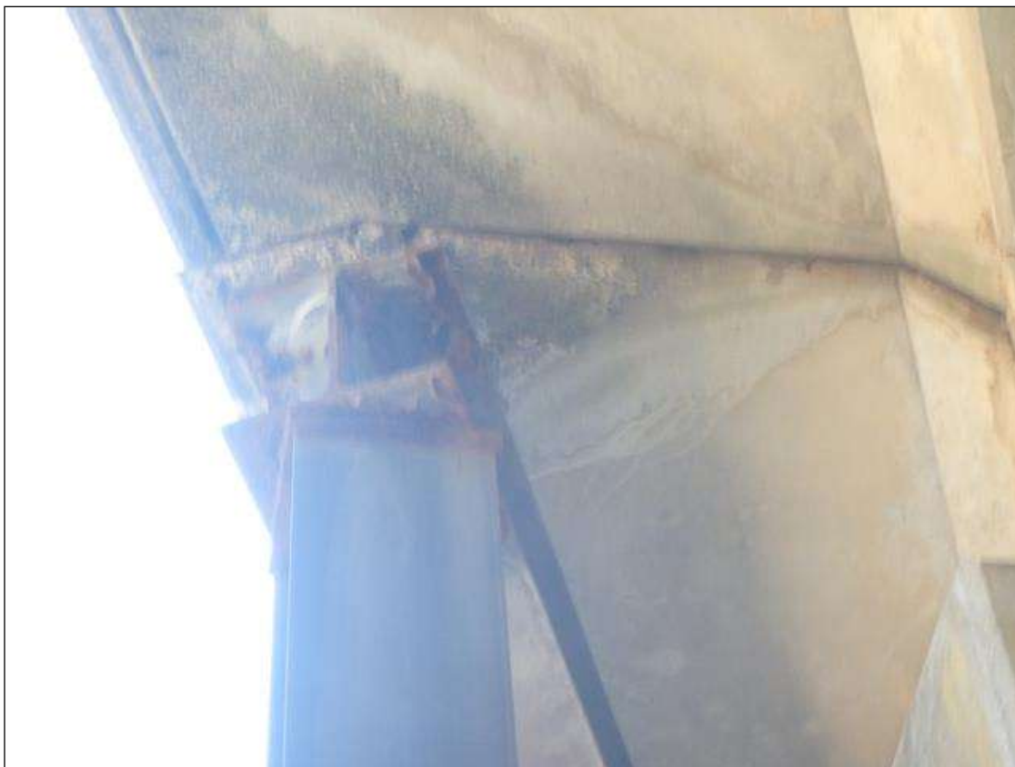
Steel H-Pile supporting Span 2 Deck left overhang at Bent 1, loose bolt thru top right flange with spall in underside of Deck.
