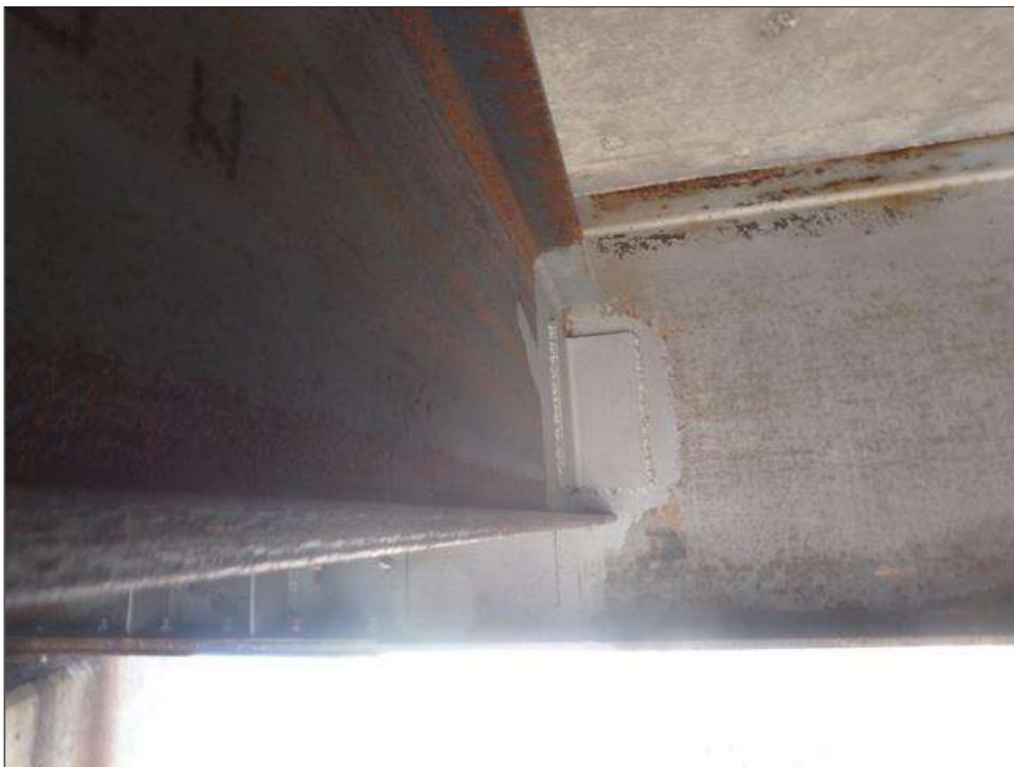
Span 4 steel intermediate diaphragm in bay 1 near Bent 3 weld connection to beam 1.
