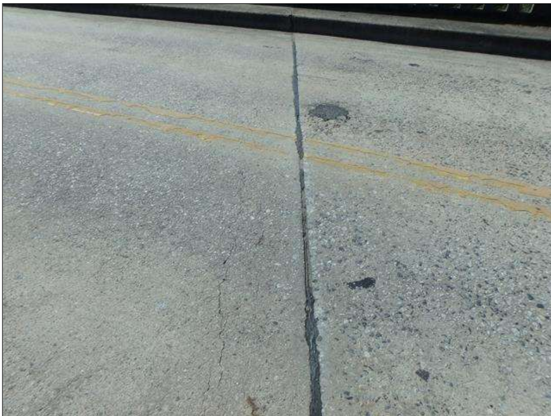
Bent 1 joint pourable seal pulled out exposing backer material near c/l and at curbs.
