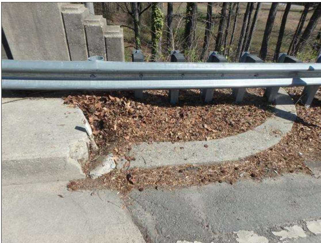
left RC sidewalk at End Bent 2, Spall with Exposed Steel, curb flare at Northeast Corner settled 8".
