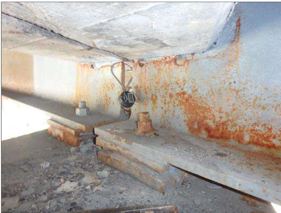
Spans 1 and 2 end of beam 2 at Bent 1, Section Loss in web below diaphragm, Surface Corrosion initiated.
