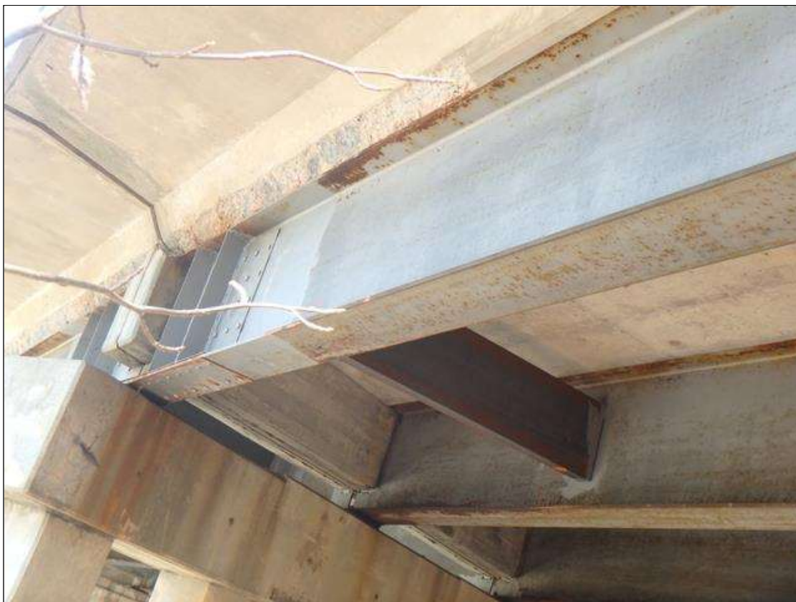
Span 4 Deck underside in right overhang, beginning at Bent 3, spall in build-up adjacent to beam 5.
