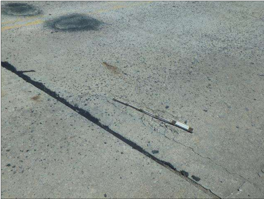
Span 3 Deck surface at Bent 2 joint near right curb, 1/16" cracks and Delamination.
