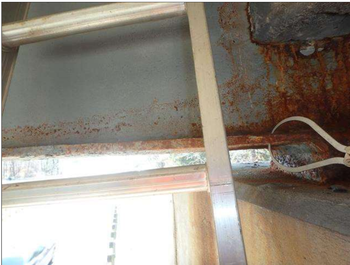
Span 2 Beam 5 at Bent 1, Section Loss in lower web and bottom flange, Surface Corrosion/Freckled Rust initiated since beam was cleaned and painted.
