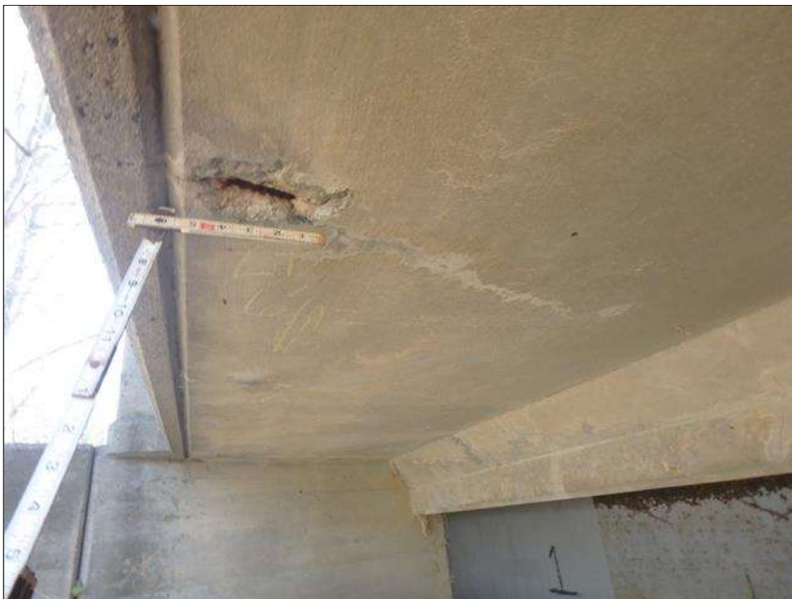
Span 4 Deck underside left overhang 6' from End Bent 2, Spall with Exposed Steel.
