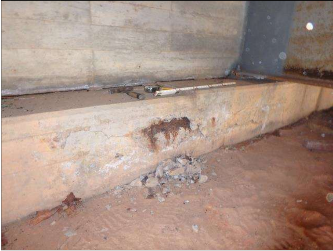
End Bent 1 Cap in bay 4, Spall with Exposed Steel and Delamination with cracks.
