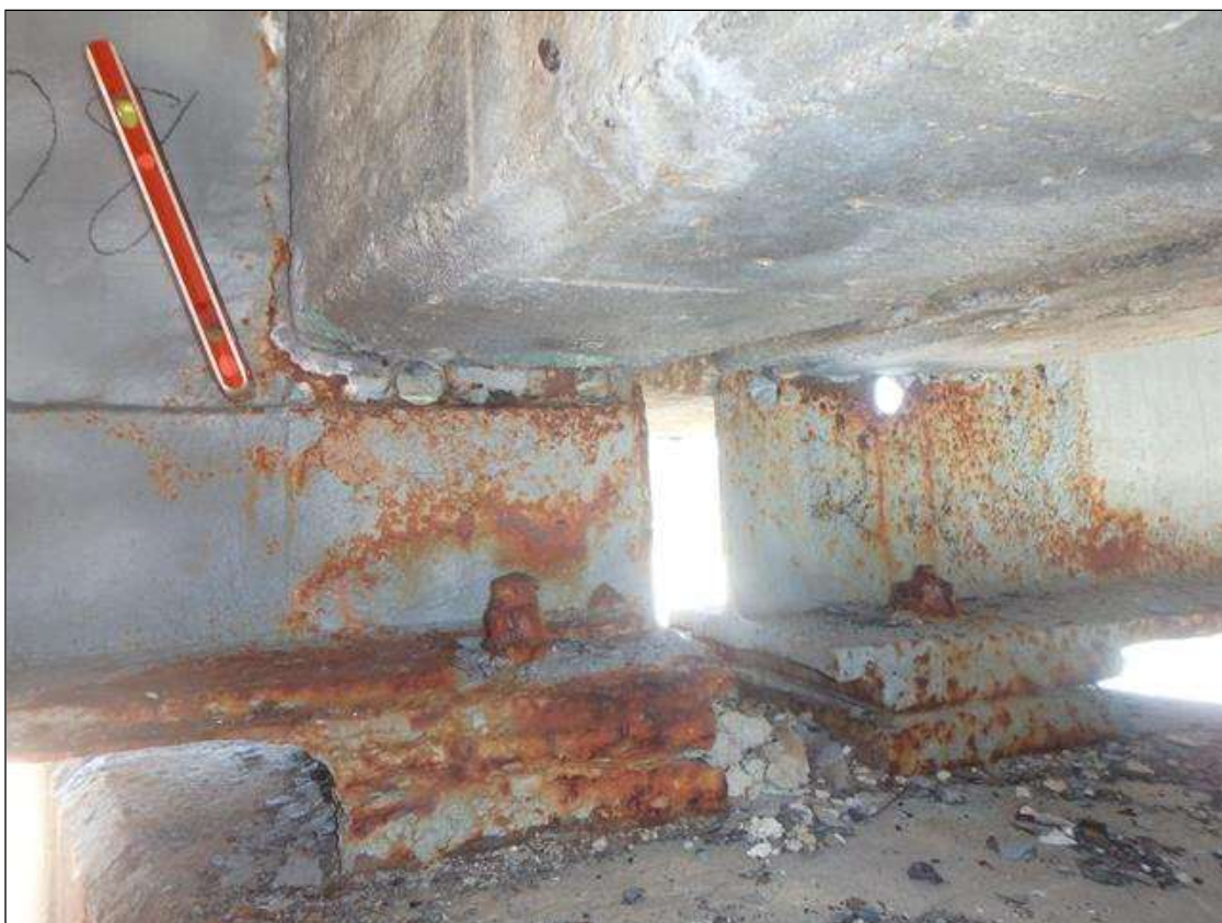
Spans 1 and 2 ends of Beam 1 at Bent 1, Section Loss in the web below the diaphragms, Freckled Rust/ surface corrosion initiated.
