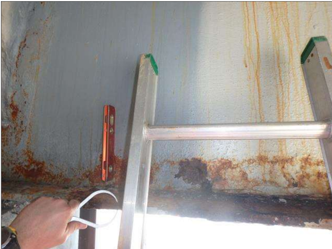
PRIORITY MAINTENANCE: Span 2 beam 1 at Bent 1, Active Corrosion & Section Loss in the lower web and bottom flange.
