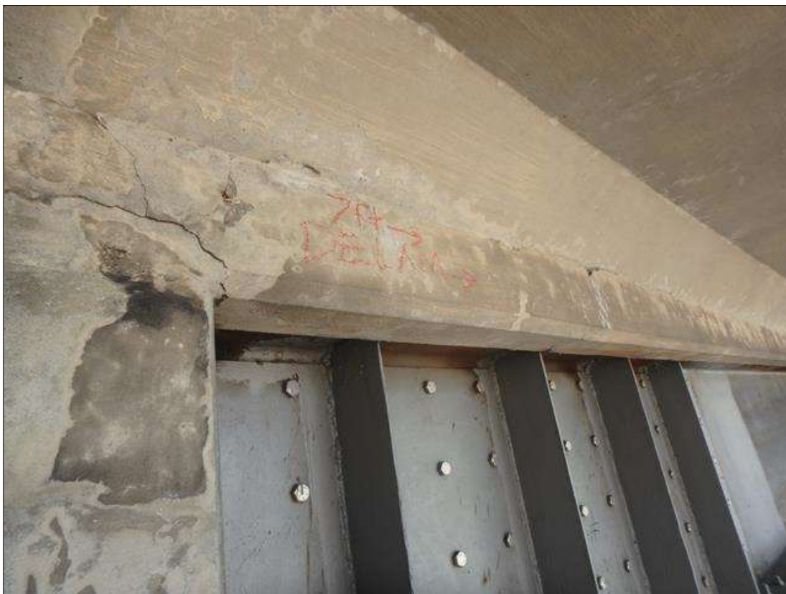
PRIORITY MAINTENANCE: Span 3 RC Deck underside left overhang at Bent 3, Delamination in build up 7' long x 6" x 4".
