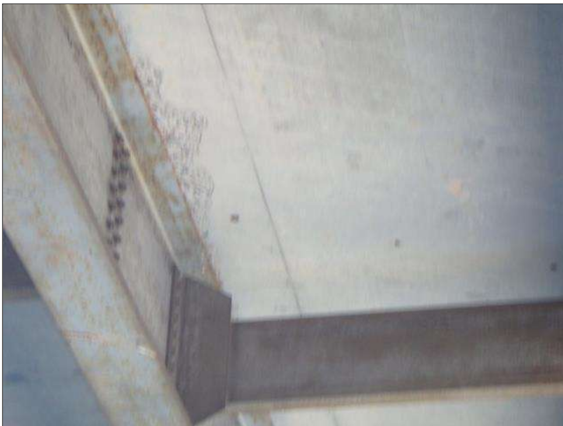
Span 2 Deck underside at mid-Span in bay 2 along beam 2, spall no exposed steel.
