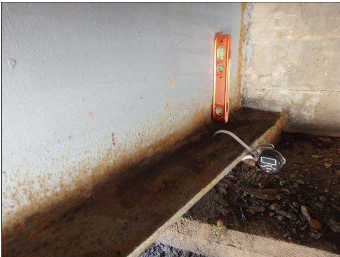
PRIORITY MAINTENANCE: Span 4 Beam 1 right side at End Bent 2, bottom flange has Active Corrosion and scale with Section Loss, Lower web has Section Loss with corrosion initiated.
