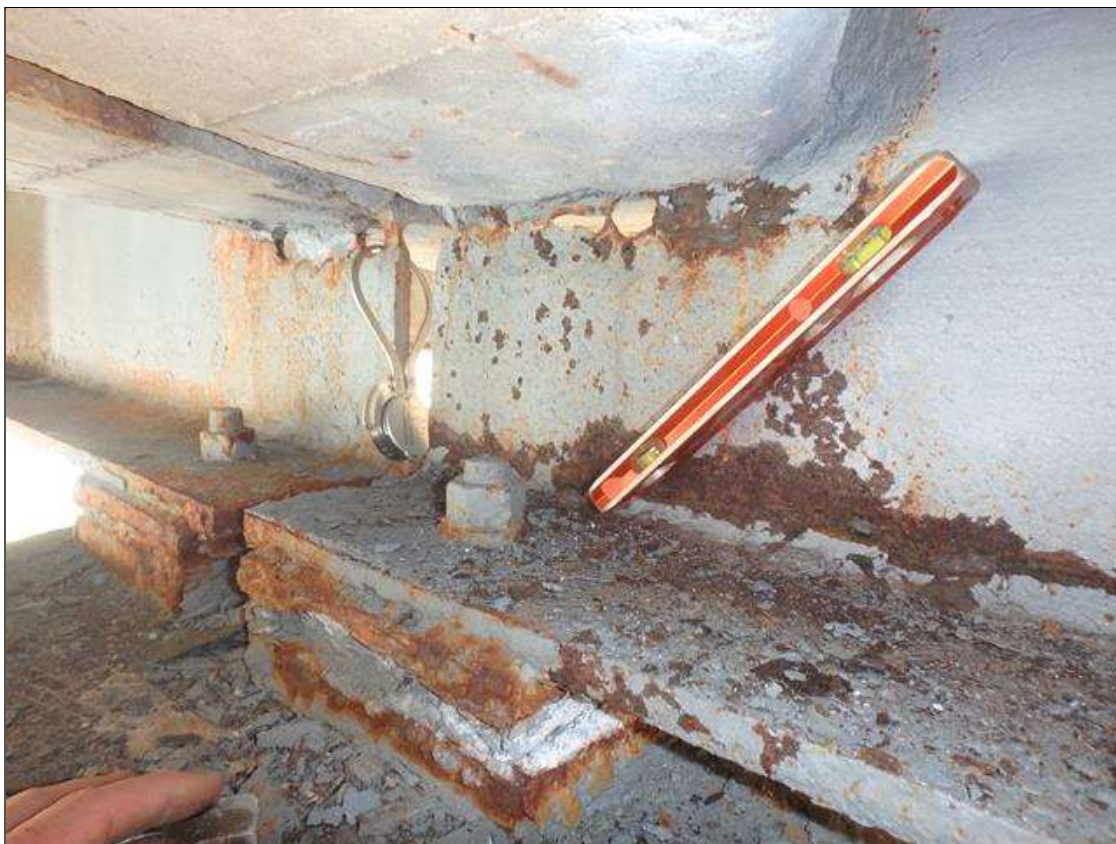
PRIORITY MAINTENANCE: Span 1 Beam 4 at Bent 1, Active Corrosion and Section Loss below end diaphragm and in lower web at bottom flange.
