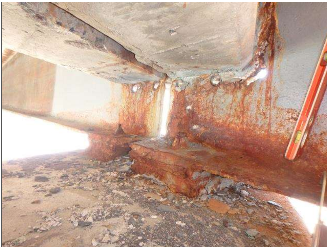
Spans 1 and 2, beam 5 at Bent 1 Section Loss in the web at diaphragm and along bottom flange.
