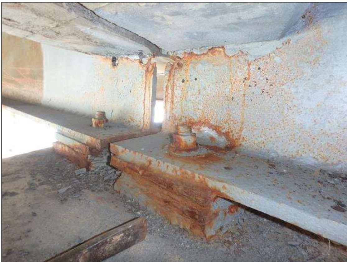
Spans 1 & 2 ends of beam 3 at Bent 1, Section Loss in the web below diaphragm, Freckled Rust/Surface Corrosion initiated since beam was cleaned and painted.
