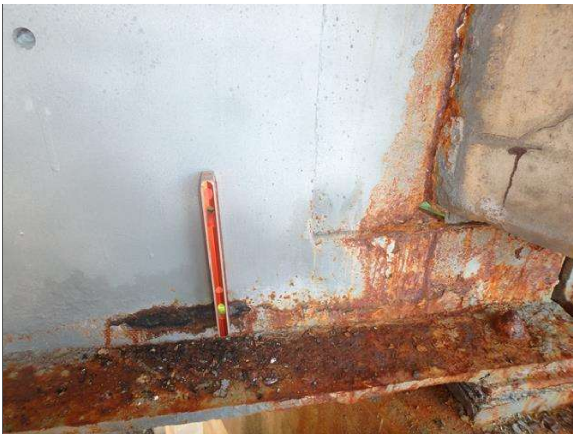
Span 1 Beam 5 at Bent 1, Repair plate welded to right side of web has Active Corrosion and Section Loss in lower web.
