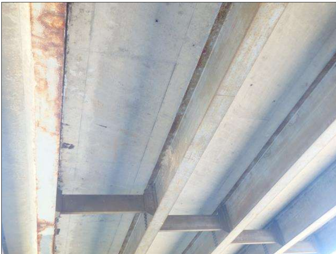
Span 2 Beam 2 above Right South Bound lane, impact scrapes to bottom flange.
