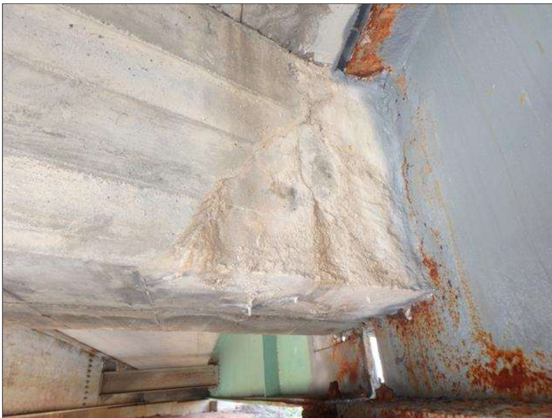
Span 2 RC end diaphragm at Bent 1 bay 1, 1/8" cracks with efflorescence buildup.
