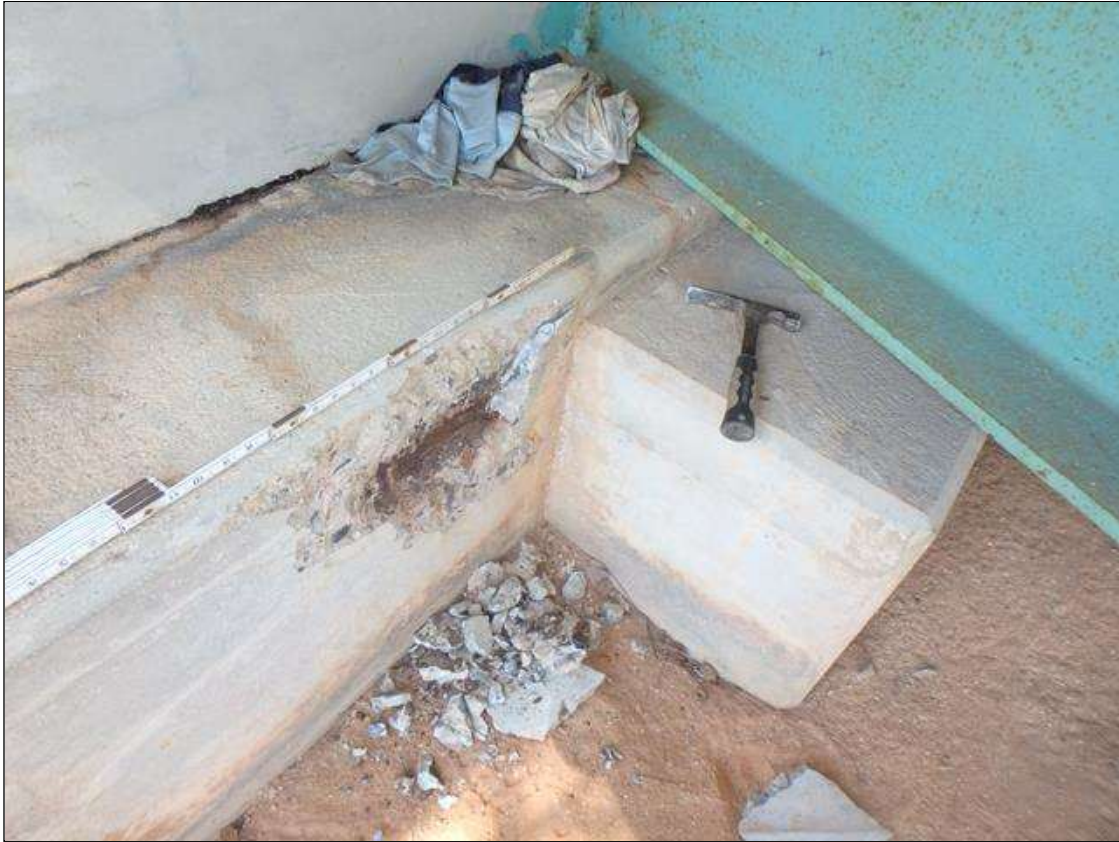
End Bent 1 Cap below right overhang near brace pile, Spall with Exposed Steel.
