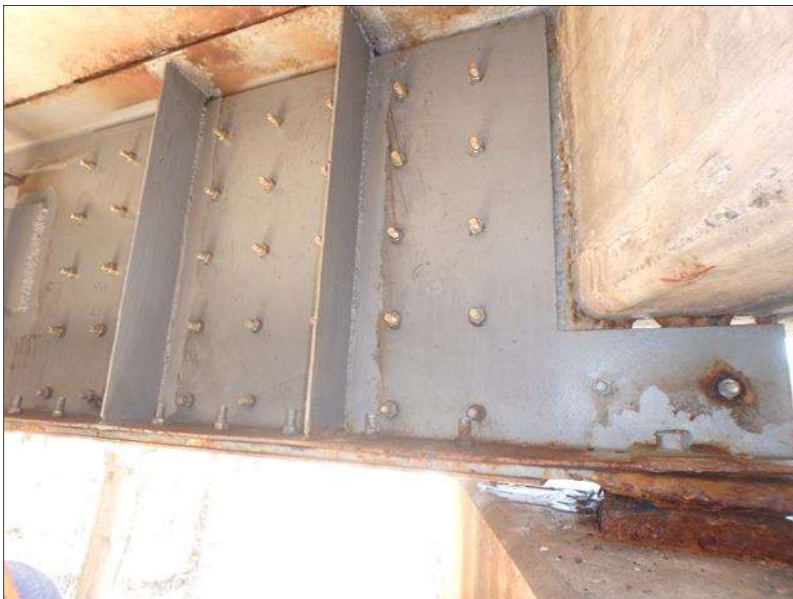
Span 4 Beam 5 at Bent 3, Temporary Repair to Section Loss, 1/4" thick plates bolted to web and bottom flange.
