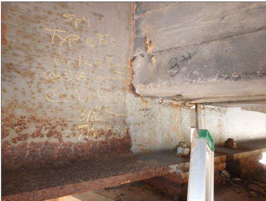
Spans 3 and 4 Beam 2 at Bent 3, end of beams Section Loss in the web below diaphragm, Freckled Rust initiated since beam was painted.
