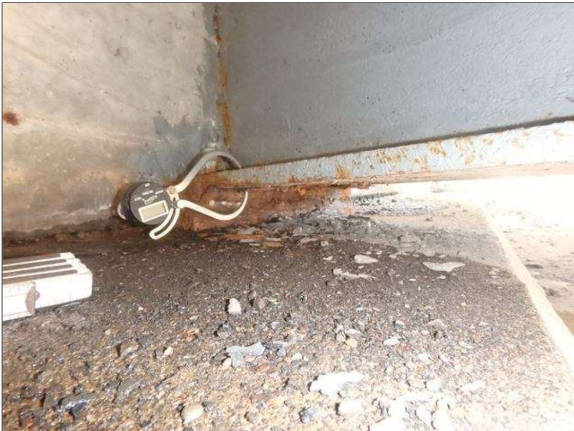
PRIORITY MAINTENANCE: Span 4 Beam 5 at End Bent 2, bottom flange in front of bearing, Active Corrosion and Section Loss.
