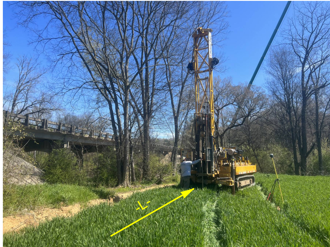
RIG ON EB1-C FACING UP STATION
