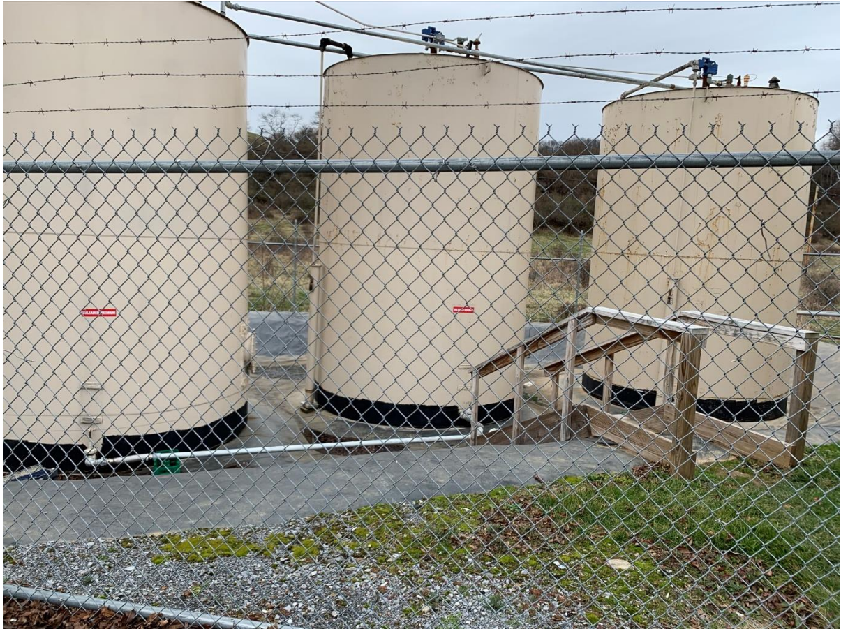
Large ASTs in the fenced area.
