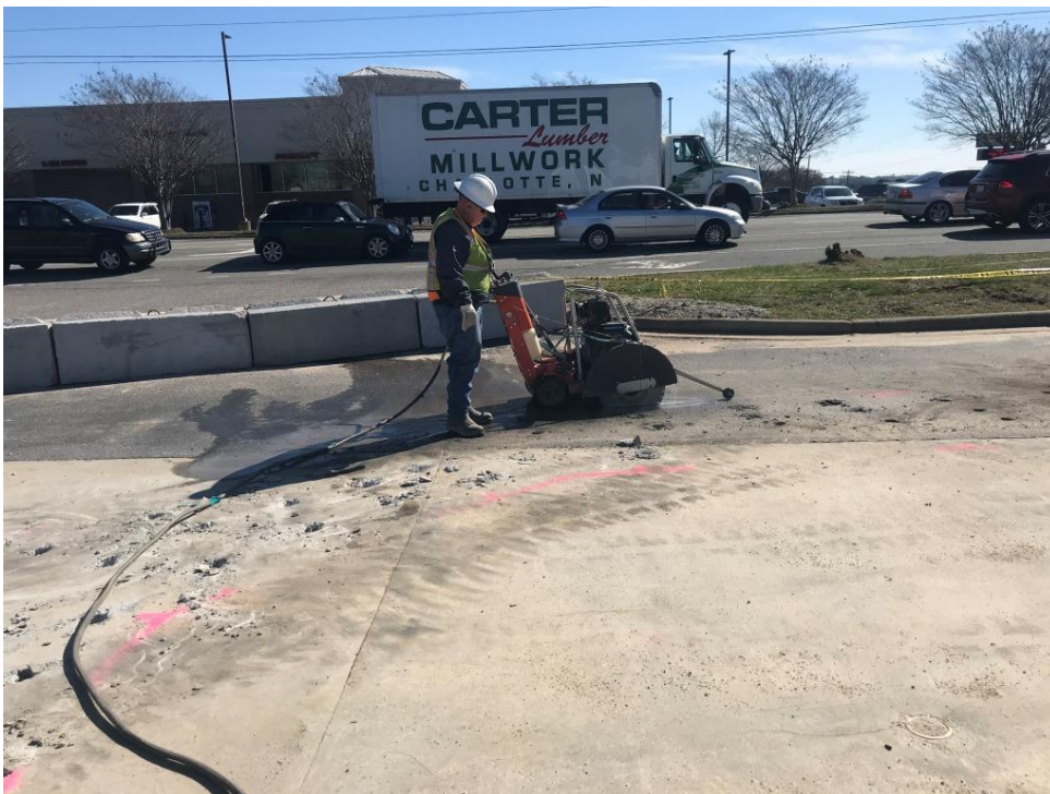
Photograph 12: CCI using a concrete saw to cut concrete and asphalt along product line trenches.
