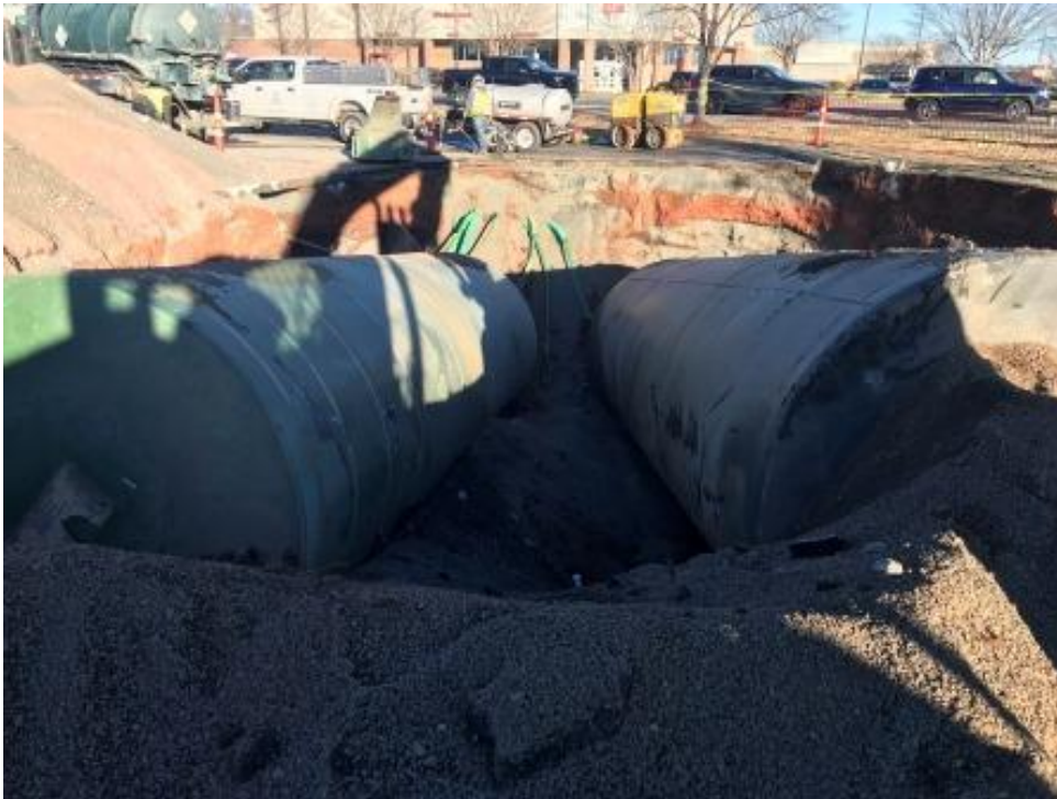
Photograph 5: USTs #1 (right) and #2 (left).
