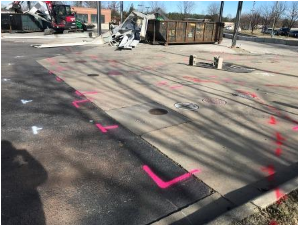
Photograph 1: UST locations outlined in pink by private utility locator.
