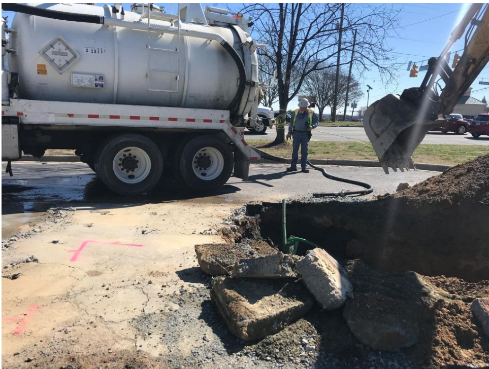
Photograph 14: CCI using a vacuum truck to remove any remaining liquid in the product lines.
