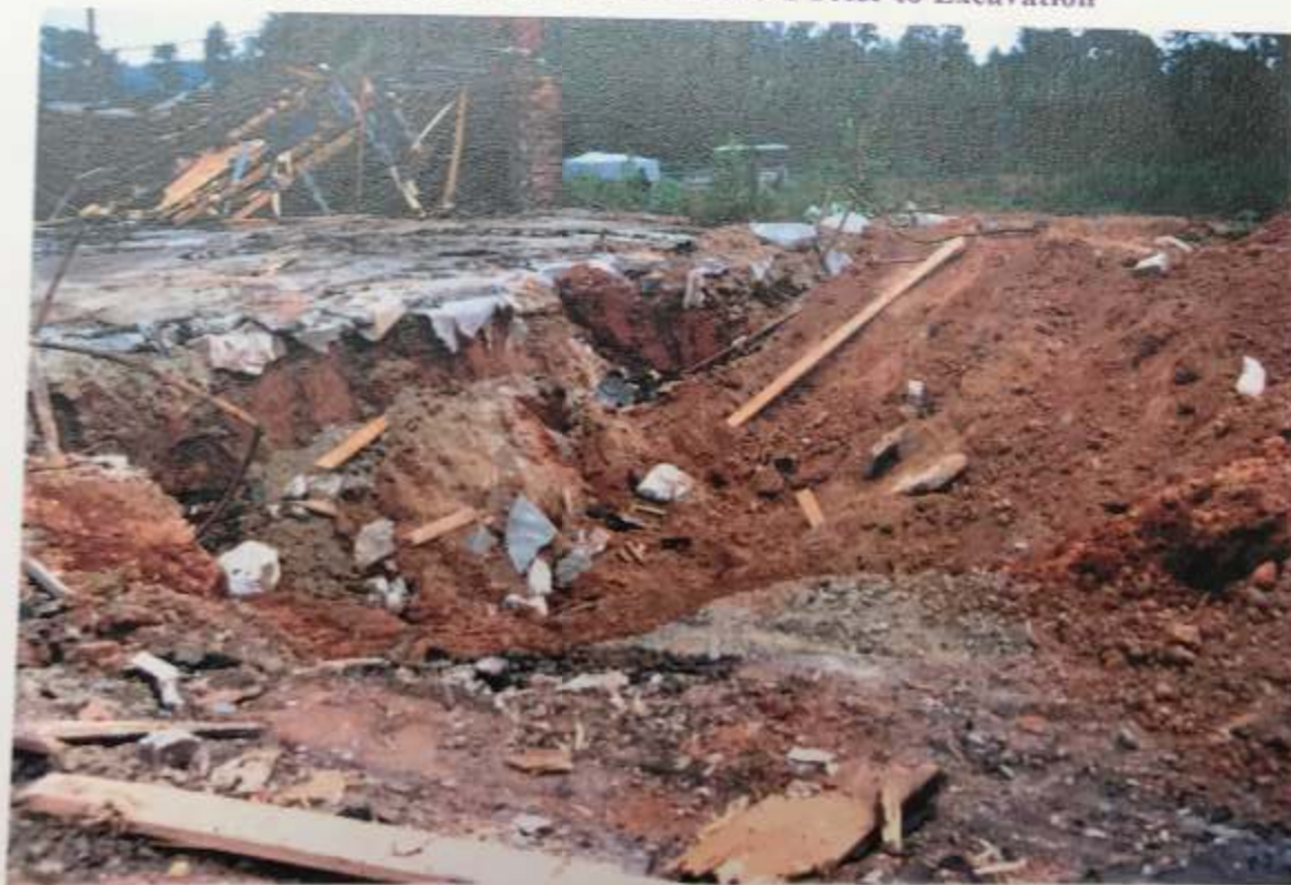
Photograph 2: Main Tank Excavation, Tanks S-1, S-2 & S-3. Vent piping in background; product lines to far left. View is to the southeast.
