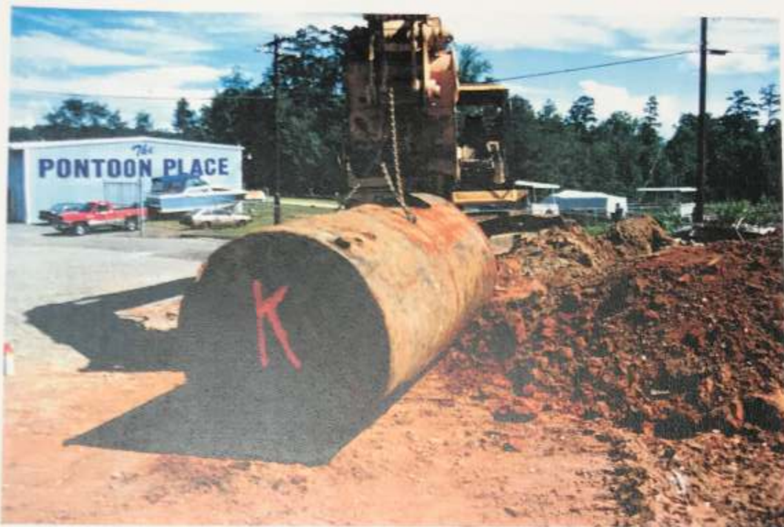
Photograph 8: Tank S-4 (Kerosene)
