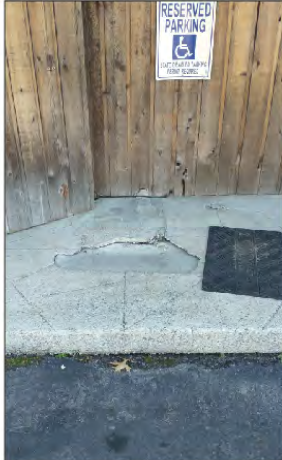
Photo 4. Patched concrete showing possible former dispenser.
