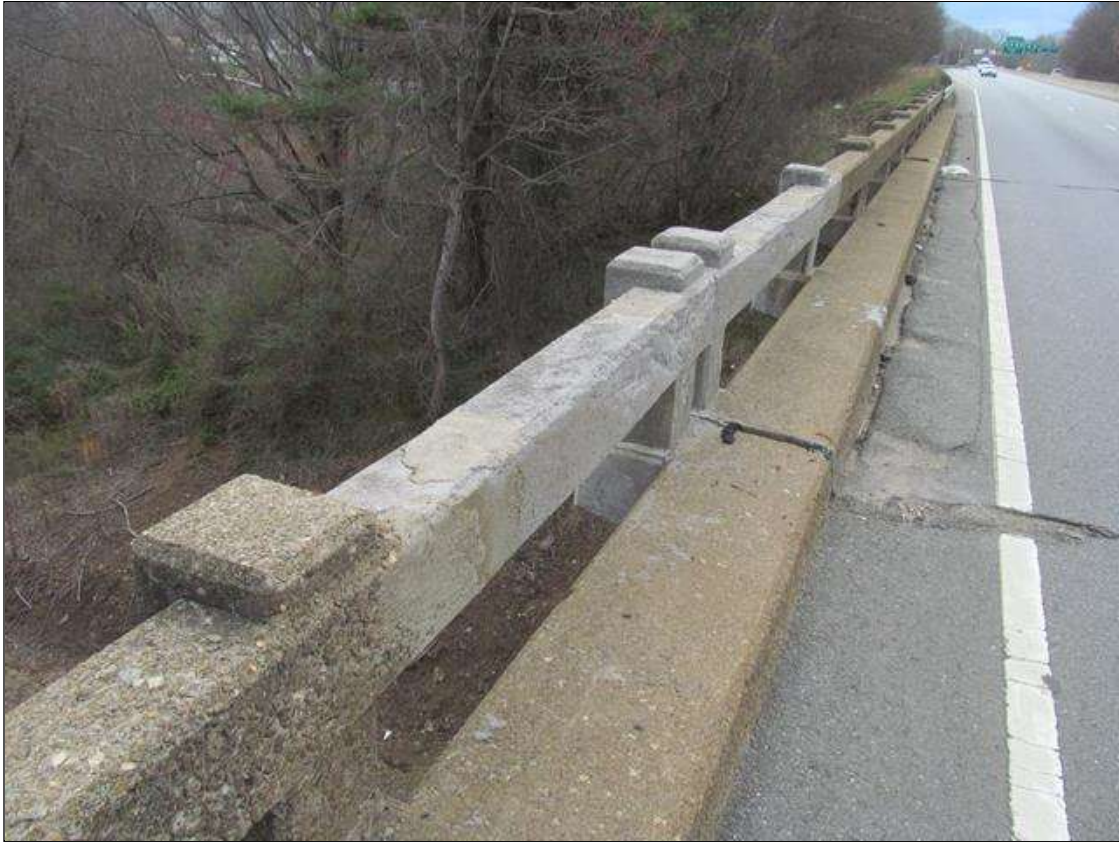
RT RAIL AT BENT 2, RC RAIL REPAIR FOR APPROX 20'L
