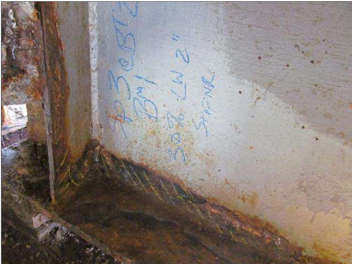
Span 3 Beam 1: BEAM END AT BENT 2, CORROSION WITH APPROX 30% SECTION LOSS (AVG 5/16" REMAINS) IN THE LOWER 2" OF THE WEB FOR APPROX 2'L. PMANT.
