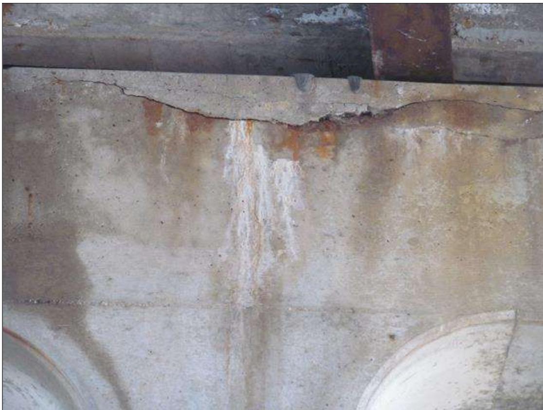
Bent 1 Cap 1: NORTH FACE, HORIZONTAL CRACKING UP TO 3/16"W WITH EFFLO AND RUST STAINING, SCATTERED.
