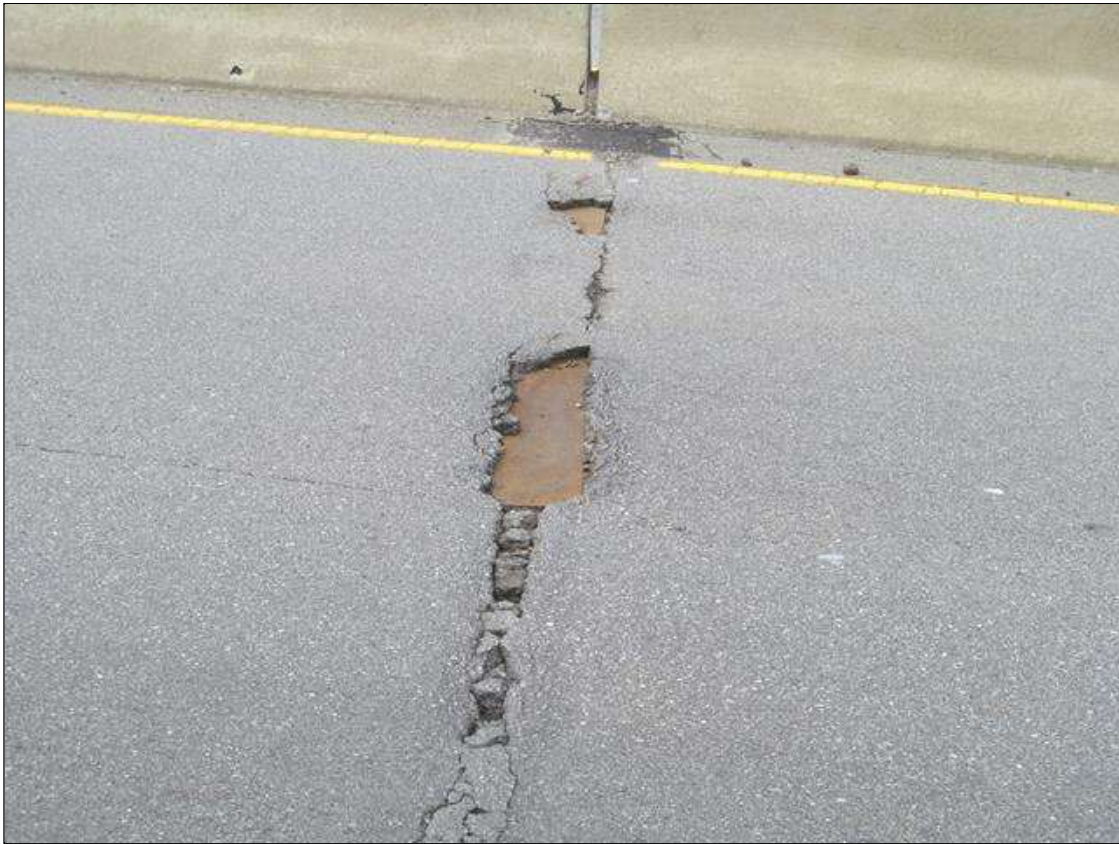
NBL AT BENT 1, METAL PLATE OVER THE JOINT HAS BEEN EXPOSED IN AREAS OF AWS LOSS.
