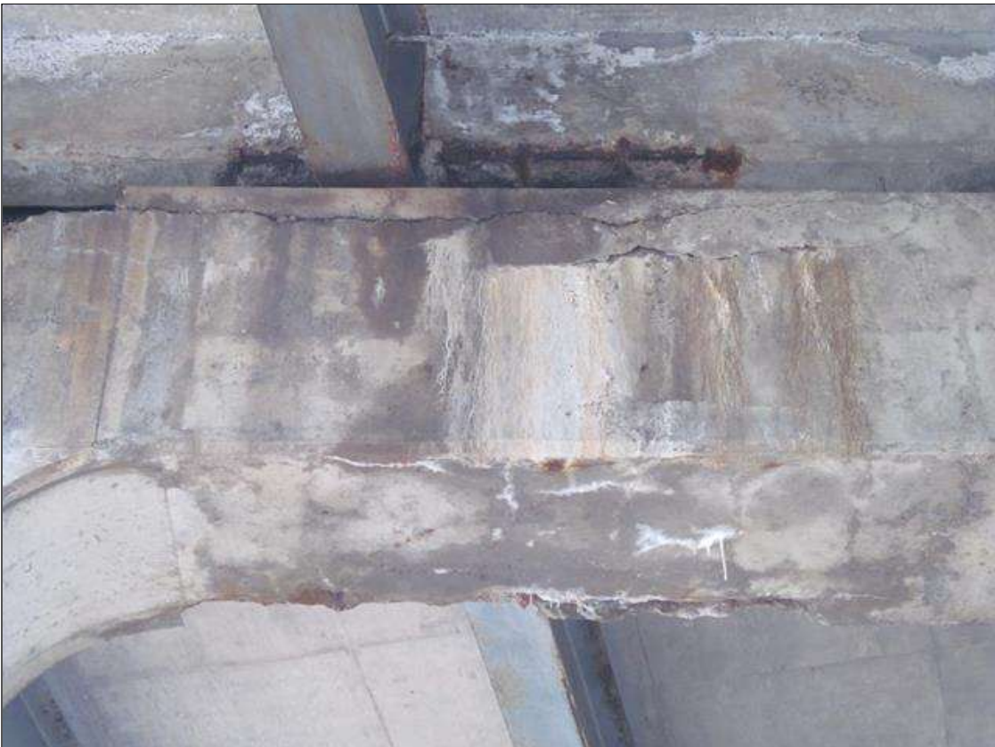
Bent 2 Cap 1: SOUTH FACE OF THE CAP, MAP CRACKING UP TO 1/8"W WITH EFFLOL STAINING, SCATTERED.
