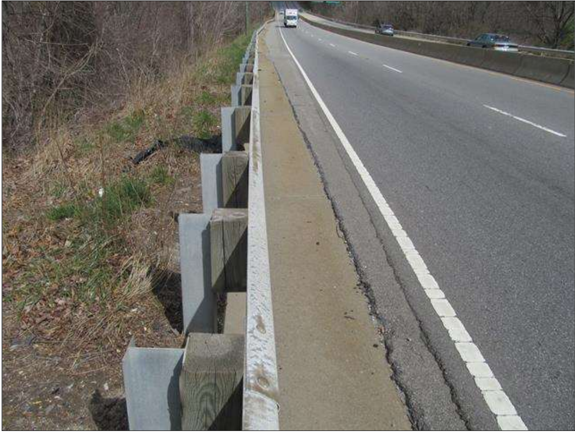
NW CORNER, GR TIED TO EXTENDED RAIL RUN
