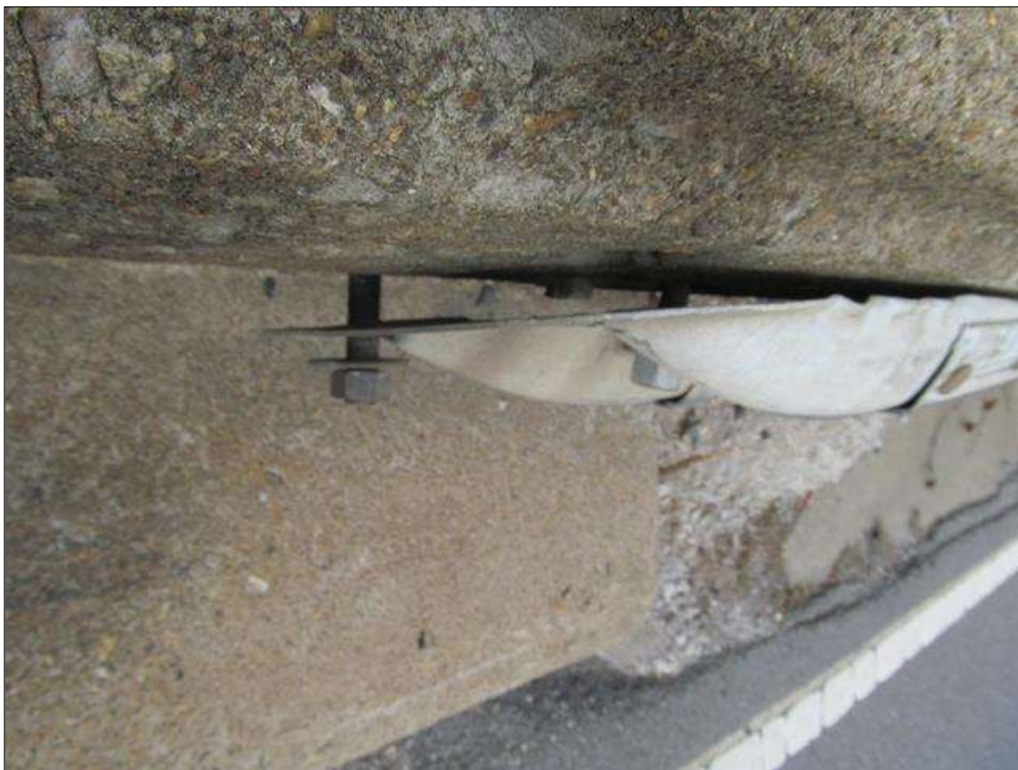
NW CORNER, GR FASTENERS ARE LOOSE OR MISSING.
