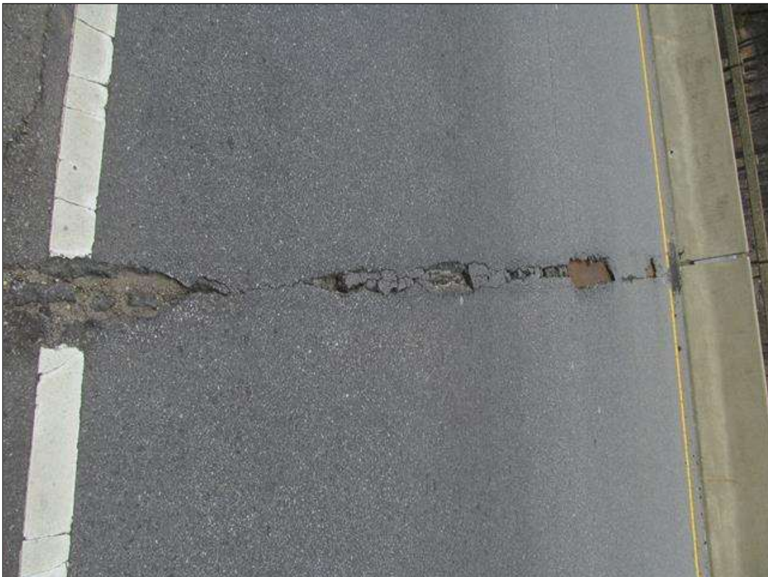
Span 1 Wearing Surface: AT BENT 1, SCATTERED SPALLING UP TO 2"D ALONG THE JOINT TOTALING APPROX 56SQFT
