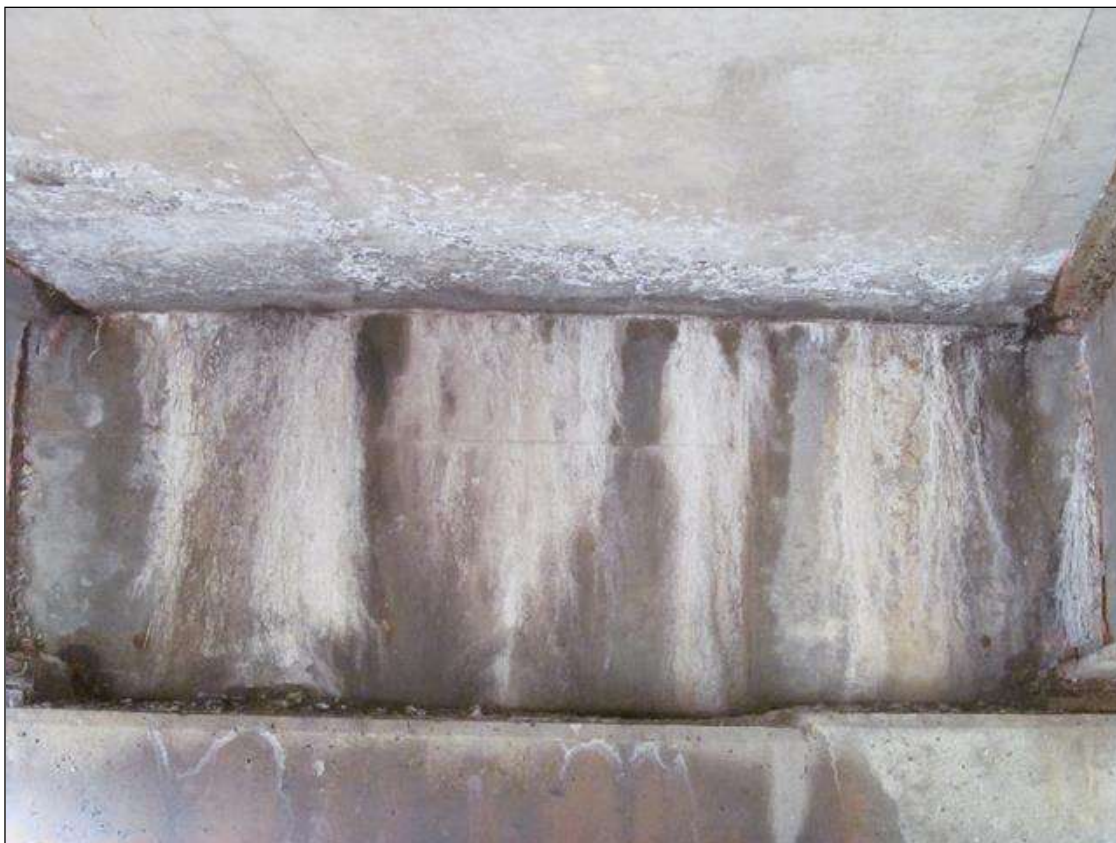
End Bent 2 Abutment/Backwall : BAY 1, SCATTERED EFFLO STAINING
