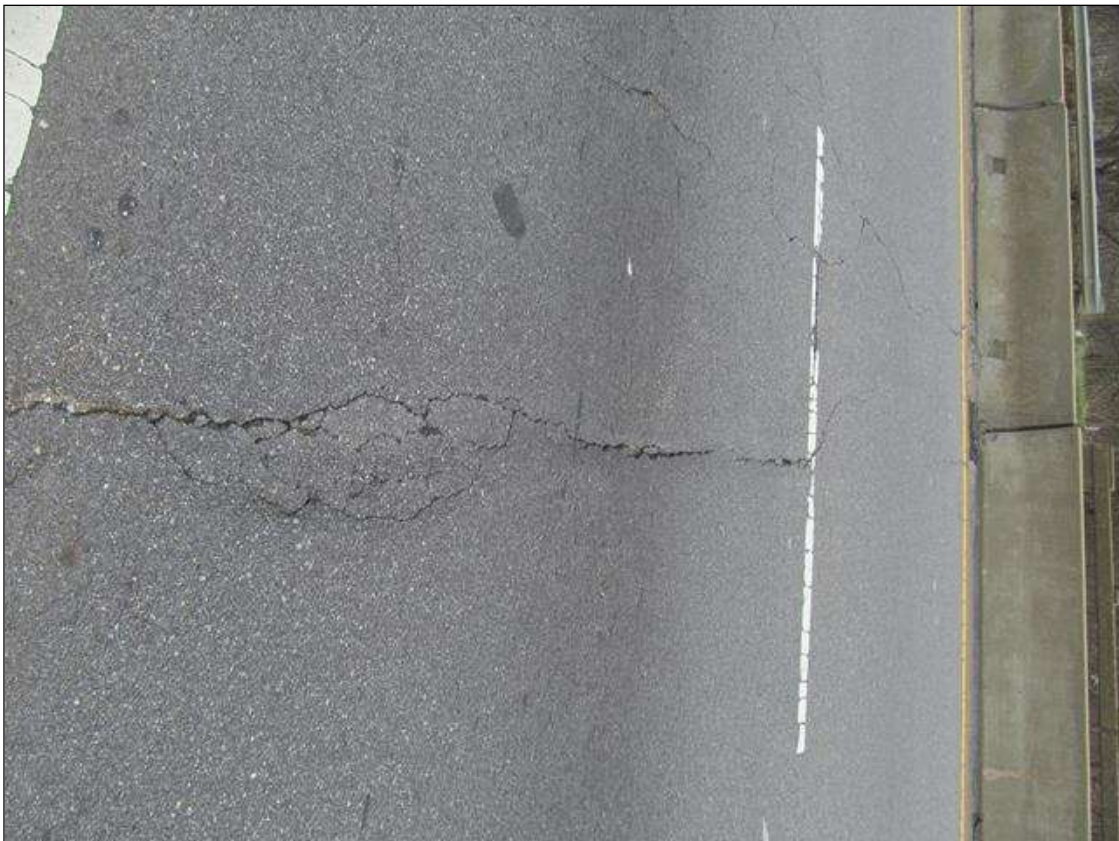
Span 3 Wearing Surface: AT THE NORTH APPROACH, FULL WIDTH TRANSVERSE CRACKING UP TO 1/8"W
