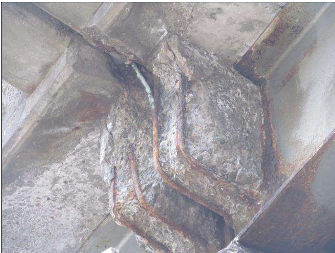
BENT 2, VIEW OF SPALLED CONCRETE END DIAPHRAGMS (LT OUTBOARD END)
