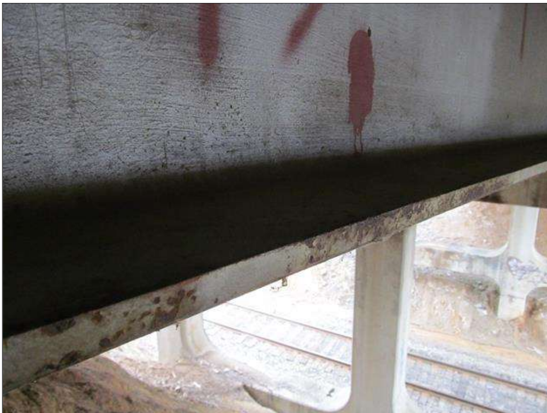
INBOARD BEAMS, SCATTERED FRECKLED CORROSION
