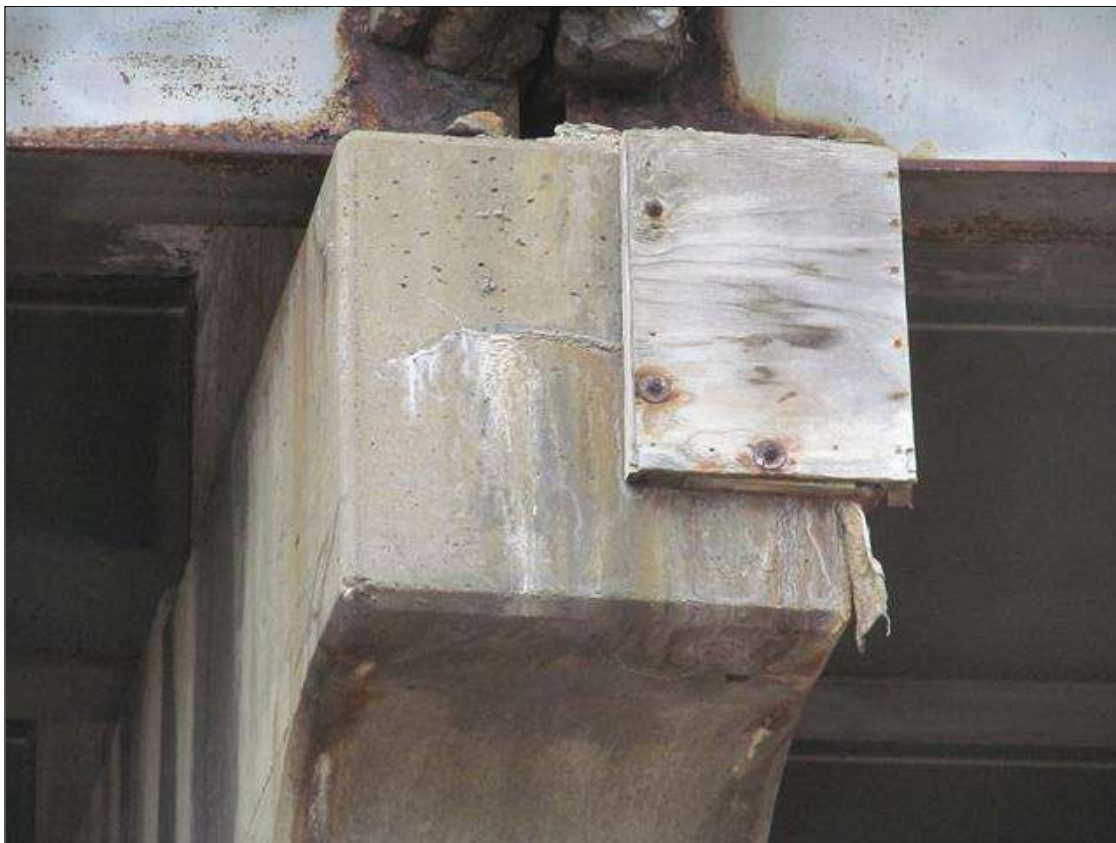
BENT 2 RT END, VIEW OF PREVIOUS REPAIR
