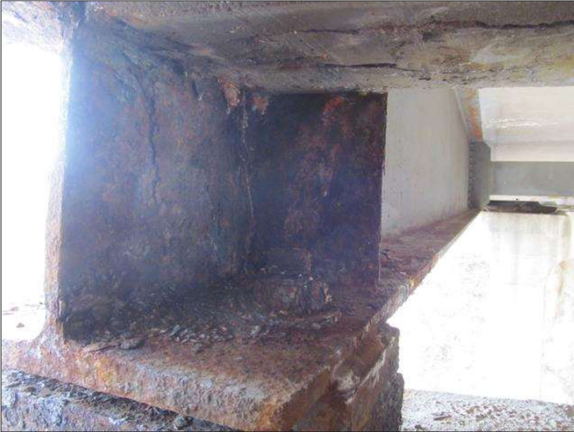
OUTBOARD BEAM ENDS AT BENT 2 HAVE SURFACE CORROSION WITH PITTING UP TO 1/16" AND LAYERED RUST.
