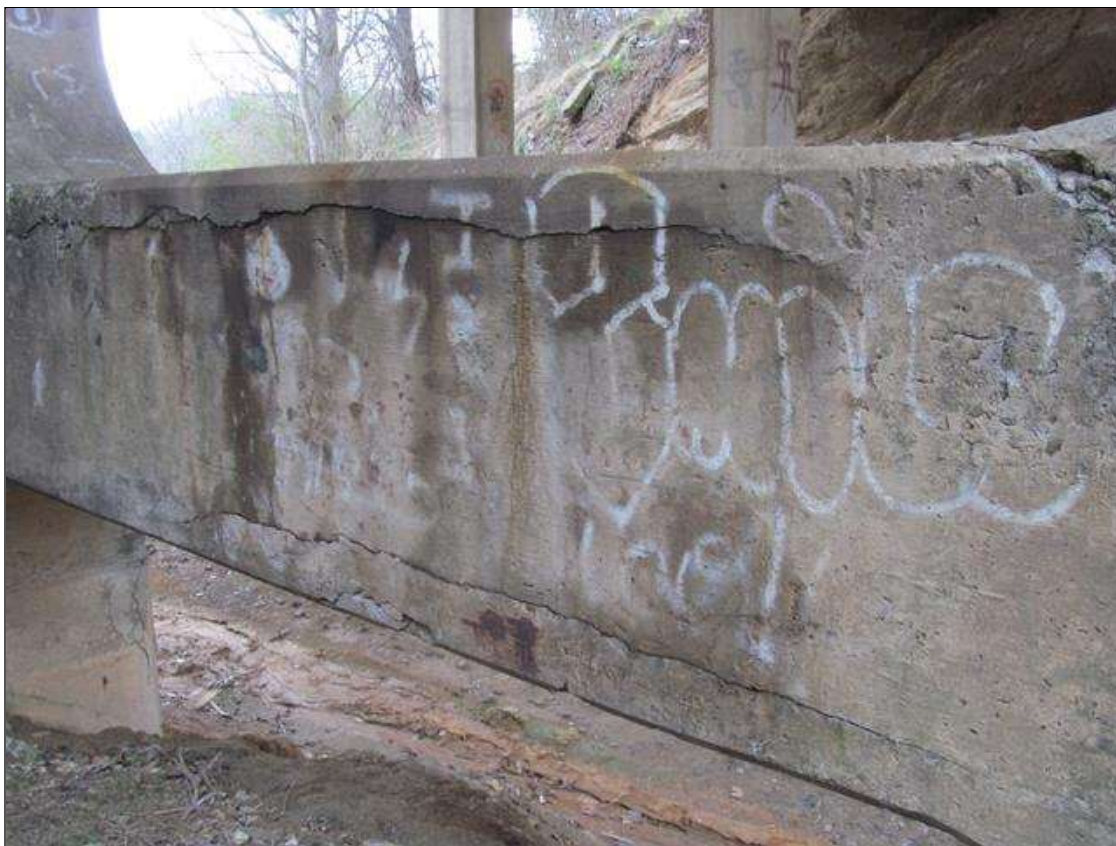
BENT 2, LOWER STRUTS HAVE HORIZONTAL CRACKING UP TO 1/4"W AT THE CORNERS.
