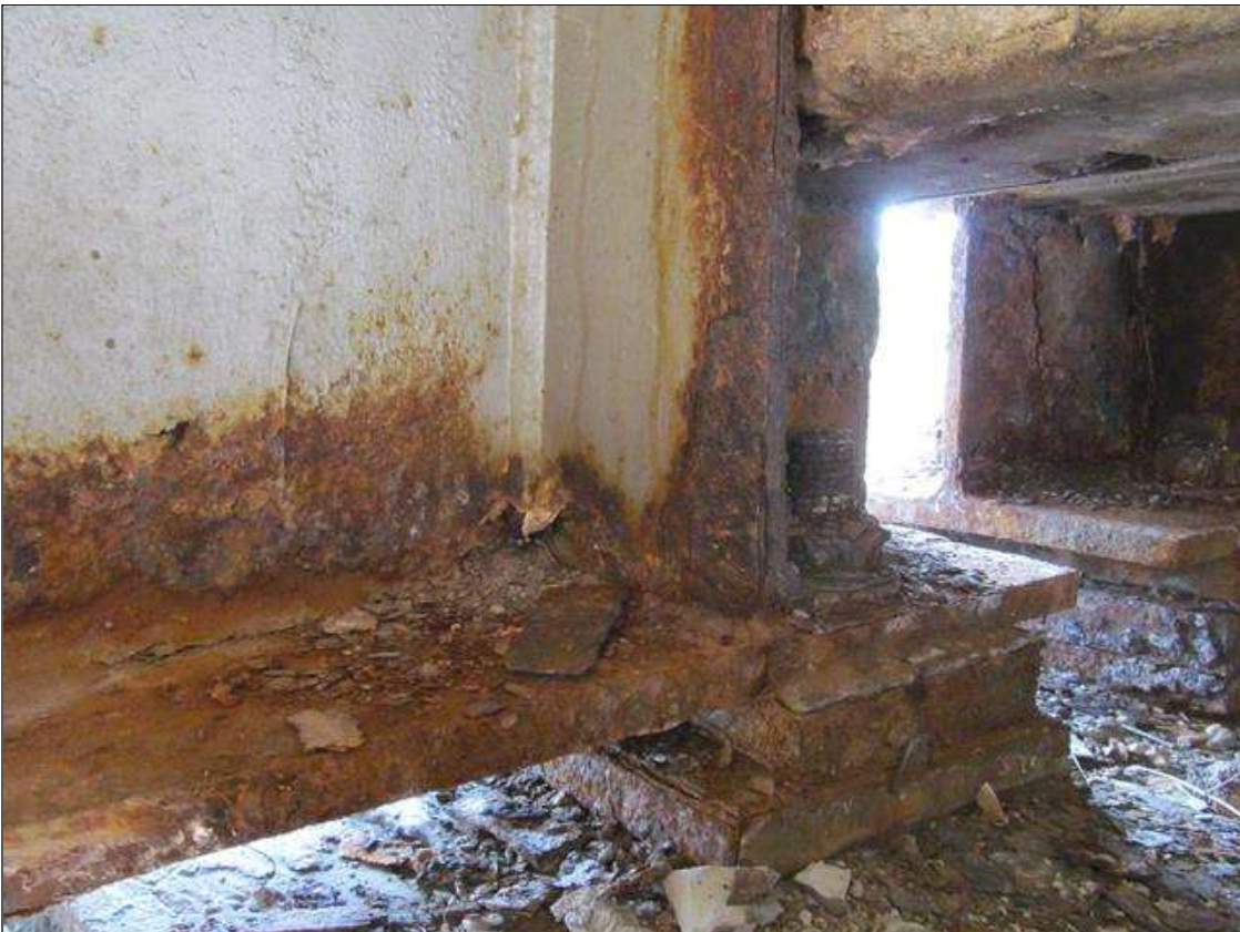
Span 3 Beam 8: BEAM END AT BENT 2 HAS SURFACE CORROSION WITH PITTING UP TO 1/16" AND LAYERED RUST FOR APPROX 2'L.
