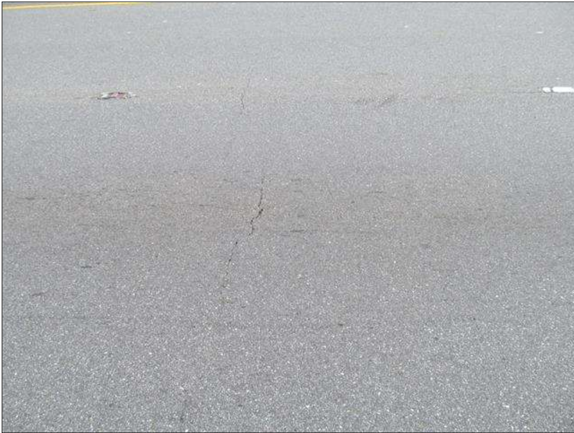
Span 2 Wearing Surface: SCATTERED MAP CRACKING UP TO 1/16"W
