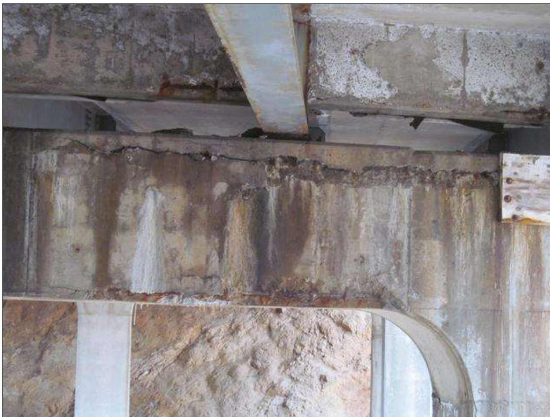
Bent 2 Cap 1: NORTH FACE, TOP 6" OF THE CAP AT BAYS 2-3, HORIZONTAL SPALLING, APPROX 10'L X 3"W X UP TO 2"D. THE AREA ABOVE HAS DELAMINATED.
