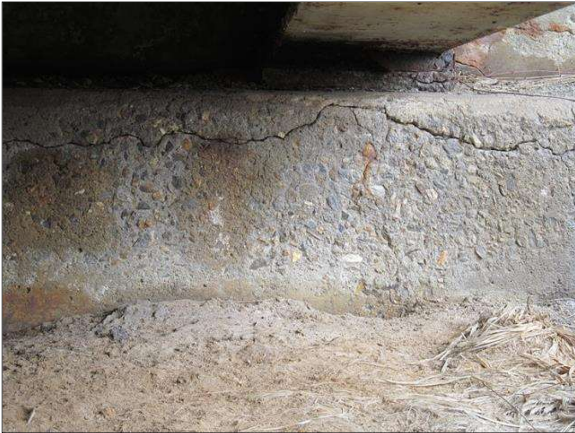
End Bent 2 Cap 1: RT END OF THE CAP FACE, HORIZONTAL CRACKING UP TO 1/8"W
