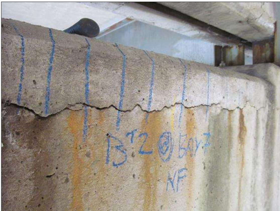
Bent 2 Cap 1: NORTH FACE, TOP 6" OF CAP, HORIZONTAL CRACKING UP TO 3/16"W IS SCATTERED ALONG THE LENGTH OF THE CAP. THE AREA ABOVE THE CRACKING IS DELAMINATED.
