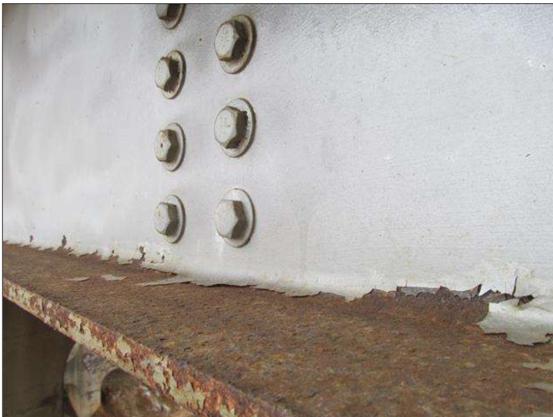
OUTBOARD BEAMS, SURFACE CORROSION ALONG THE LENGTH OF THE LOWER FLANGE IN AREAS OF PC FAILURE
