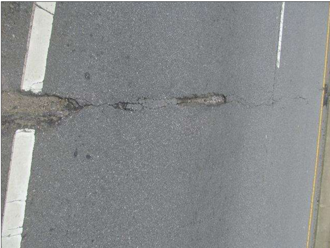
Span 2 Wearing Surface: AT BENT 2, SCATTERED SPALLING UP TO 2" D ALONG THE JOINT TOTALING APPROX 6 SQFT
