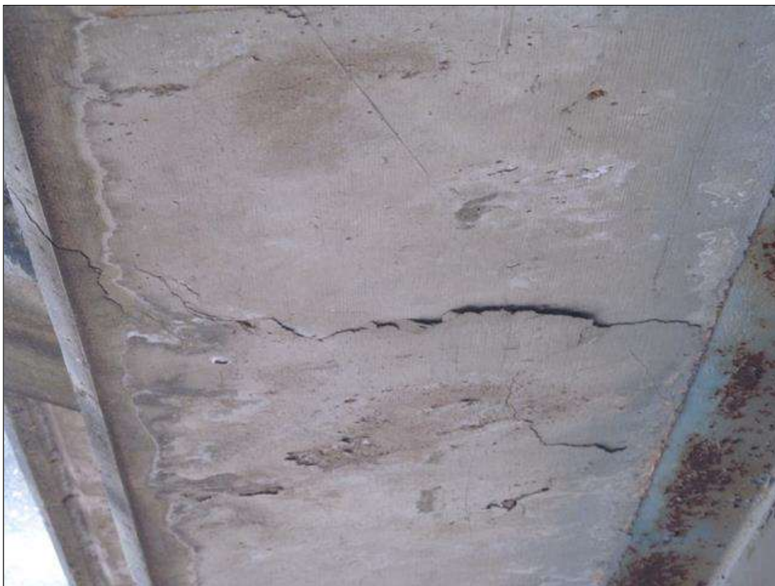
Span 1 Deck: UNDERSIDE OF THE DECK OVERHANGS, SCATTERED DELAM; TYP
