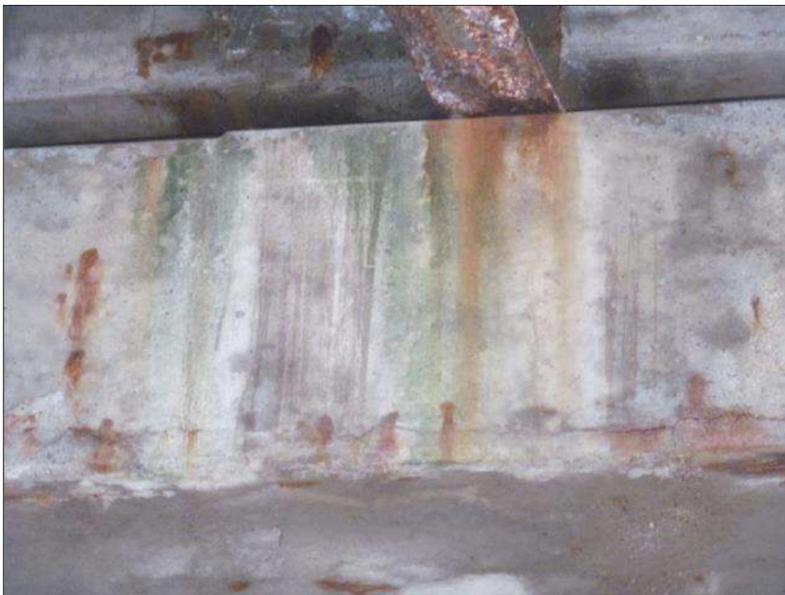
Bent 1 Cap 1: NORTH FACE, HORIZONTAL CRACKING UP TO 3/16"W WITH EFFLO AND RUST STAINING, SCATTERED.
