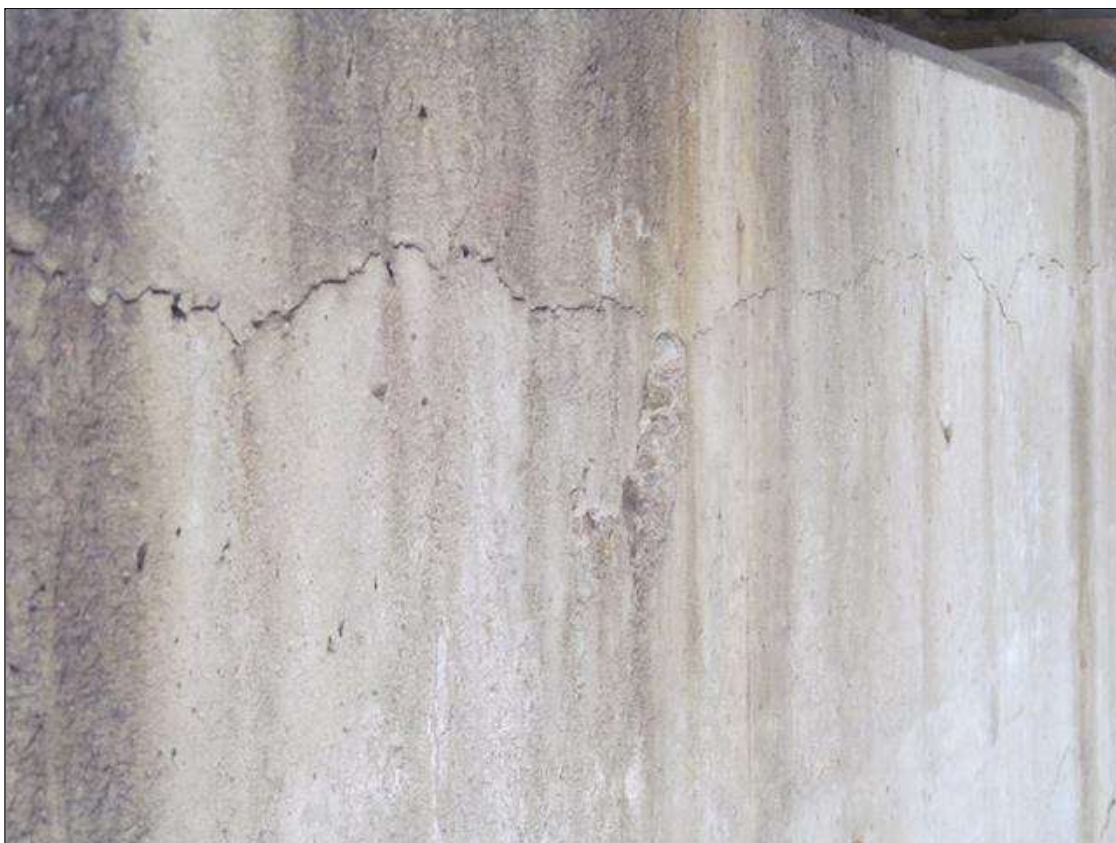
Bent 2 Cap 1: RT AND LT ENDS OF THE CAP, LOWER SIDES, HORIZONTAL AND MAP CRACKING UP TO 1/8"W WITH EFFLO BUILD-UP AND RUST STAINING.
