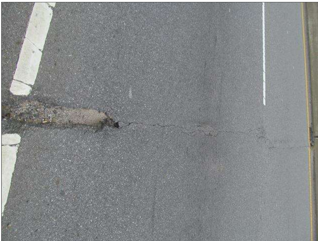
Span 1 Wearing Surface: AT BENT 1, SCATTERED SPALLING UP TO 2"D ALONG THE JOINT
