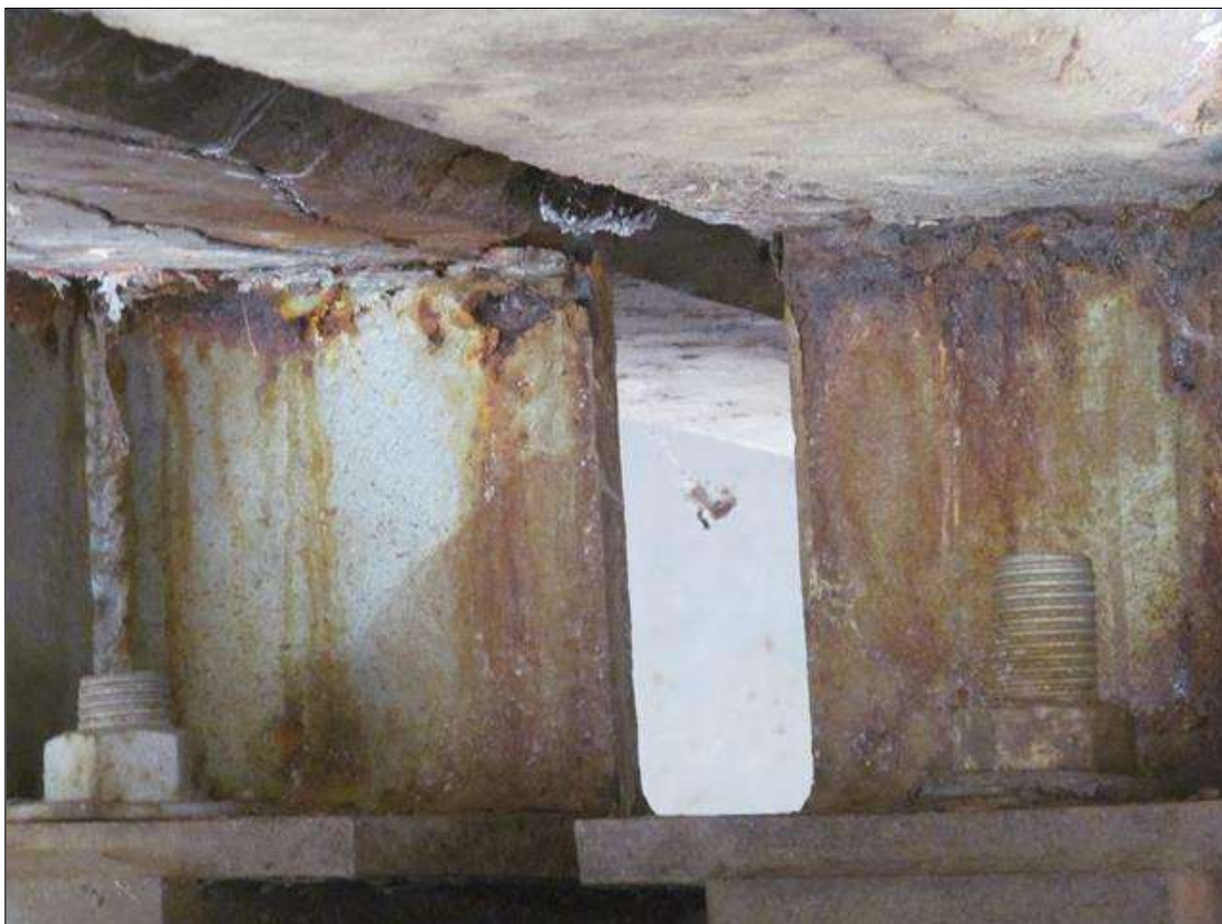
INBOARD BEAM ENDS AT BENT 2 HAVE SCATTERED SURFACE CORROSION
