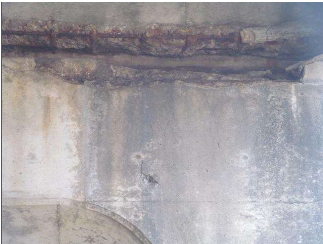
Bent 1 Cap 1: NORTH FACE AT BAY 1, TOP 4" OF THE CAP, HORIZONTAL SPALLING WITH EXPOSED RESTEEL, APPROX 4'LX 3"W X UP TO 3"D.
