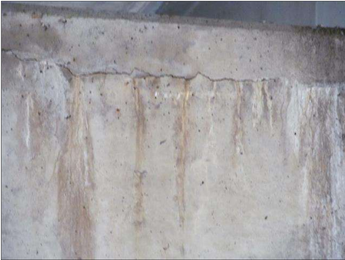
Bent 2 Cap 1: NORTH FACE, TOP 6" OF CAP, HORIZONTAL CRACKING UP TO 3/16"W IS SCATTERED ALONG THE LENGTH OF THE CAP. THE AREA ABOVE THE CRACKING IS DELAMINATED.
