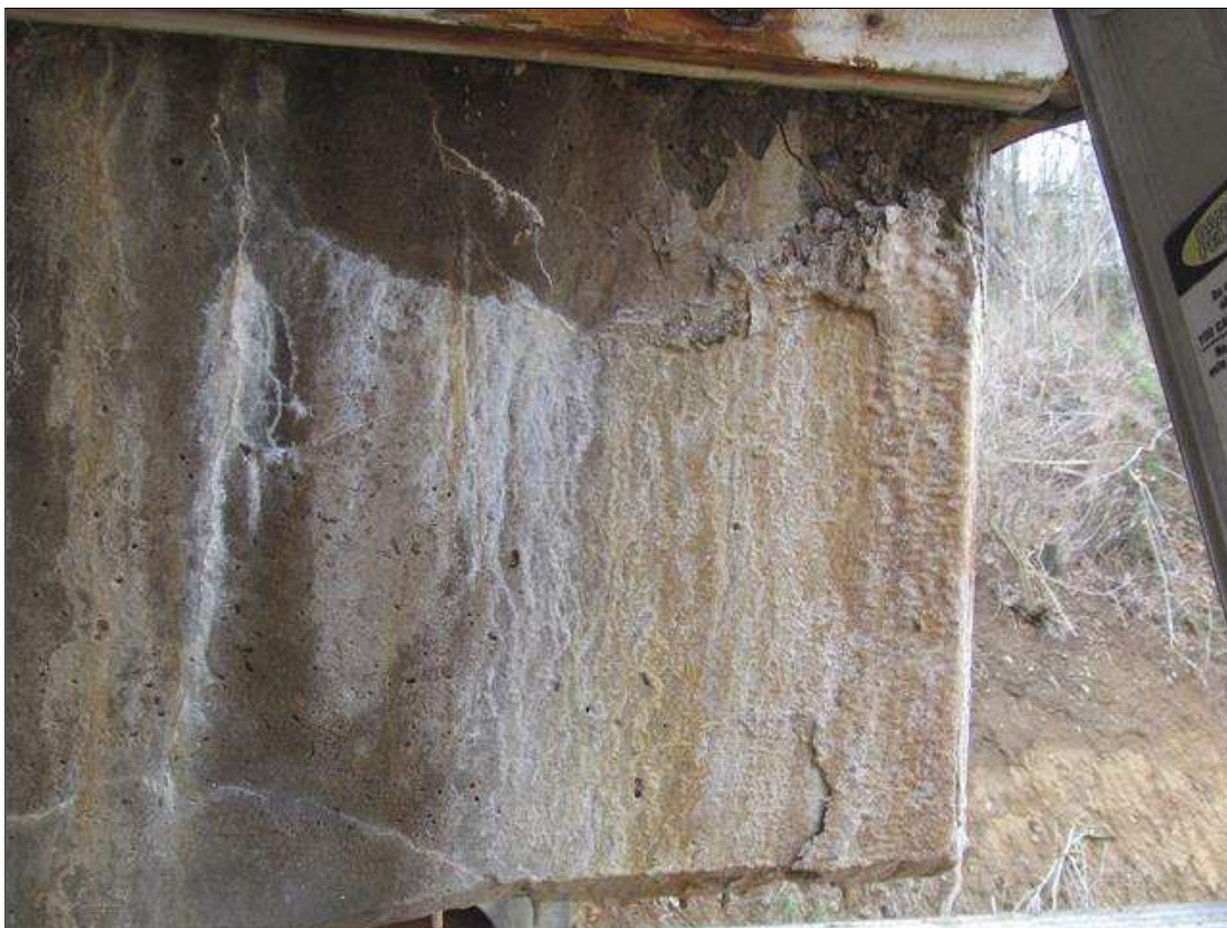
Bent 2 Cap 1: RT AND LT ENDS OF THE CAP, LOWER SIDES, HORIZONTAL AND MAP CRACKING UP TO 1/8"W WITH EFFLO BUILD-UP AND RUST STAINING.
