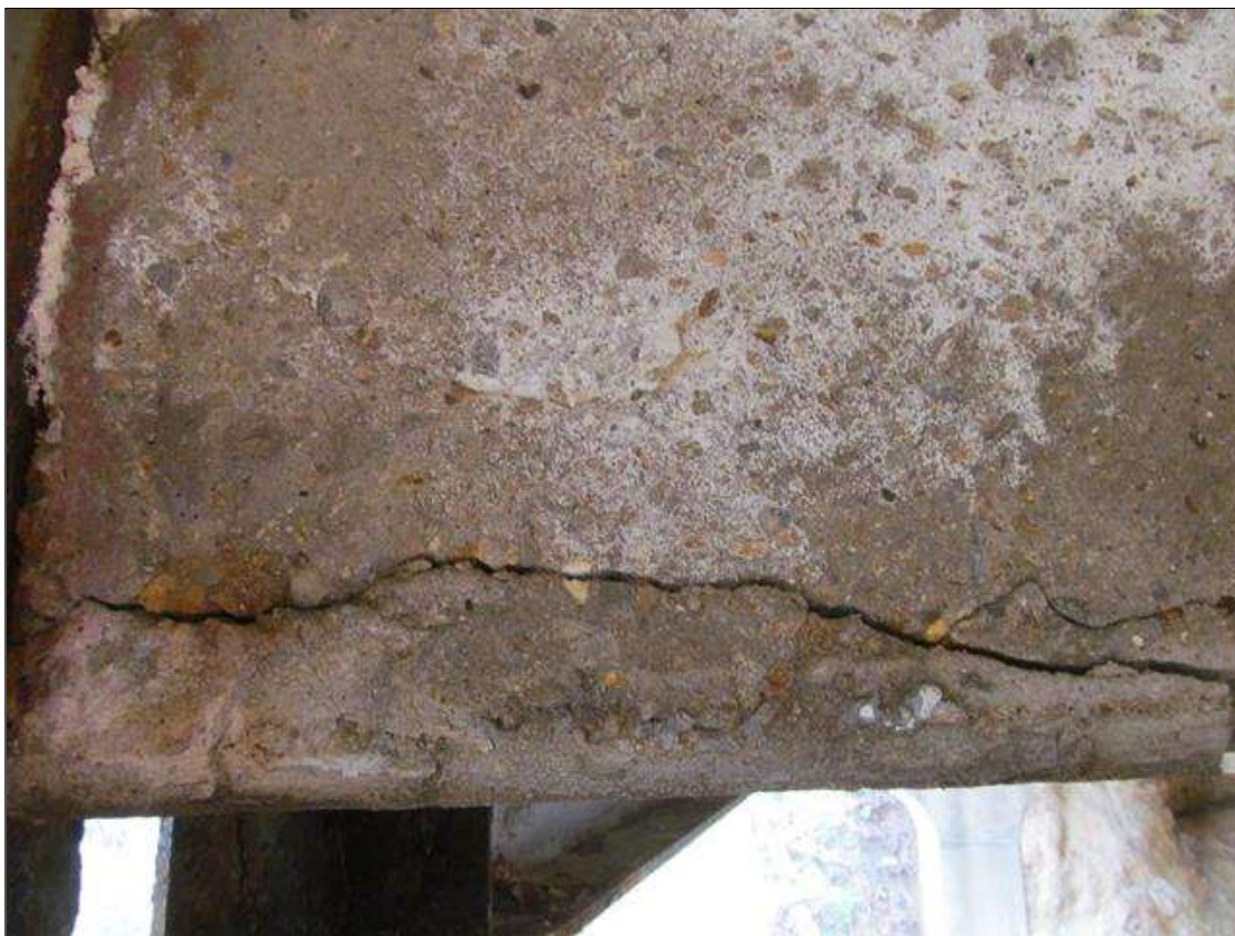
AT BENT 2, CONCRETE END DIAPHRAGMS ARE TYPICALLY CRACKED AND SPALLED EXPOSING RESTEEL. THE OUTBOARD ENDS HAVE DISINTEGRATED EXPOSING THE RESTEEL FULLY (INBOARD VIEW OF CRACKING).
