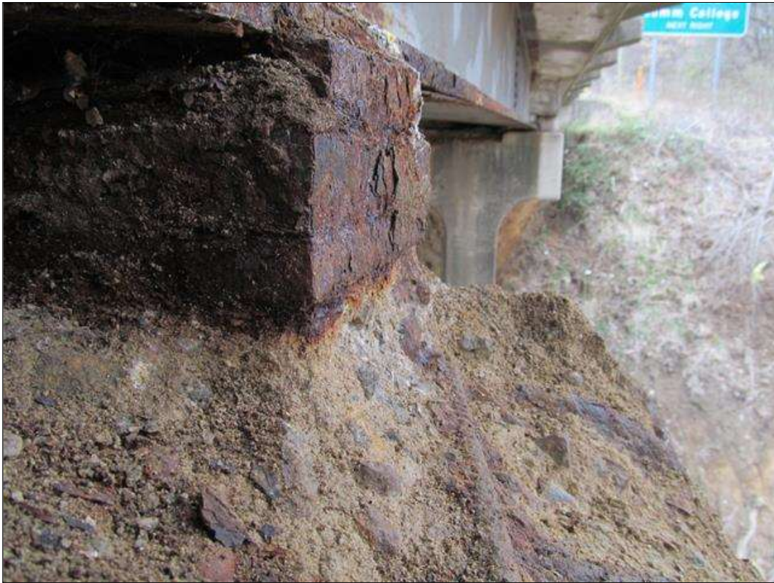
Bent 2 Cap 1: LT END OF THE CAP, PATCHED AREA (FORMERLY SPALLED) HAS FAILED EXPOSING THE RESTEEL. THE RESTEEL HAS PITTING UP TO 1/32". THE SPALLED AREA HAS UNDERMINED APPROX 3SQIN OF THE BEARING AREA OF SPAN 2, BEAM 1. THE SPALLED AREA HAS REACHED THE BEARING AREA OF SPAN 3, BEAM 1, BUT HAS NOT YET UNDERMINED IT. PMAINT.
