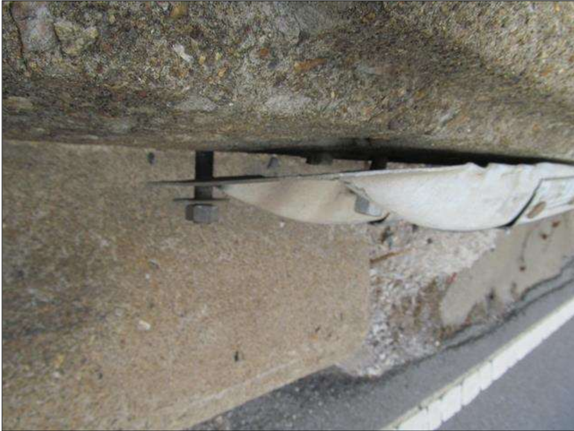
NW CORNER, GR CONNECTION BOLTS (FROM GTO STRUCTURE) ARE MISSING/LOOSE
