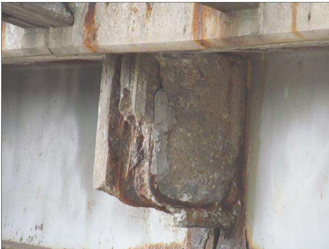
AT BENT 2, CONCRETE END DIAPHRAGMS ARE TYPICALLY CRACKED AND SPALLED EXPOSING RESTEEL. THE OUTBOARD ENDS HAVE DISINTEGRATED EXPOSING THE RESTEEL FULLY.
