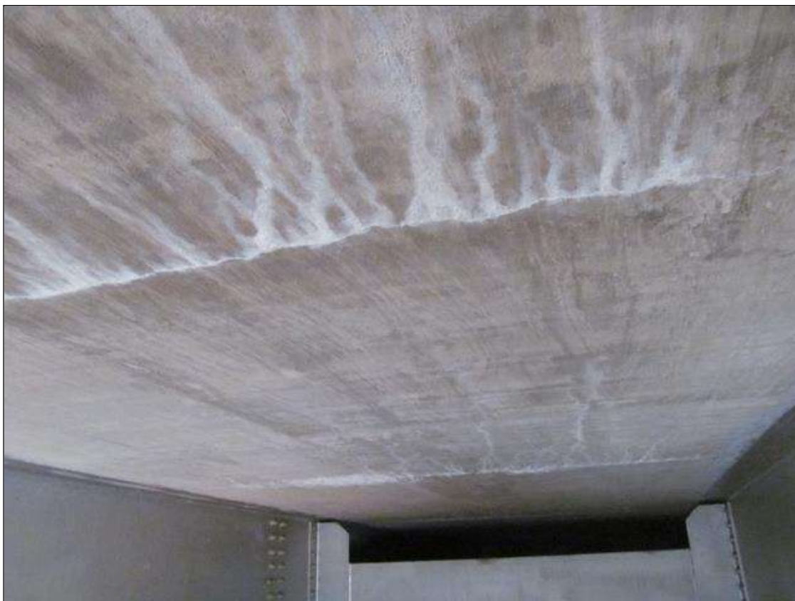
Span 1 Deck: UNDERSIDE OF THE DECK, HL TRANSVERSE CRACKING WITH EFFLO STAINING, SCATTERED; TYP
