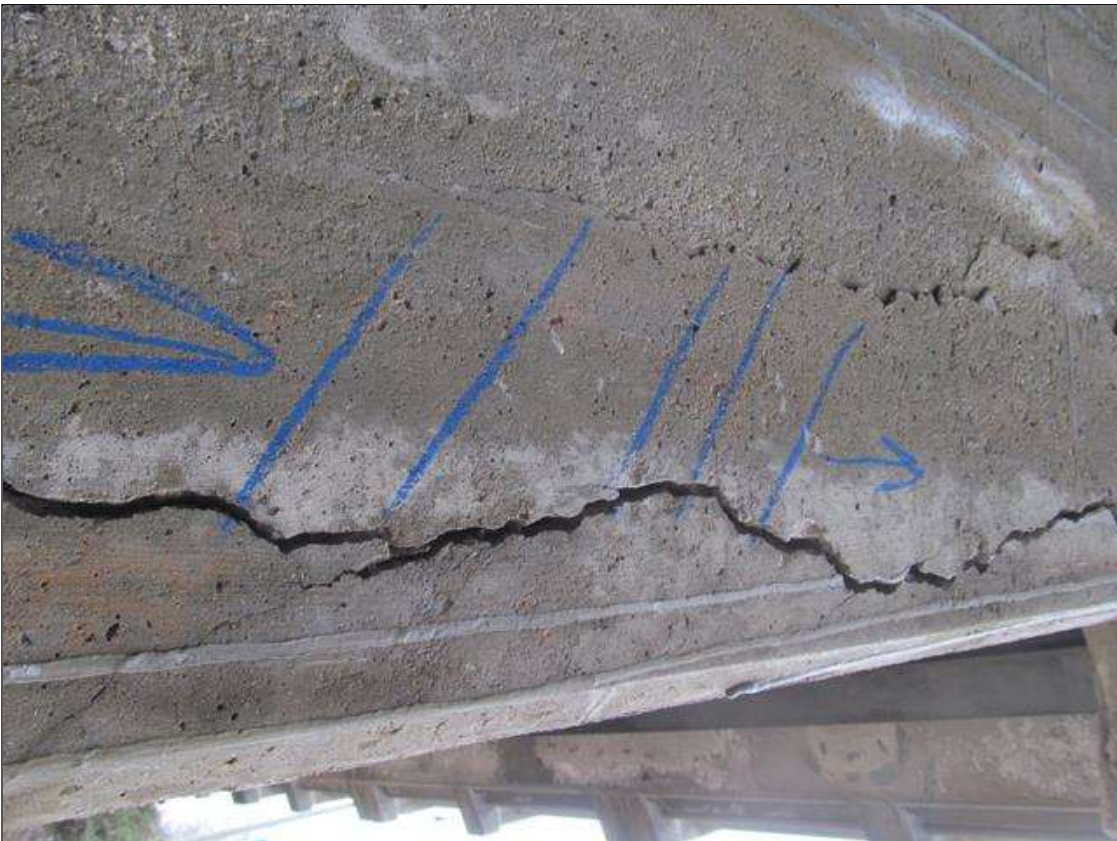
Bent 2 Pile 1: COLUMN CORNERS, VERTICAL CRACKING UP TO 3/8"W RUNS APPROX 3/4 OF THE HEIGHT. APPROX 5SQFT OF DELAM IS ADJACENT TO THE CRACKING.
