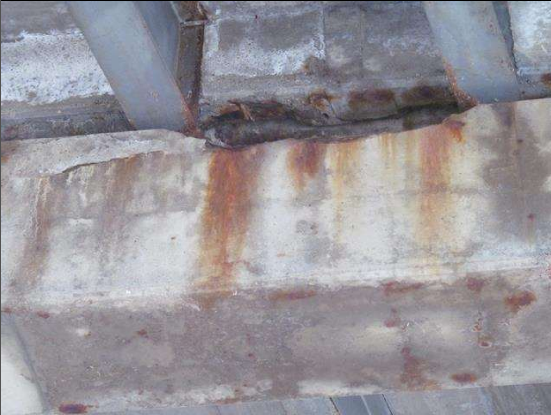
Bent 2 Cap 1: SOUTH FACE, TOP OF THE CAP AT BEAMS 4-5, HORIZONTAL SPALLING, APPROX 5'L X 3"W X UP TO 4"D EXPOSING THE RESTEEL.
