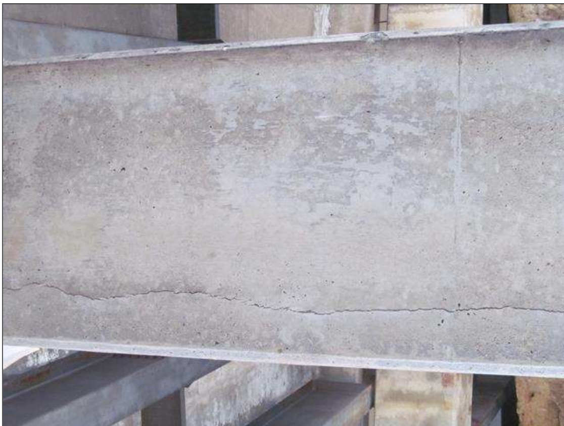
Bent 2 Pile 2: AT THE CORNERS, VERTICAL CRACKING UP TO 1/8"W, SCATTERED ALONG THE HEIGHT.
