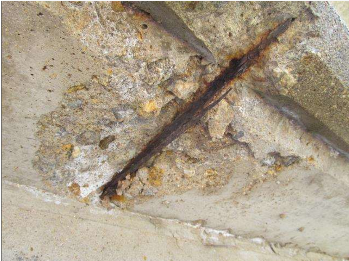
Span 1 Deck: LT DECK OVERHANG, APPROX 1SQFT SPALL WITH EXPOSED RESTEEL, UP TO 1"D.
