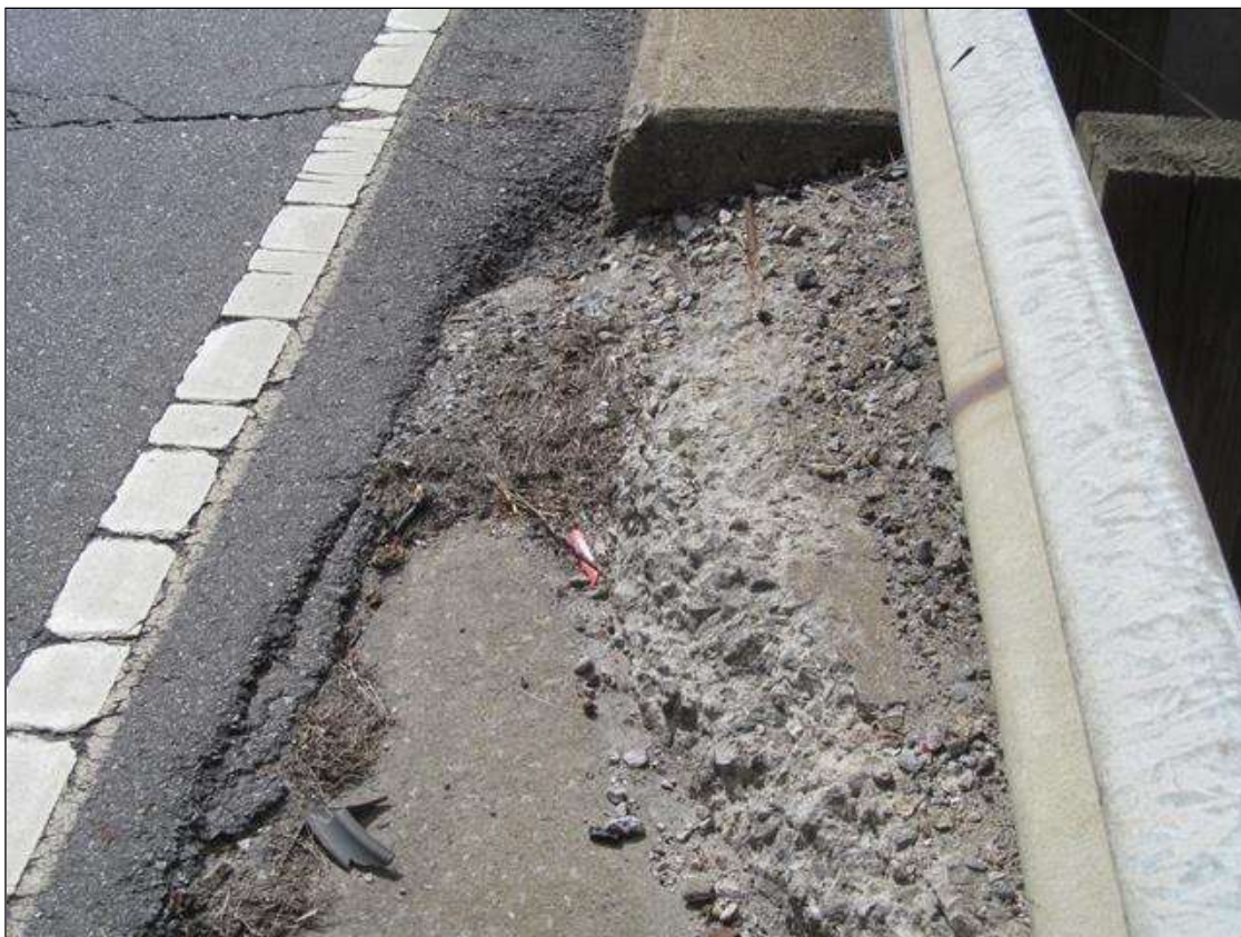
NW CORNER, CONCRETE CURBING HAS DISINTEGRATED EXPOSING RESTEEL FOR APPROX 3'L.
