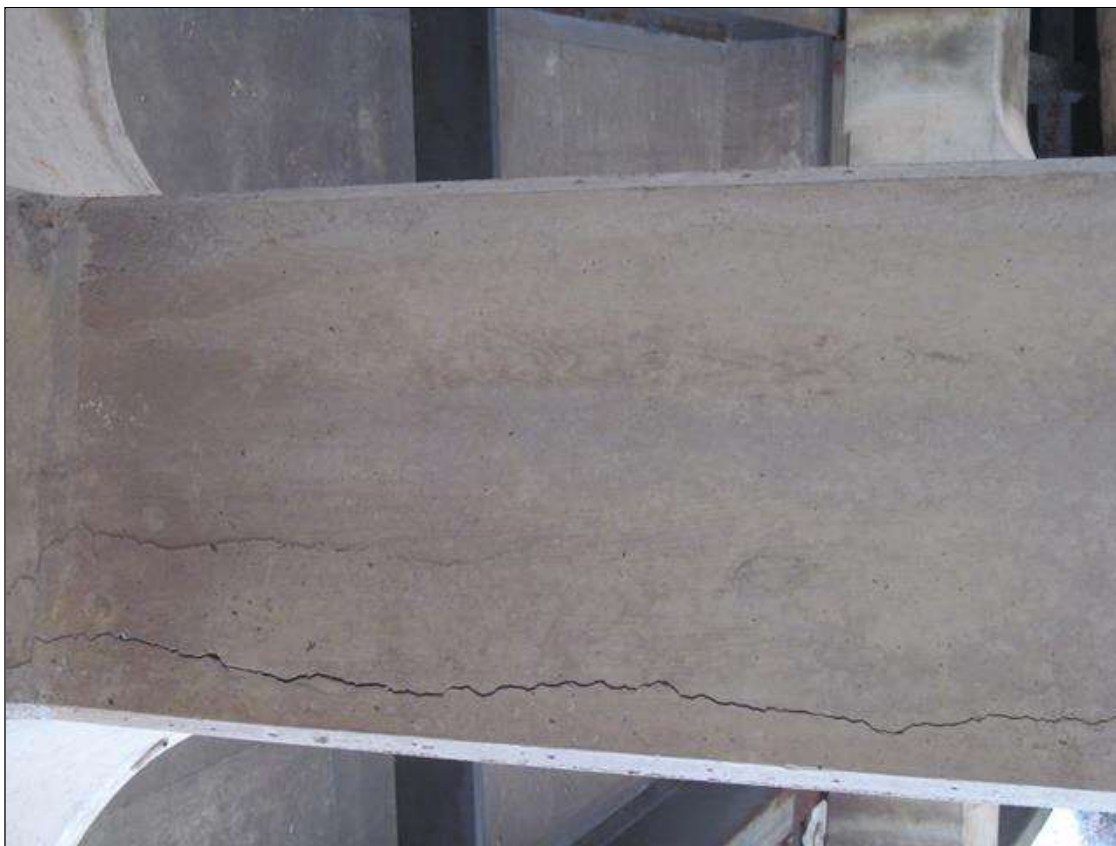
Bent 2 Pile 3: AT THE CORNERS, VERTICAL CRACKING UP TO 1/8"W, SCATTERED ALONG THE HEIGHT.
