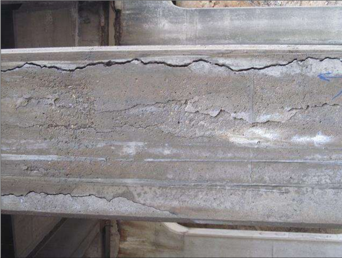
Bent 2 Pile 1: COLUMN CORNERS, VERTICAL CRACKING UP TO 3/8"W RUNS APPROX 3/4 OF THE HEIGHT. APPROX 5SQFT OF DELAM IS ADJACENT TO THE CRACKING.
