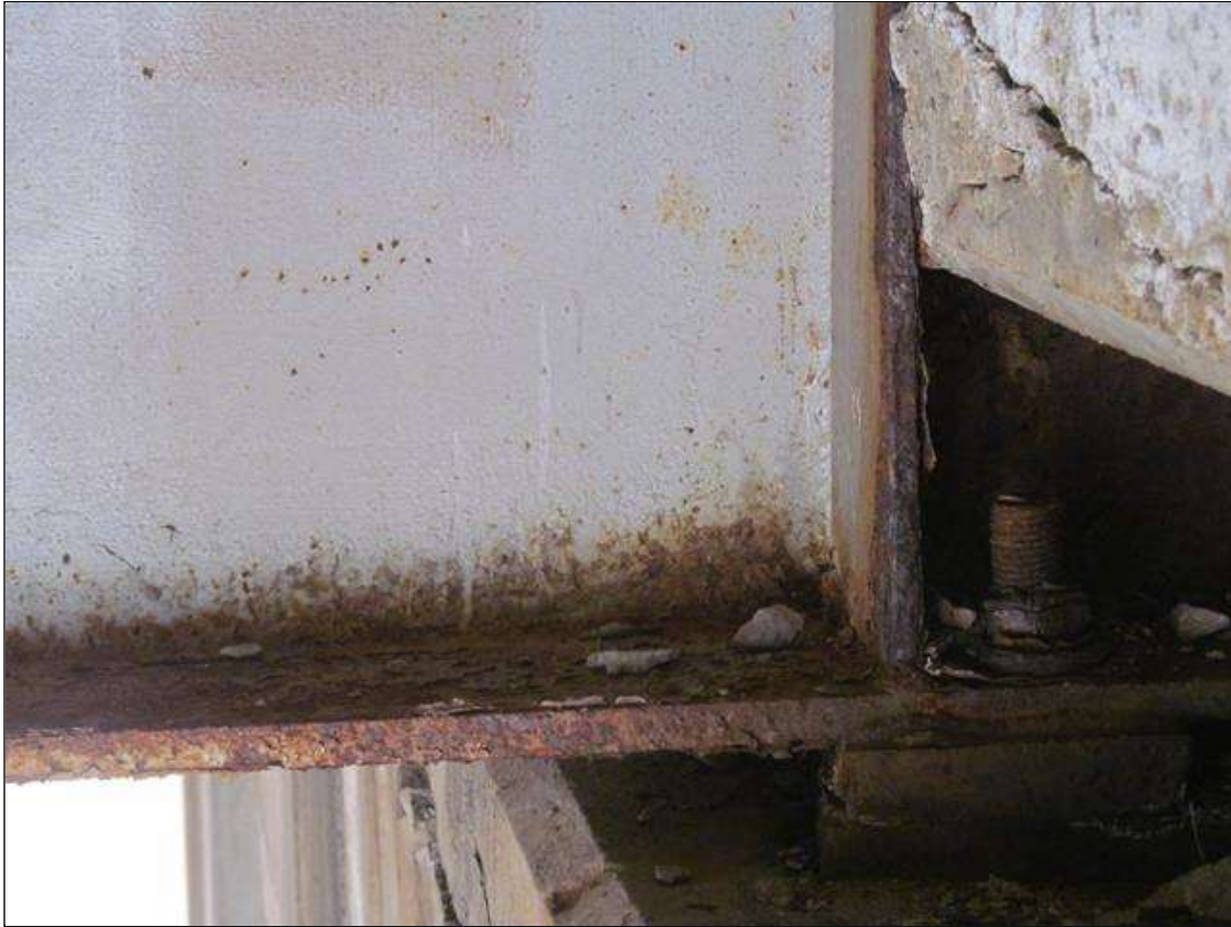
Bent 2 Cap 1: LT END OF THE CAP, PATCHED AREA (FORMERLY SPALLED) HAS FAILED EXPOSING THE RESTEEL. THE RESTEEL HAS PITTING UP TO 1/32". THE SPALLED AREA HAS UNDERMINED APPROX 3SQIN OF THE BEARING AREA OF SPAN 2, BEAM 1. THE SPALLED AREA HAS REACHED THE BEARING AREA OF SPAN 3, BEAM 1, BUT HAS NOT YET UNDERMINED IT. PMAINT.
