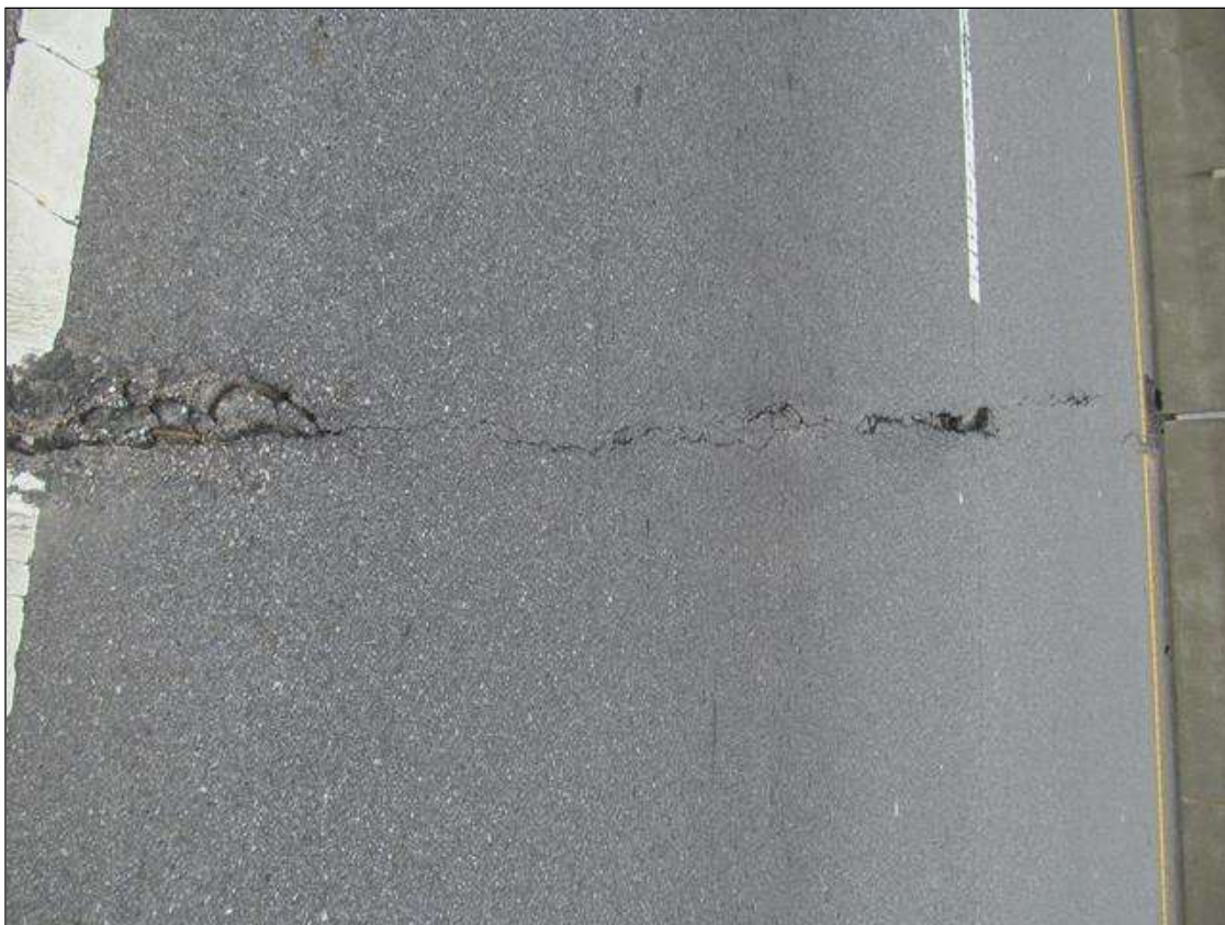
Span 2 Wearing Surface: AT BENT 2, SCATTERED SPALLING UP TO 2"D ALONG THE JOINT TOTALING APPROX 3SQFT
