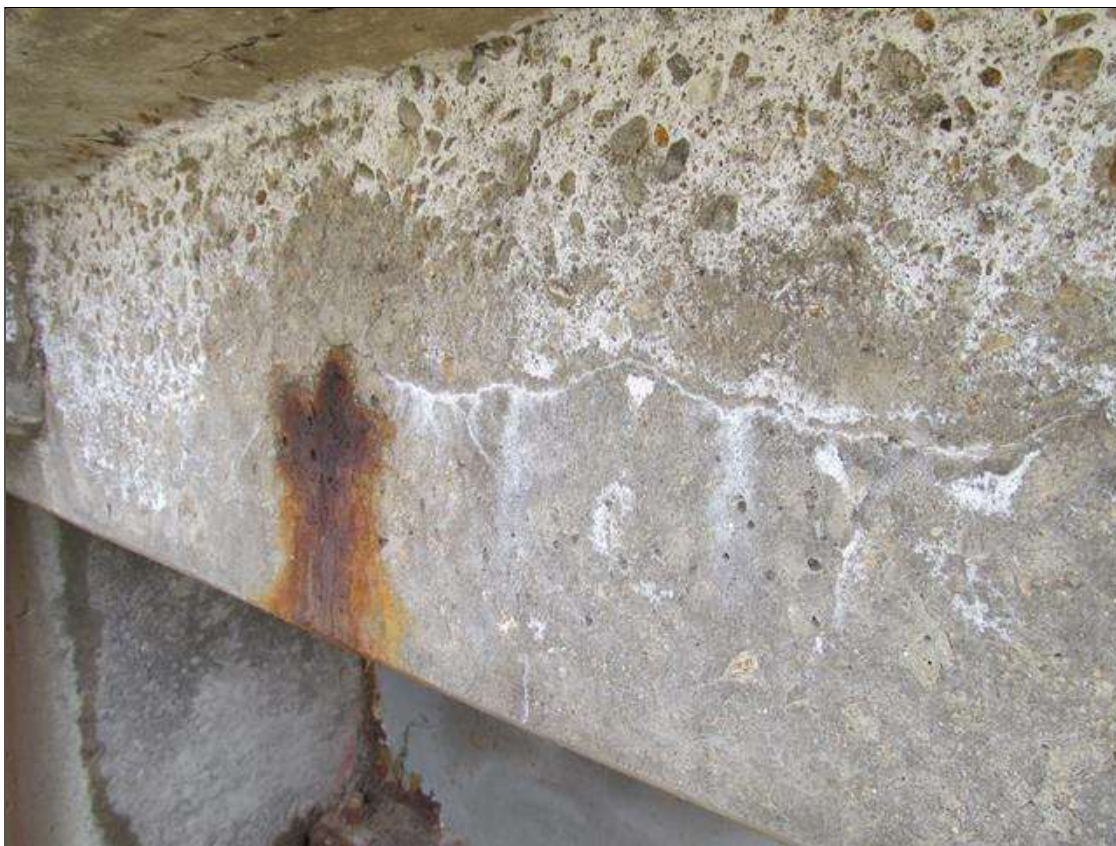
Span 1 Deck: RT & LT ENDS, HORIZONTAL HL CRACKING WITH RUST STAINING, SCATTERED
