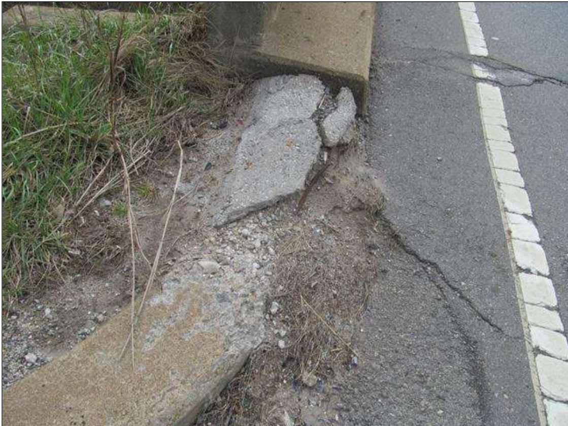
NE CORNER, CONCRETE CURBING HAS BEEN DAMAGED AND BROKEN EXPOSING RESTEEL FOR APPROX 2'L.
