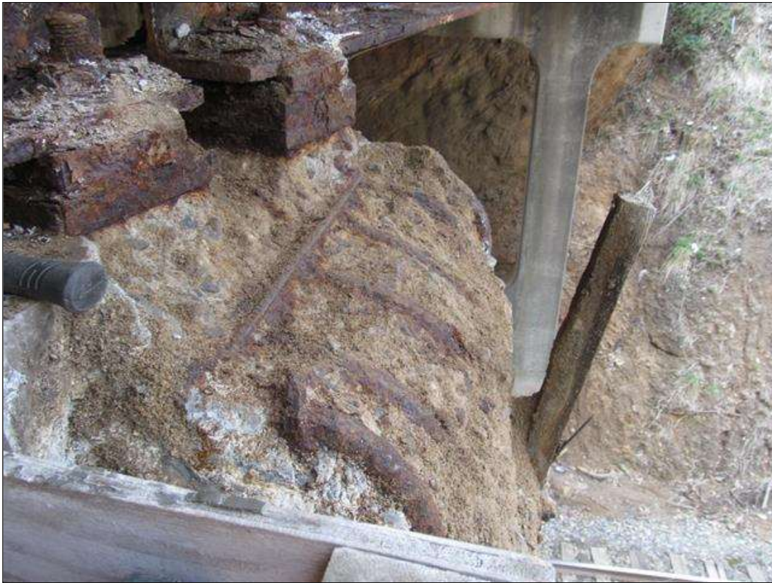
Bent 2 Cap 1: LT END OF THE CAP, PATCHED AREA (FORMERLY SPALLED) HAS FAILED EXPOSING THE RESTEEL. THE RESTEEL HAS PITTING UP TO 1/32". THE SPALLED AREA HAS UNDERMINED APPROX 3SQIN OF THE BEARING AREA OF SPAN 2, BEAM 1. THE SPALLED AREA HAS REACHED THE BEARING AREA OF SPAN 3, BEAM 1, BUT HAS NOT YET UNDERMINED IT. PMAINT.
